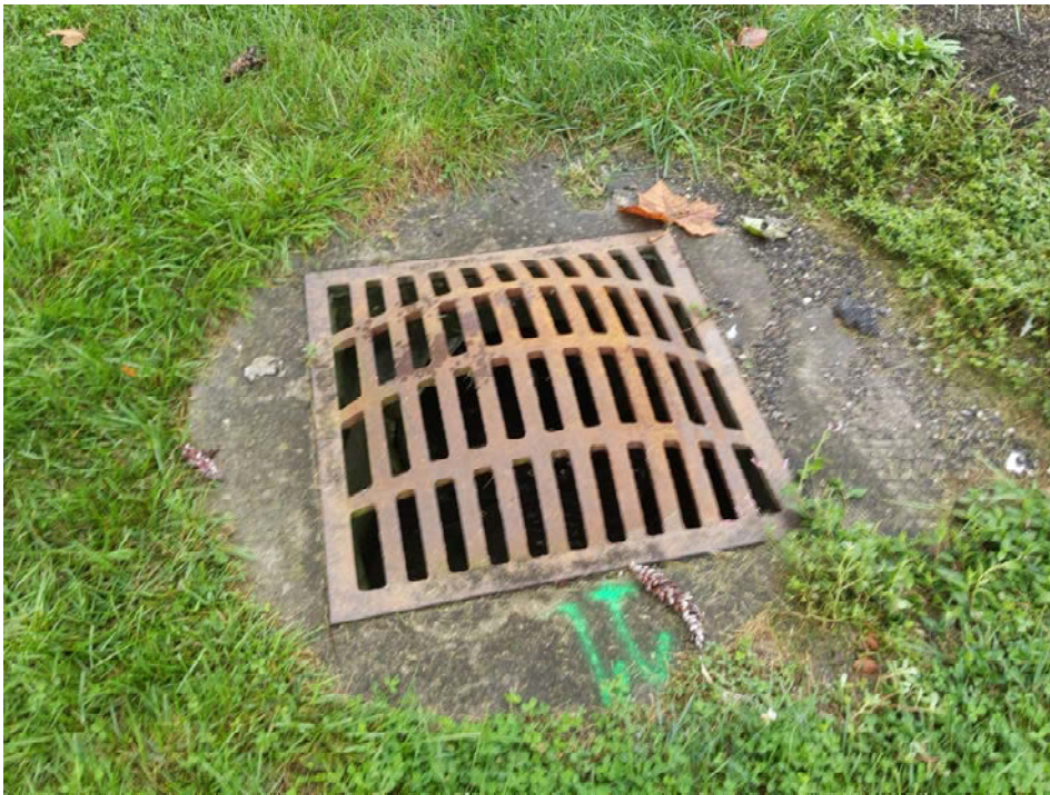
13. Looking west to drainage grate within existing right-of-way. Drainage in the investigated area is captured in open channels as well as a network of enclosed systems.
