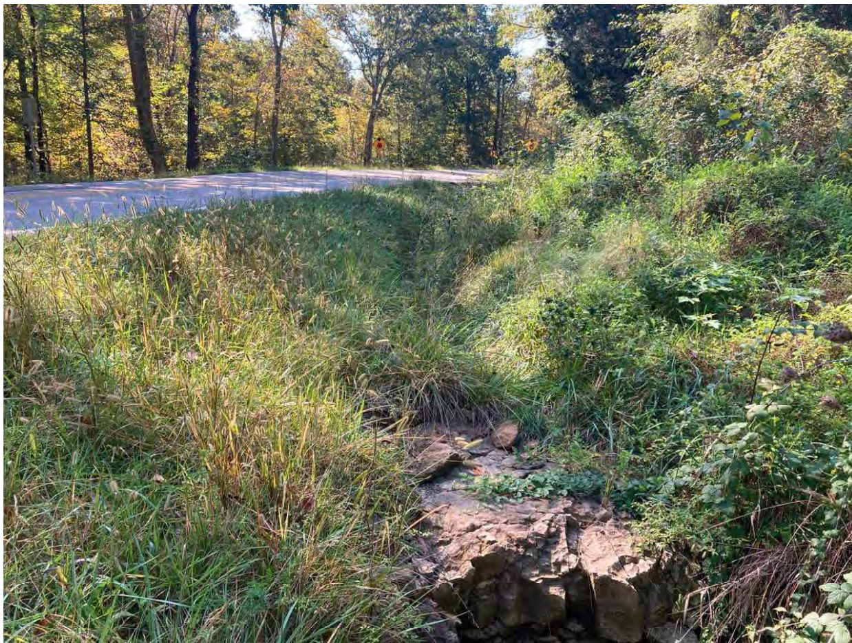
5 – View of RSD1 facing south; bedrock exposed in portions of the ditch
