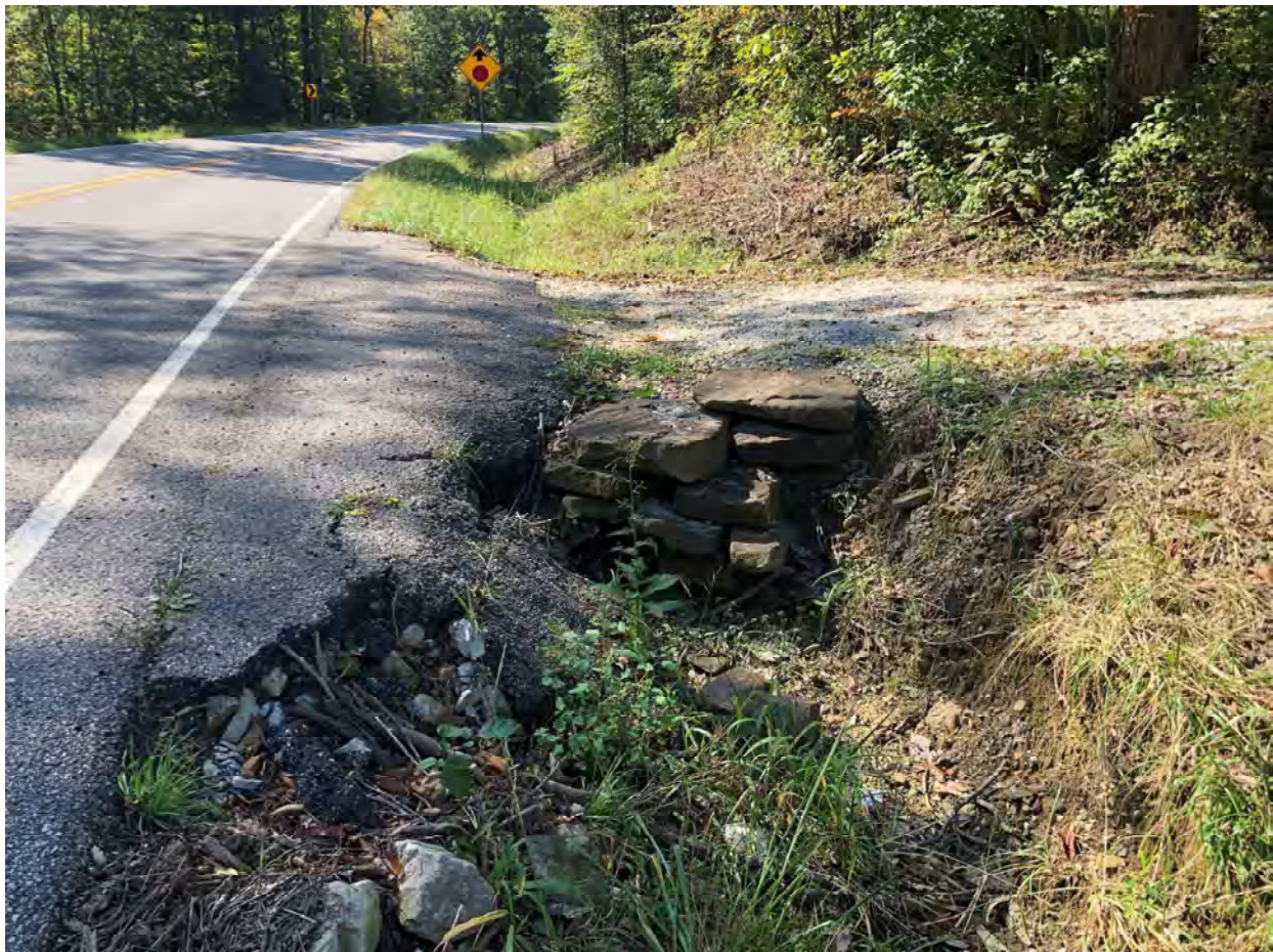
8 – View of private driveway over RSD1 facing southwest; a 12 inch diameter pipe conveys water beneath the driveway
