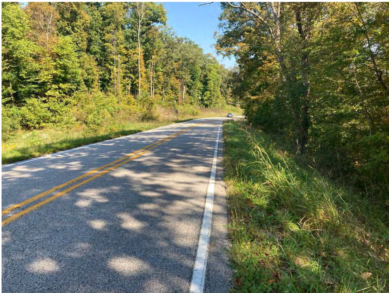
3 – View of SR 237 road embankment facing northeast; note steep slope east of road
