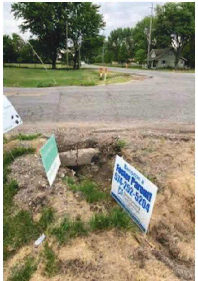
12- Facing North from Southwest Quadrant, Failing Drain under CR 18
