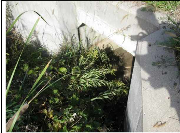
13. Looking northeast at culvert inlet under SR 39 on north side of I-70.
