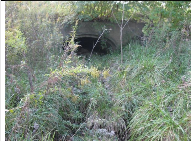
19. Looking southwest at UNT 1 and culvert outlet from east side of SR 39.
