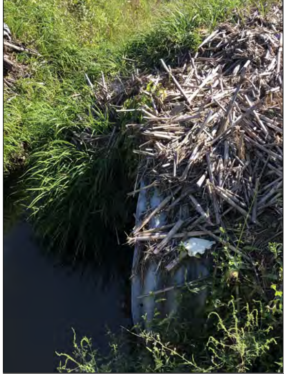
Picture 8—UNT to Lick Creek project structure northeast view; 9 SEP 2021. Note extensive drift deposits (corn stalks) from flooding.
