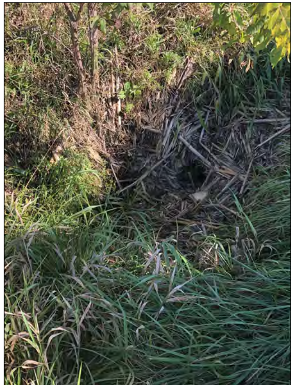
Picture 28—Northwest quadrant edge of Wetland 2 and pipe under overgrown farm entrance; north view; 9 SEP 2021.
