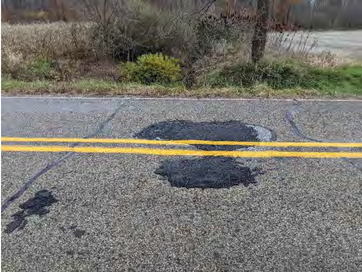
Photo 7: Wearing surface condition over small structure
