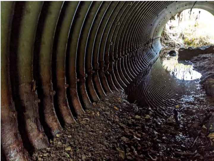
Photo 4: Rusting throughout the entire pipe.
