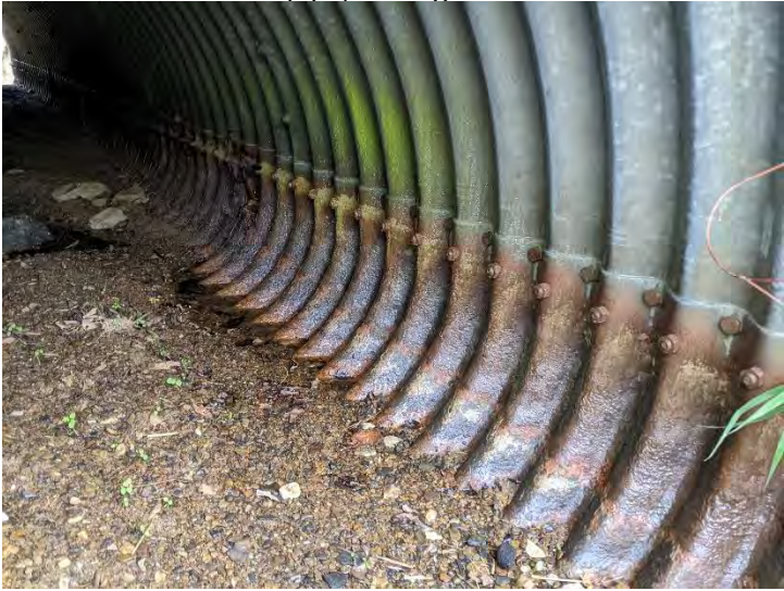
Photo 3: Condition of pipe, rusting and water line
