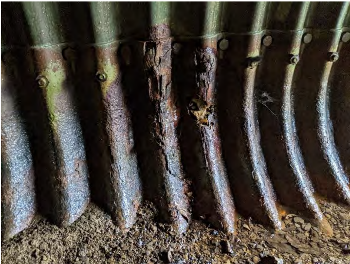
Photo 6: Pipe rusting out along the water line.
