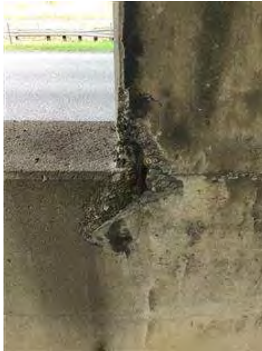
PHOTO 11 Condition Description Spall West Side Bent #2 Center Column
