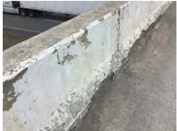
File Description Damage to North Barrier Rail Mid Span File Type Category Condition
