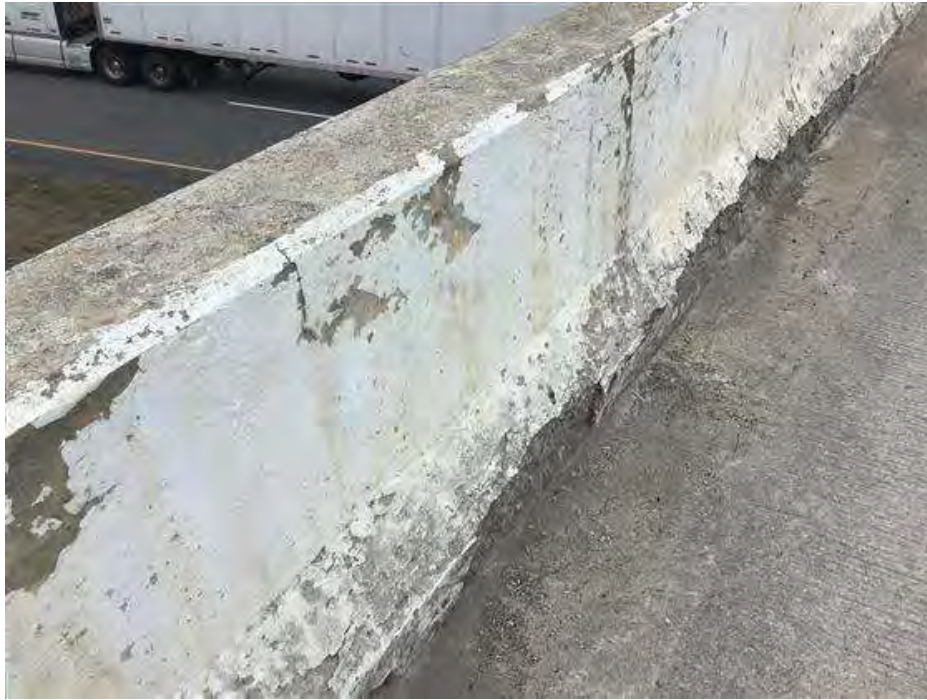
PHOTO 3 Condition Description Damage to North Barrier Rail Mid Span
