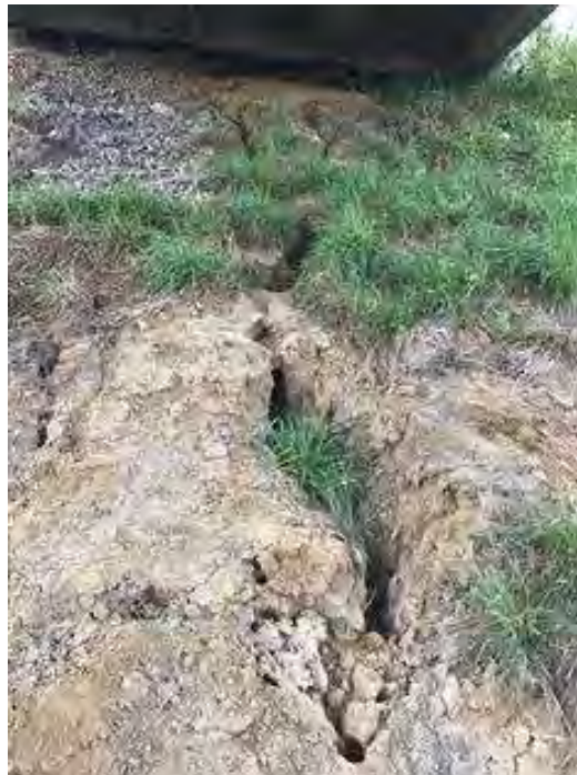
PHOTO 22 Other, Maintenance - Bridge Description Erosion under Span D facing North
