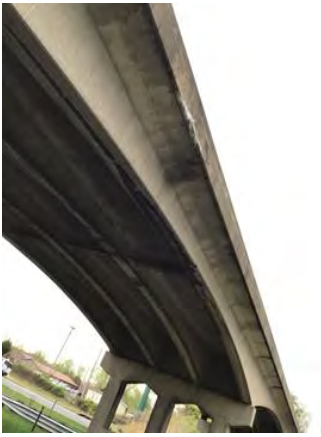
File Description Span B south coping and beam. File Type Category Condition
