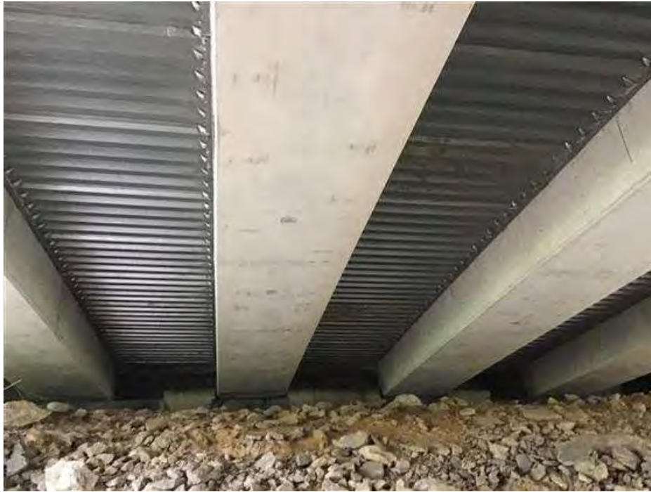
PHOTO 7 Condition Description Span A facing south.
