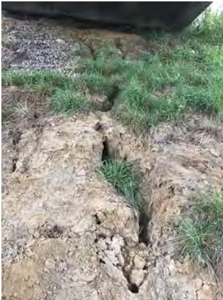
File Description Erosion under Span D facing North
