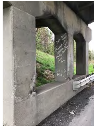
File Description Pier 2 east side. File Type Category Condition
