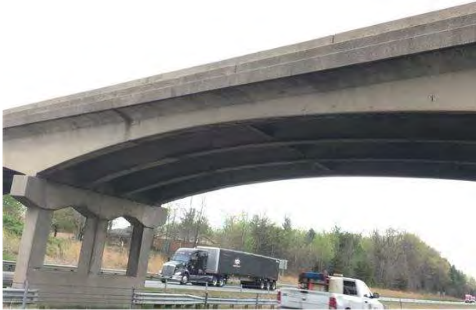
PHOTO 17 Condition Description Minor Spalls and Cracks in Beam #1 Span C
