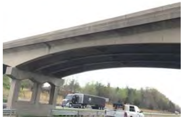
File Description Minor Spalls and Cracks in Beam #1 Span C
