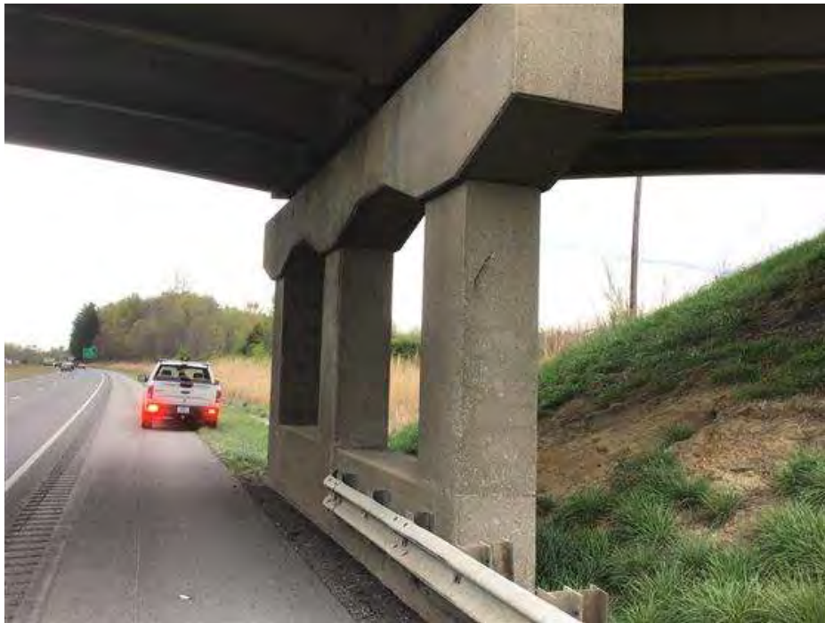
PHOTO 18 Condition Description Bent #4 facing Northeast
