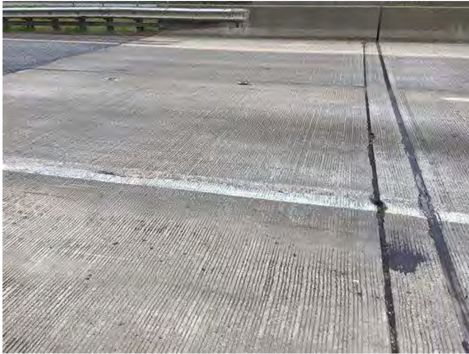
PHOTO 5 Condition Description North joint and approach slab.
