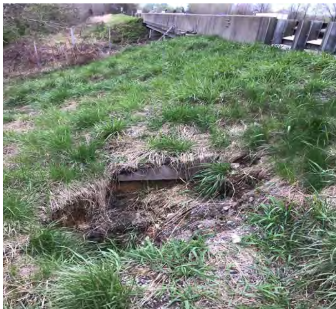
PHOTO 1 Description Sinkhole on northeast shoulder just past north approach.
