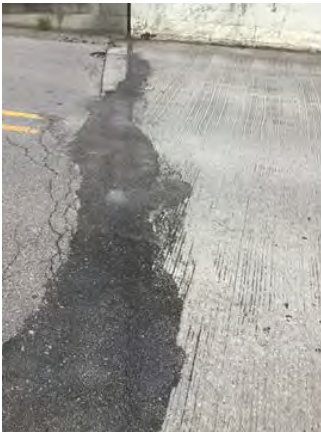
File Description East Joint facing South File Type Category Condition, Maintenance - Bridge
