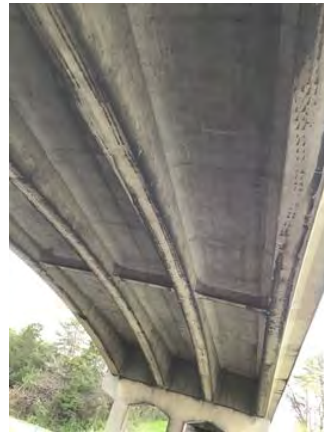
File Description Span C facing west. File Type Category Condition
