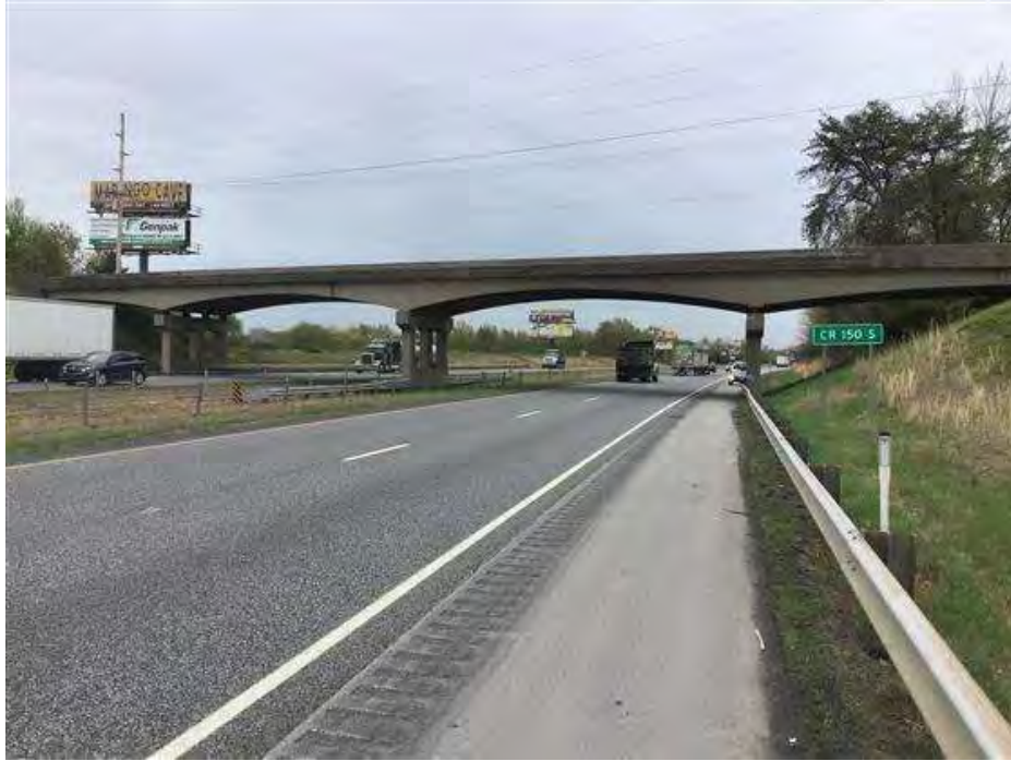
PHOTO 7 Elevation, Condition Description Side facing South
