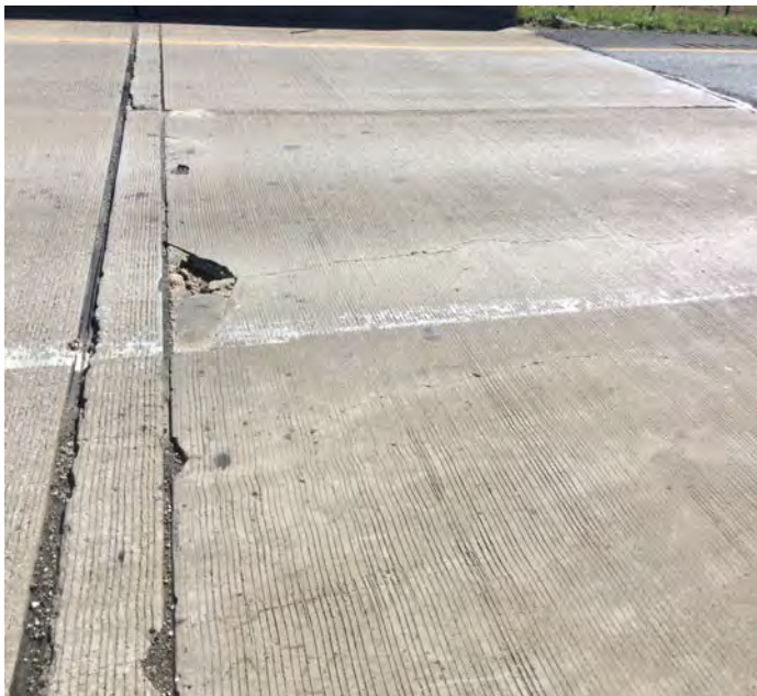
PHOTO 1 Description South joint and approach slab.
