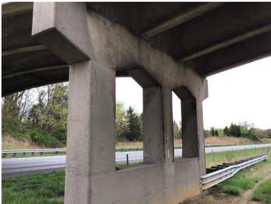
PHOTO 14 Condition Description Pier 3 east side.
