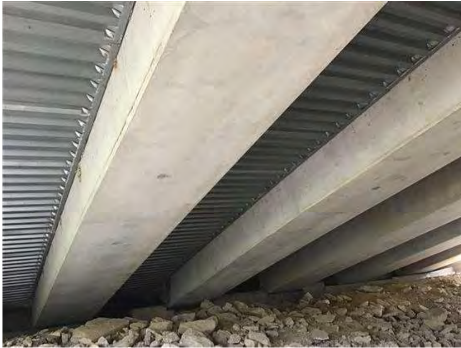
PHOTO 7 Condition Description Span A facing south.
