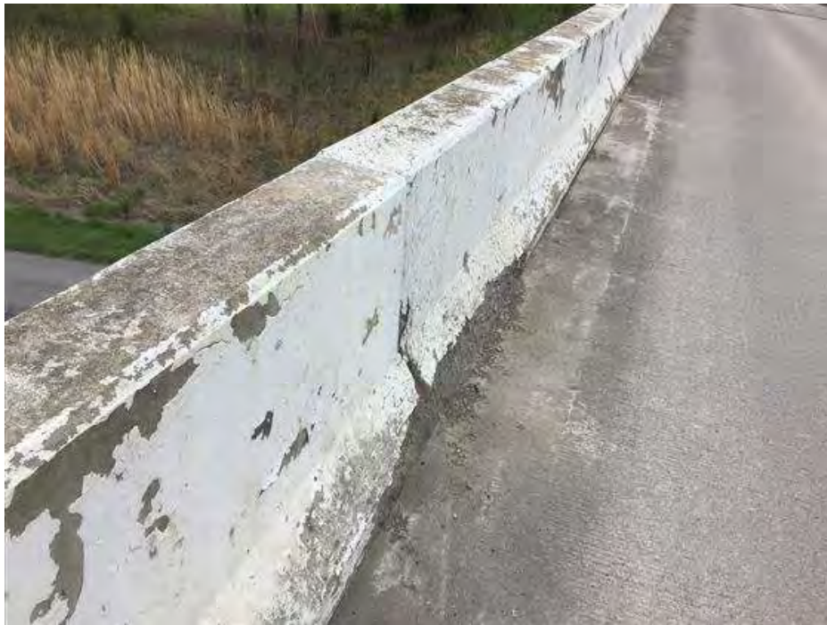
PHOTO 4 Condition Description Damage to North Barrier Rail over Span C facing East
