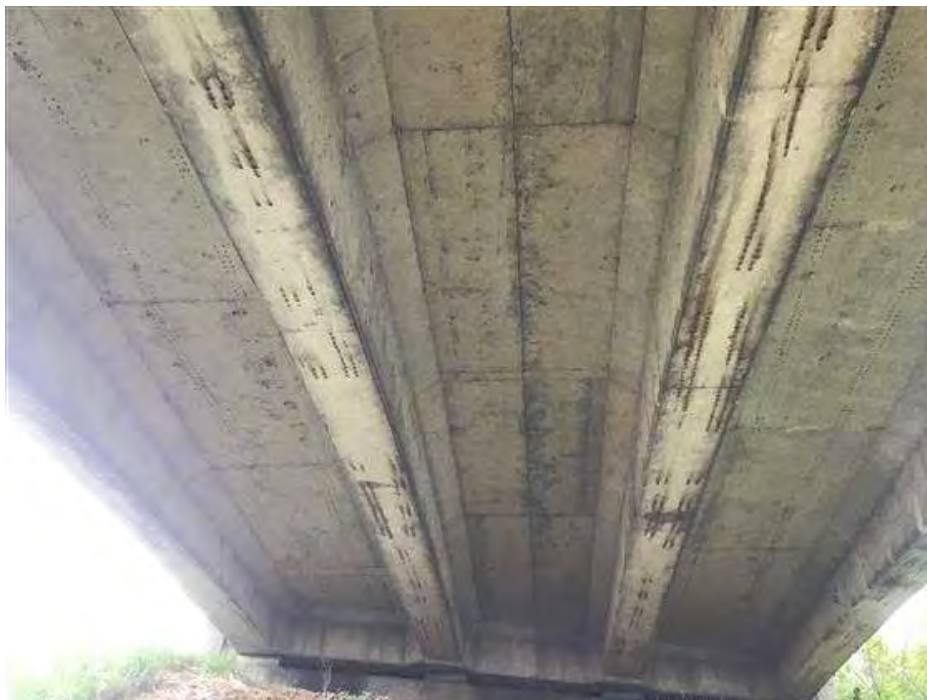
PHOTO 20 Condition Description Underside Span D facing East
