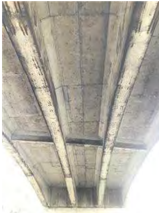
PHOTO 16 Condition Description Underside Span C facing West
