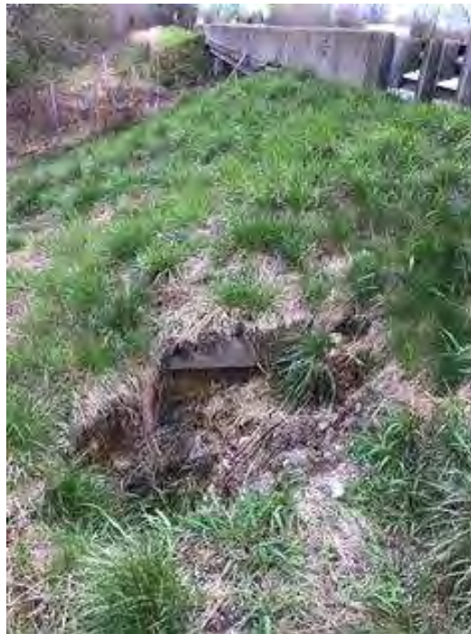
PHOTO 18 Condition, Other, Maintenance - Bridge Description Sinkhole on northeast shoulder just past north approach.
