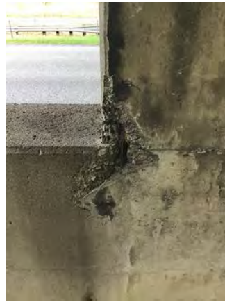
File Description Spall West Side Bent #2 Center Column
