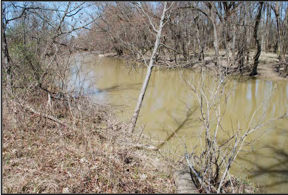
Figure 3. View of erosion along the south bank of the Wabash River, facing northwest.
