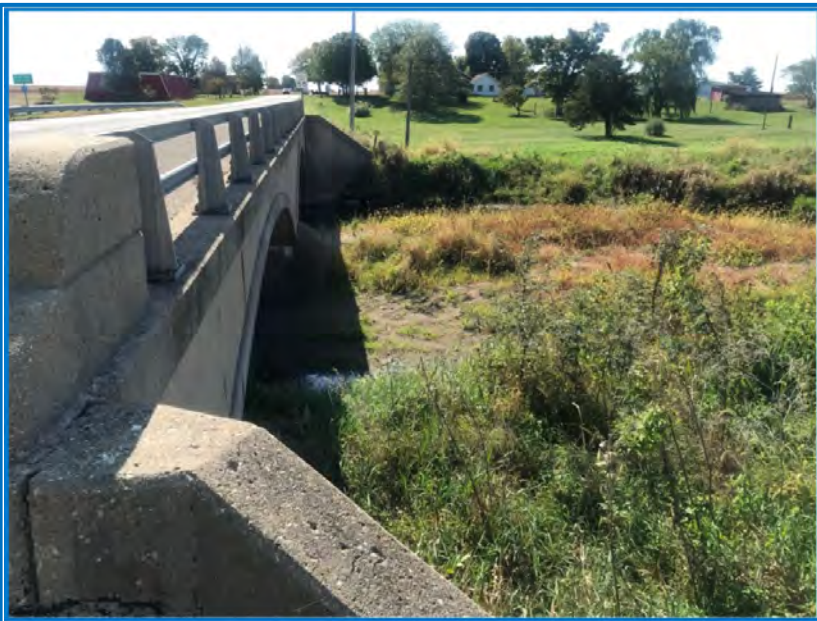
Photo 7 – View of the west side of the US 41 bridge over Coal Creek facing south (10/8/2019).
