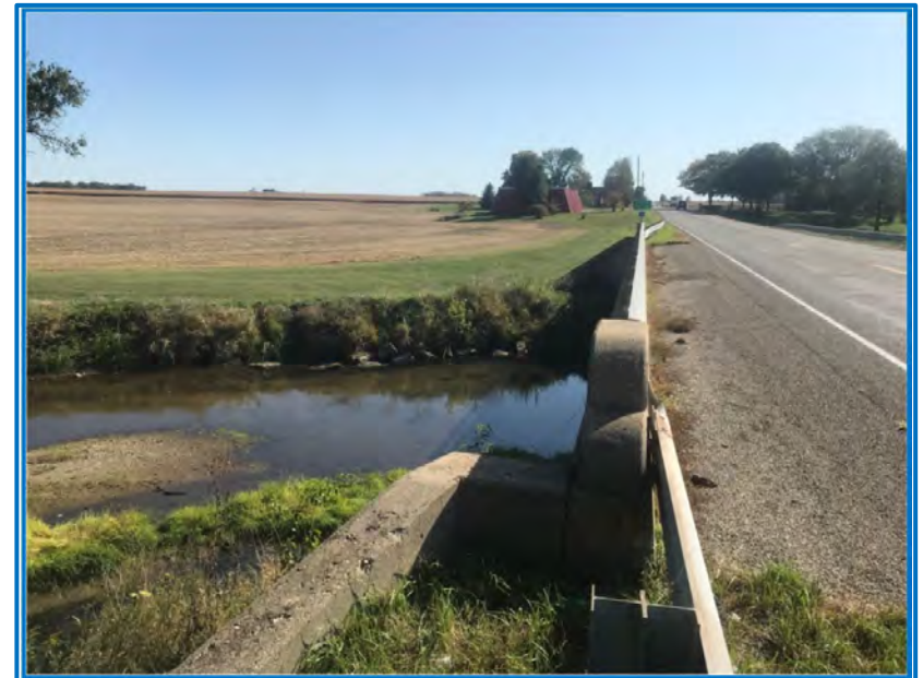
Photo 8 – View of the east side of the US 41 bridge over Coal Creek facing south (10/8/2019).
