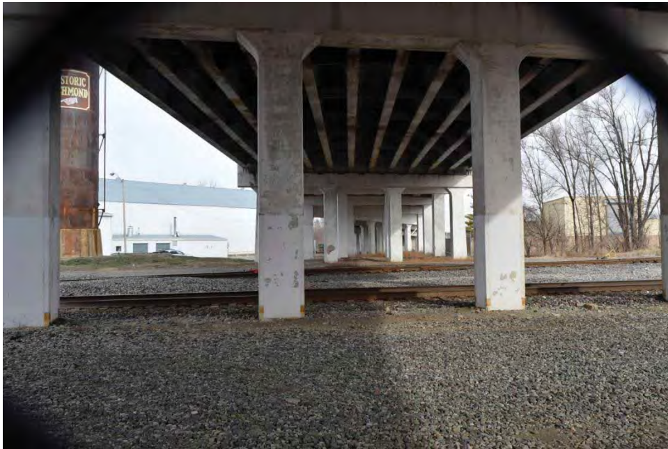
Photograph 36. View of the railyards and the underside of the US 27 bridge from North E Street, facing north.
