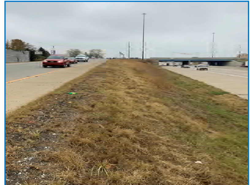
Photo 8 - View of WB I-465 entrance ramp at the Emerson Avenue and I-465 interchange facing west (10/20/2020).
