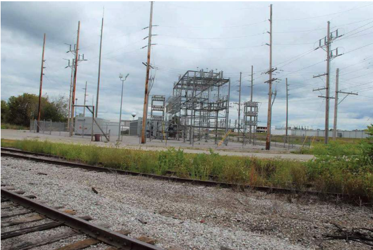
19. An electrical substation sits on Swager Road west of the railroad track at the east end of the APE.
