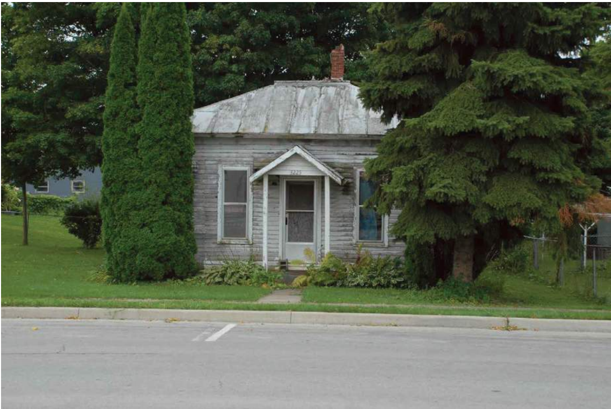
5. The small, hipped roof house (151-017-07041) at 103 West Albion Street is an example of a Contributing-rated structure in the APE.
