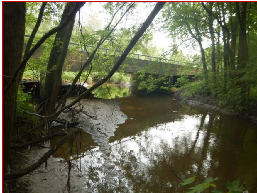
Photo 56. Looking north at Bear Creek from the southwestern quadrant of the intersection of Bear Creek and SR 1.
