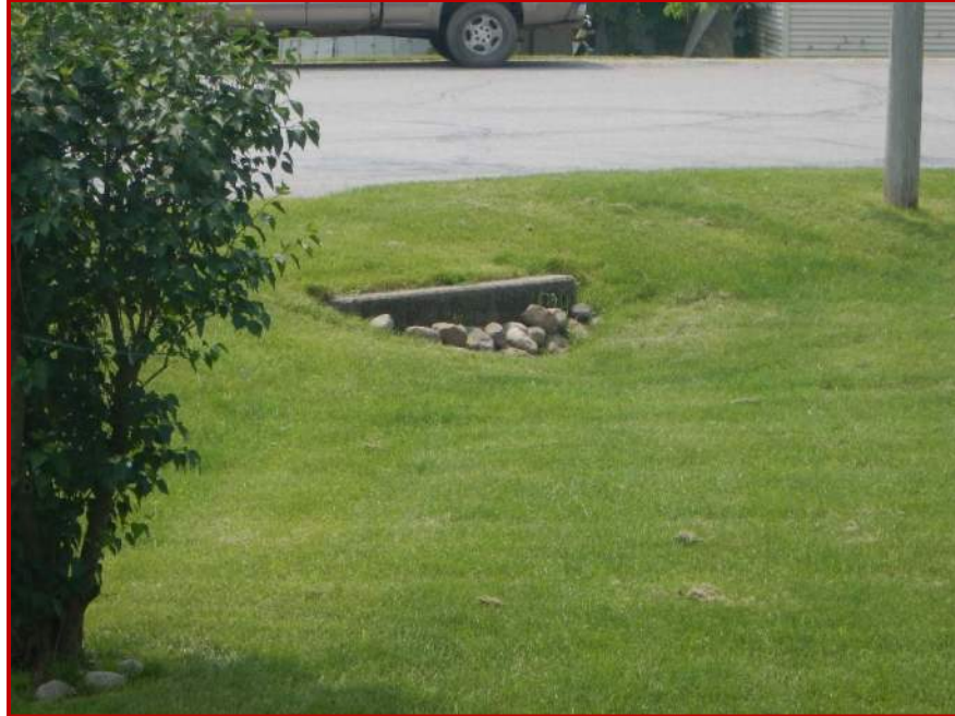
Photo 25. Looking south at a culvert along the intersection of SR 1 and Washington Street.
