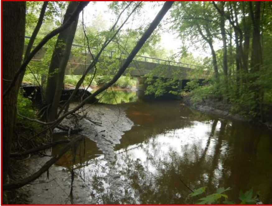
Photo 3. Looking northeast, upstream, along Bear Creek, from the southwest quadrant of the crossing of SR 1 over Bear Creek.
