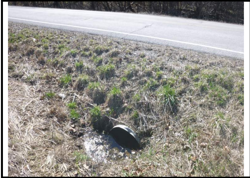
Looking at the north end of a 12" corrugated metal pipe (CMP) under SR 16 that collects farm field drainage. Culvert is approximately 300' east of the Fire Station driveway.
