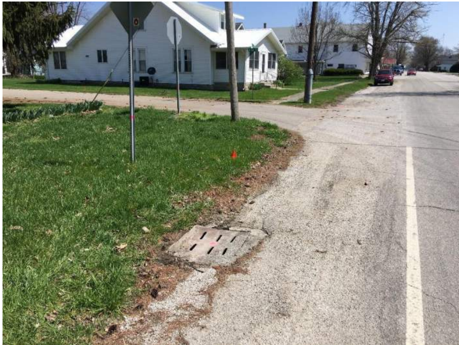
Sub-standard storm sewer at 1 st Street looking east.
