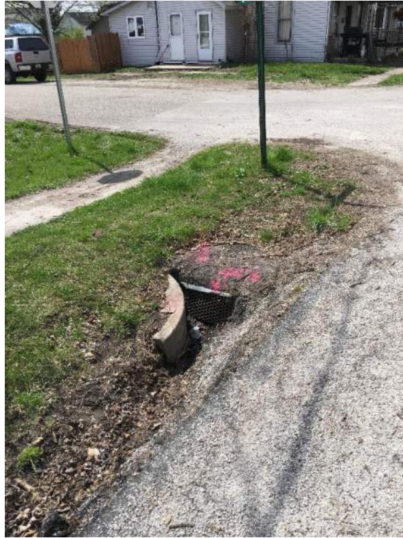
Drainage structure at the southeast corner of Chandler Street and SR 16 looking southwest.
