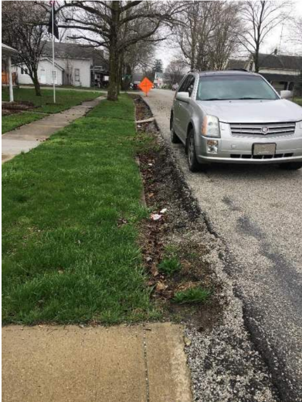
Drainage and safety concerns along the south side of SR 16 near Chandler Street.
