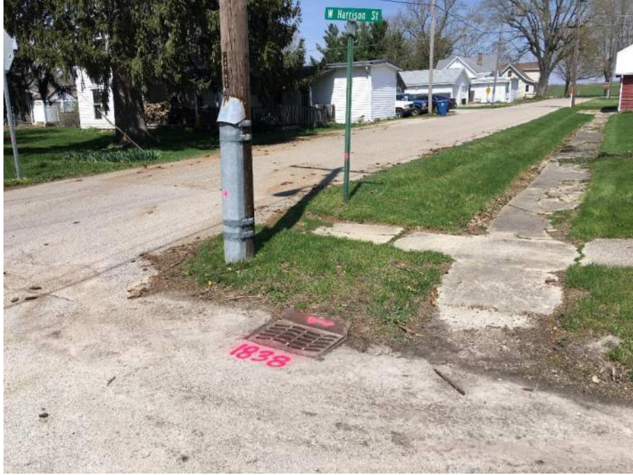
Deteriorated sidewalk at 1 st Street looking north.
