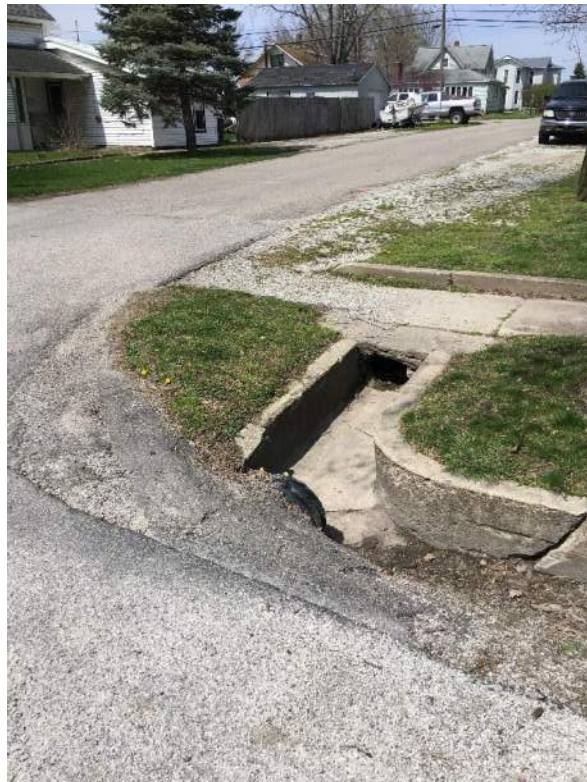
Drainage structure at northeast corner of Chandler Street and SR 16 looking north.
