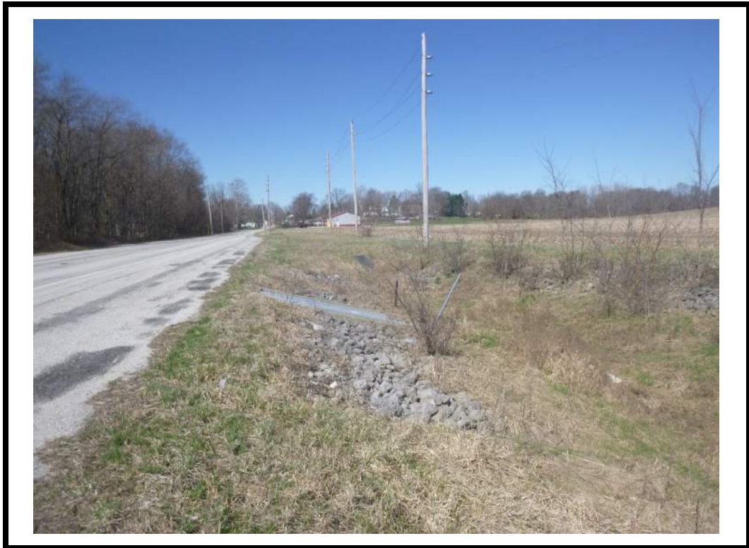
Looking west from the old culvert under SR 16 before the stream was relocated through a box culvert east of the culvert. Ditch will end at the culvert, approximately 800' east of the Fire Station driveway.
