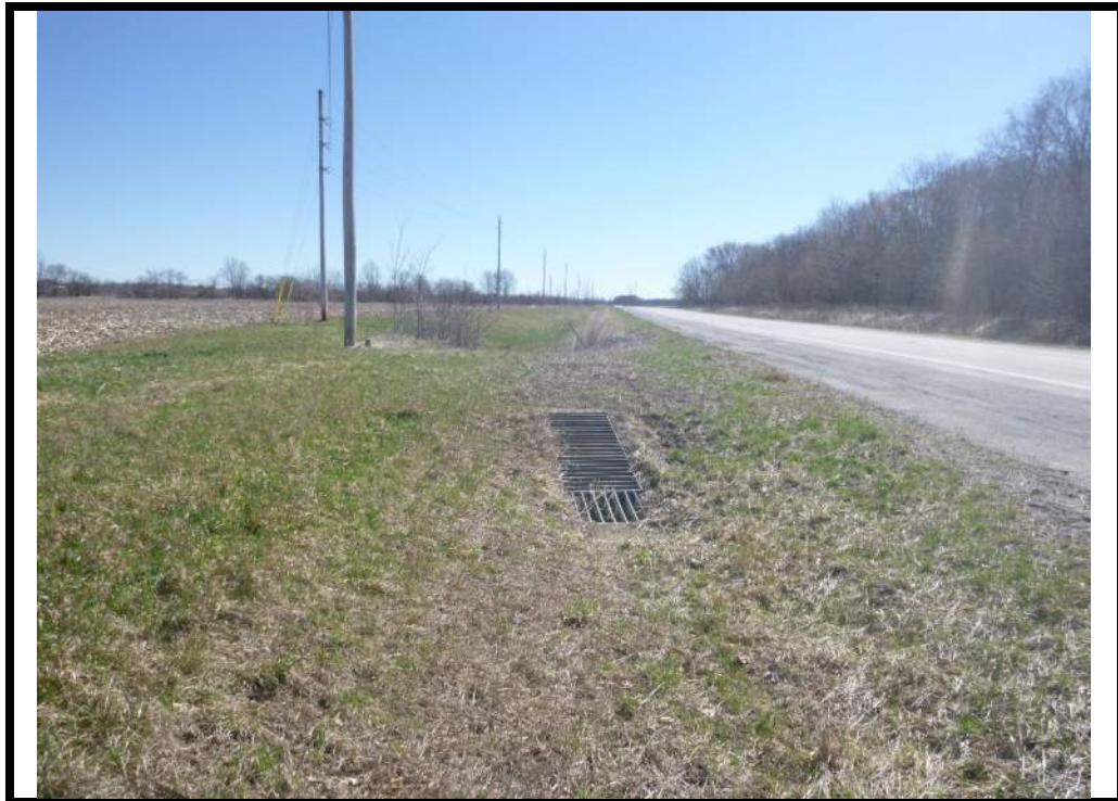
Looking east at the farm drive culvert approximately 725' east of the Fire Station driveway. Culvert will be replaced.
