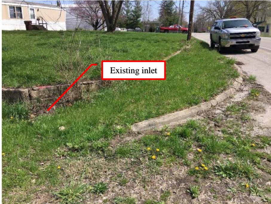
Silt and weeds on roadway at North Street looking east.
