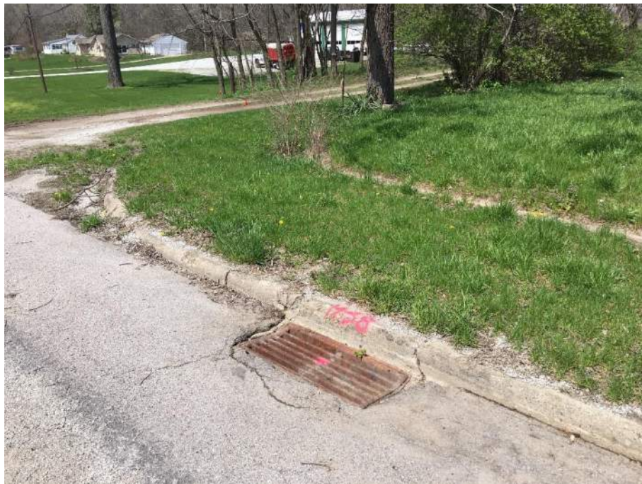
At North Street looking northwest at deteriorated curb and cracked pavement.
