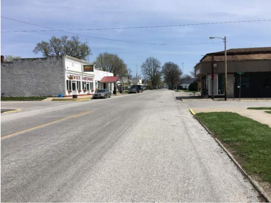
Overlay of pavement leaving little curb height for drainage at Payson Street looking east.
