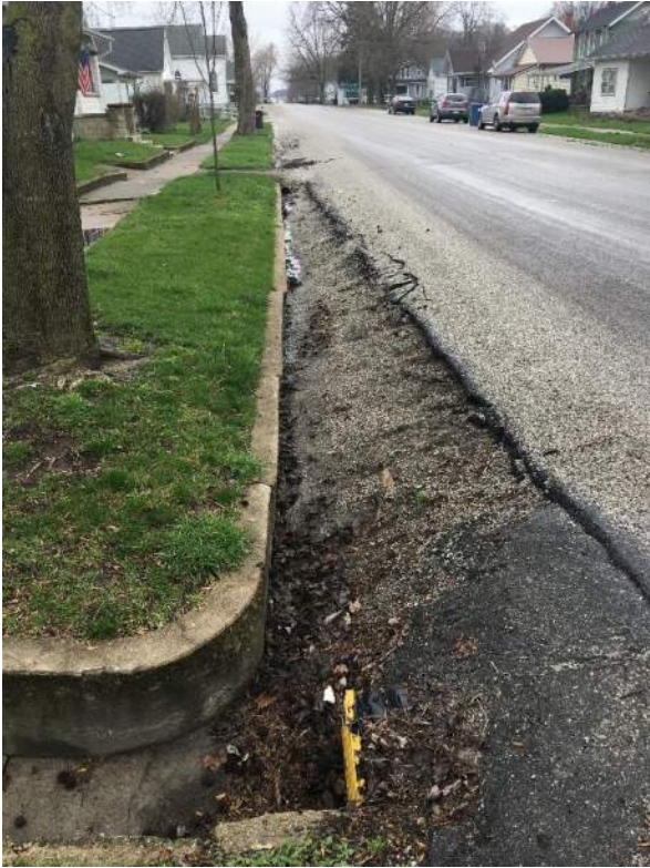
Drainage and safety concern along the north side of SR 16 at Chandler Street.
