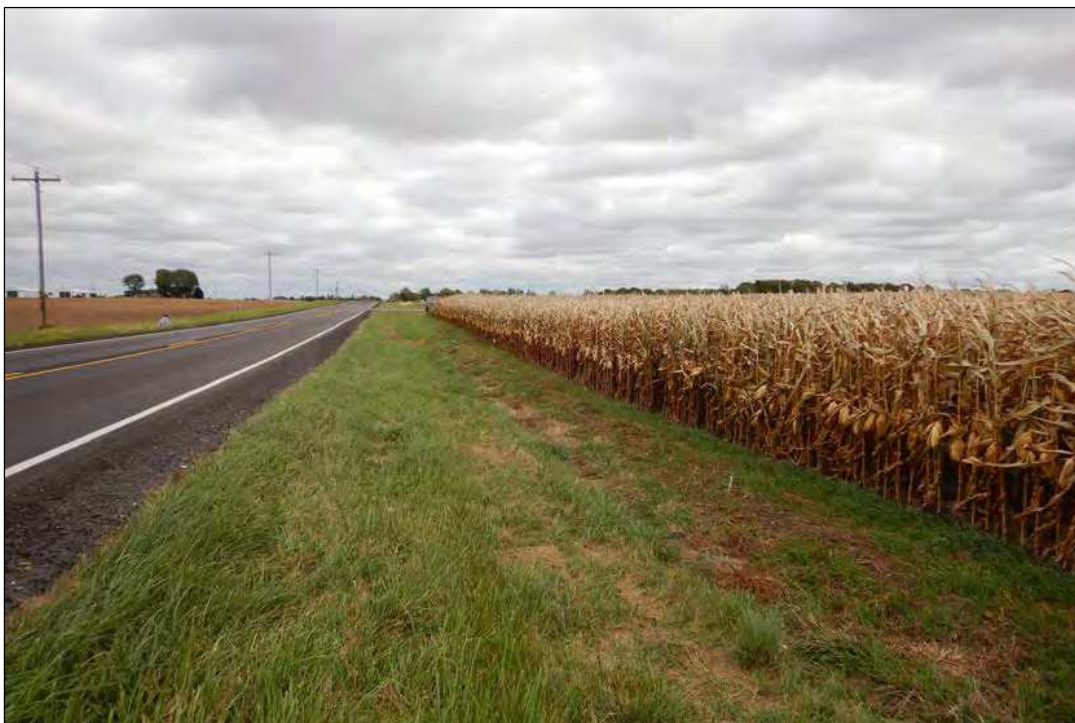
Photo 2: Roadway embankment south of SR 234 and west of the project culvert, facing east.
