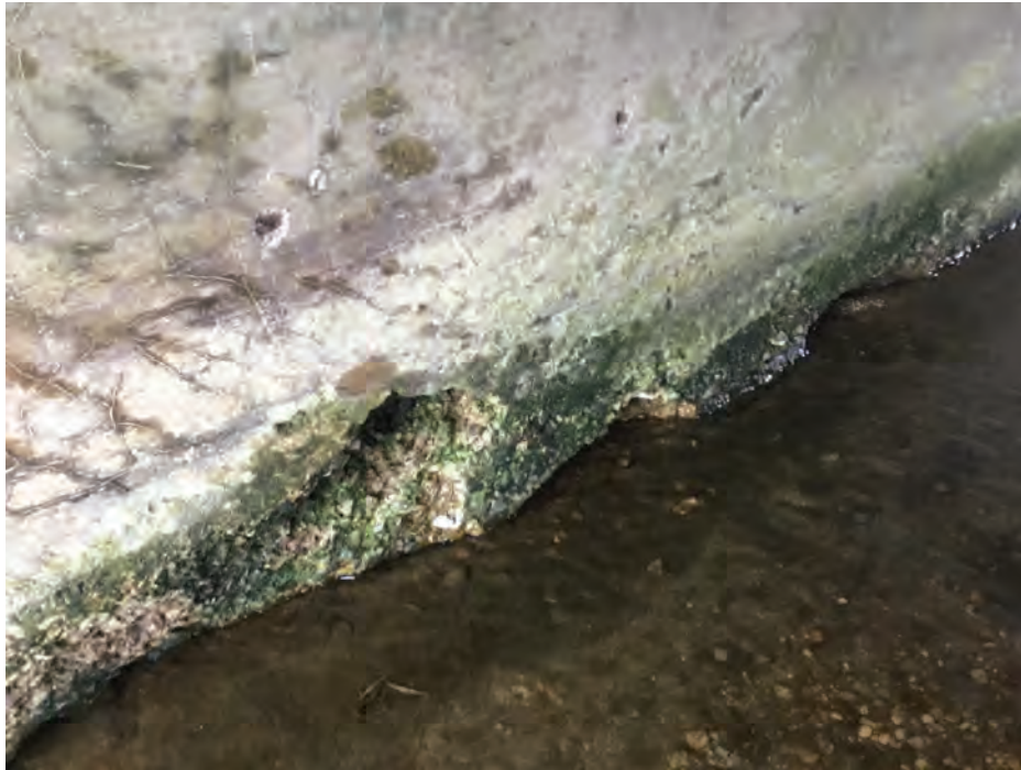
PHOTO 10 Condition Description East abutment has spalling about the water line
