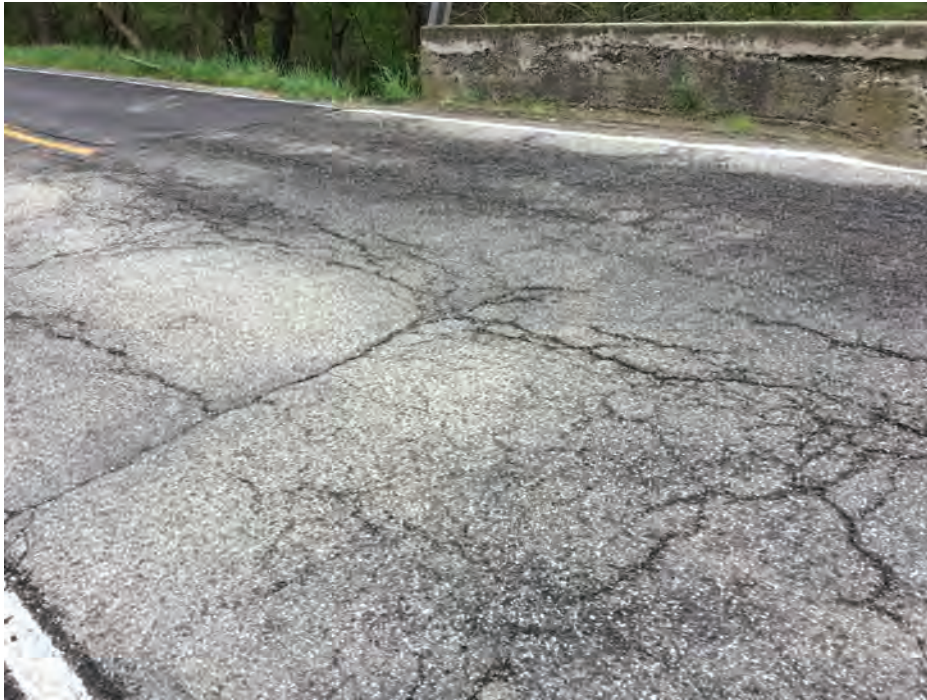
PHOTO 3 Condition Description Pavement condition above culvert
