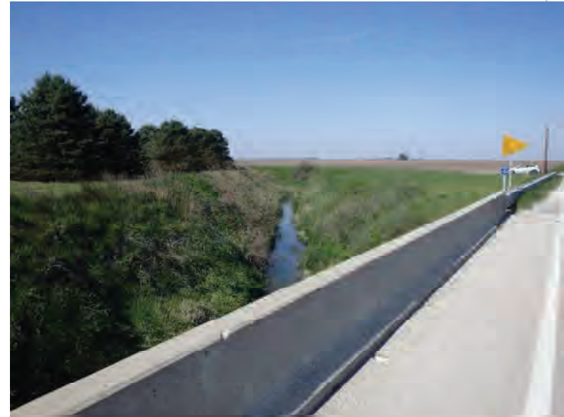
Picture 792: looking southwest, downstream, along Holder Ditch from the top of the structure 026-86-05817 B on the south side of SR 26, 05/07/2020 (Exhibit 6AT)
