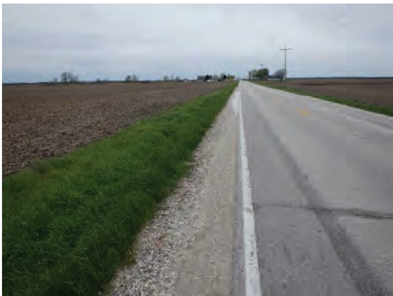
Picture 693: looking west along a roadside ditch on the south side of SR 26, 05/04/2020 (Exhibit 6AK)
