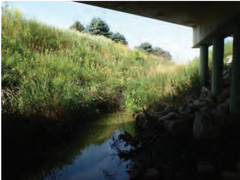
Picture 793: looking southwest, downstream, along Holder Ditch from beneath the structure, 07/19/2019 (Exhibit 6AT)
