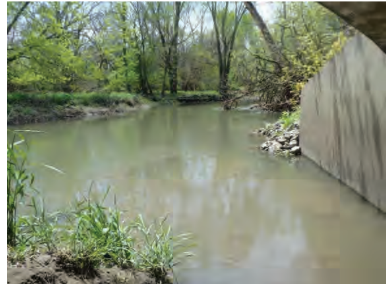
Picture 528: Looking southwest, downstream, along Big Pine Creek, from the southern opening of the structure, 05/04/2020 (Exhibit 6AB)
