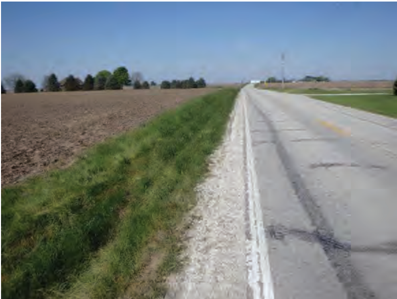
Picture 801: looking west along a roadside ditch on the south side of SR 26, east of Holder Ditch and west of N 1100 E, 05/07/2020 (Exhibit 6AT)
