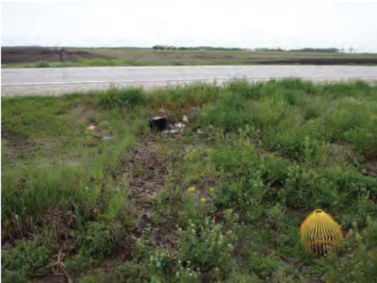
Picture 645: looking north at the south opening of structure CLV 026 86 18.25 and the start of Channel 7 on the south side of SR 26, 05/04/2020 (Exhibit 6AI)
