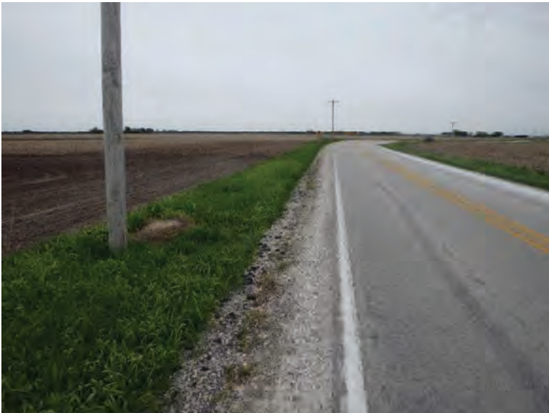
Picture 729: looking east along a roadside ditch on the north side of SR 26, east of N 725 E and west of N 875 E, 05/04/2020 (Exhibit 6AO)
