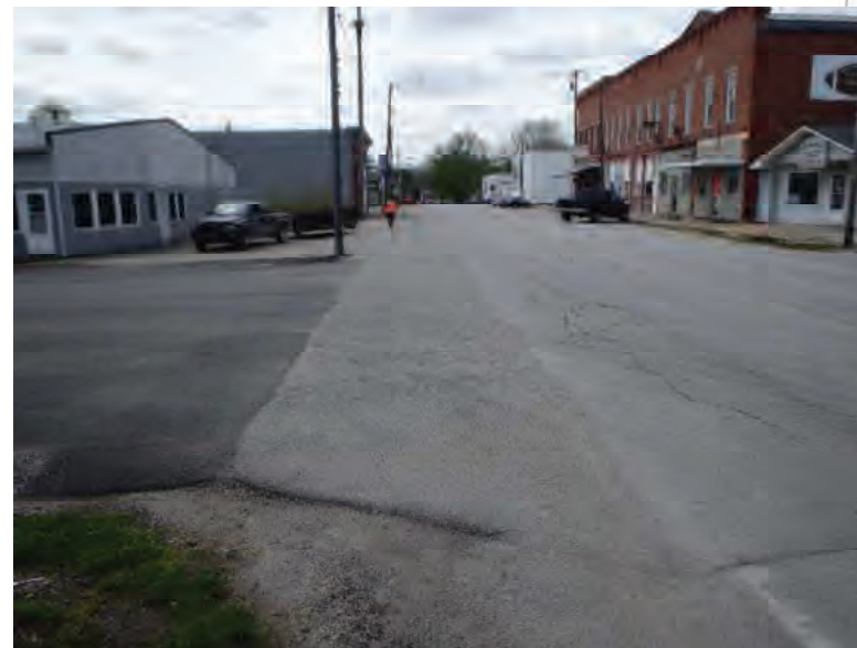
Picture 566: Looking west, toward the southern junction of SR 26 and SR 55, along the southern side of SR 26 within Pine Village, 05/07/2020 (Exhibit 6AD)
