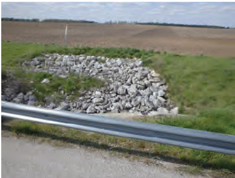
Picture 835: looking north at riprap from the top of structure CLV 026 86 23.24 over the Gephart-Magee Ditch, on the north side of SR 26; no channel present, 05/07/2020 (Exhibit 6AW)
