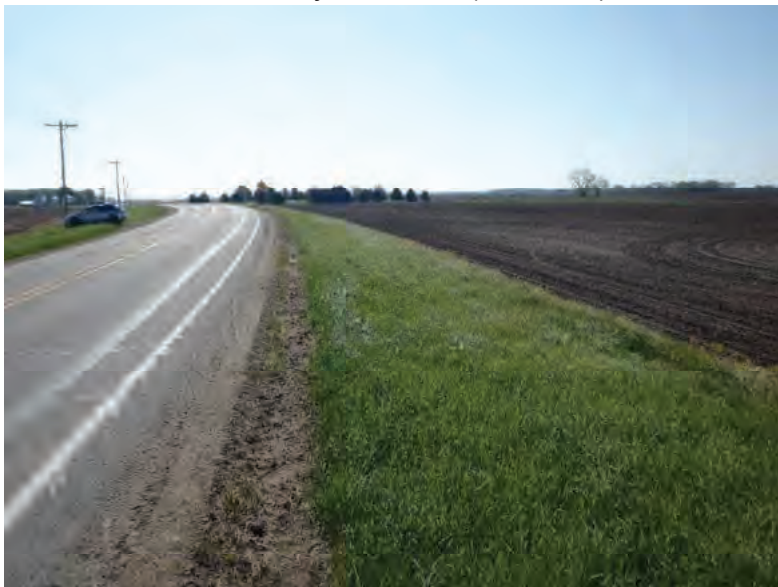
Picture 785: looking southeast along a grassed slope on the south side of SR 26, east of N 875 E and west of Holder Ditch, 05/07/2020 (Exhibit 6AS)
