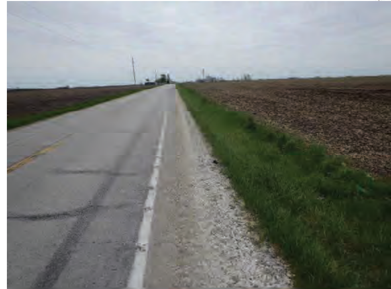
Picture 616: looking east along a roadside ditch on the south side of SR 26, 05/04/2020 (Exhibit 6AG and Exhibit 6AH)
