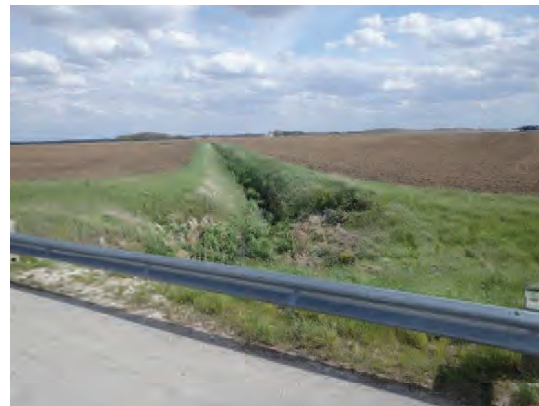
Picture 838: looking southeast, downstream, along the Gephart-Magee Ditch from the top of the structure on the south side of SR 26, 05/07/2020 (Exhibit 6AW)
