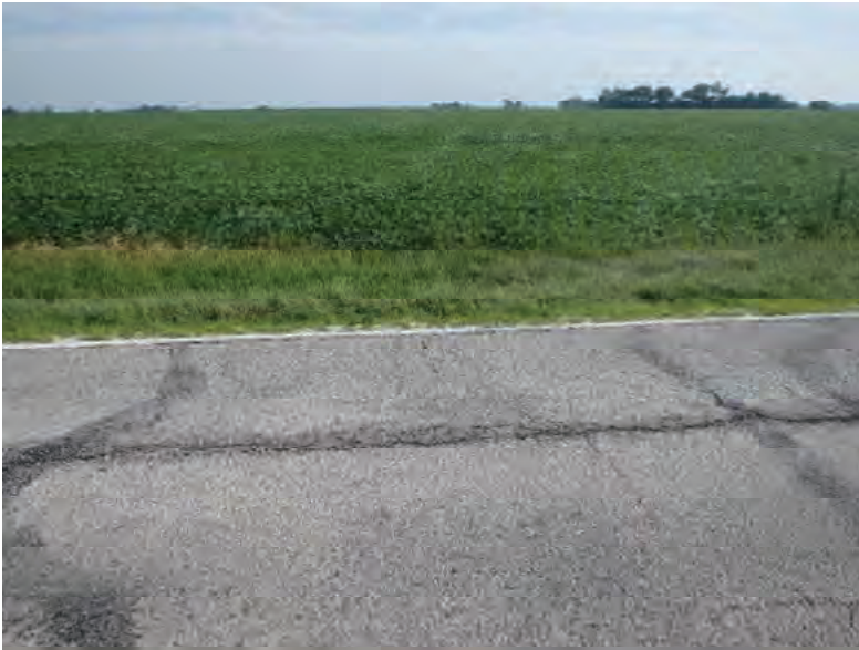
Picture 771: looking north at the mostly buried opening of structure CLV 026 86 21.52 within a roadside ditch on the north side of SR 26, 07/19/2019 (Exhibit 6AR)
