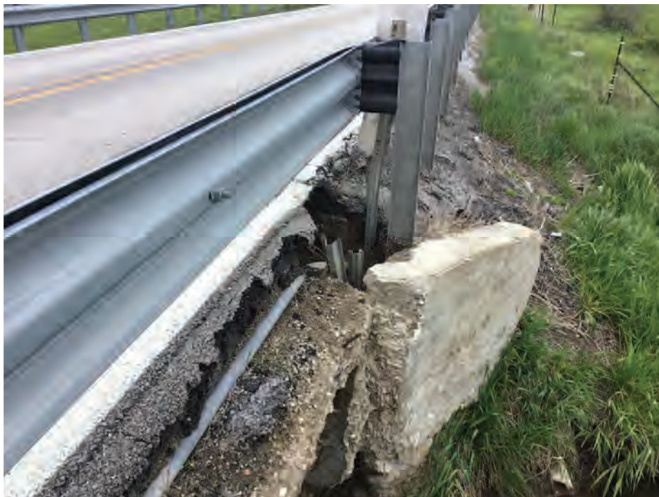
PHOTO 13 Condition, Maintenance - Culvert Description Erosion occurring at SE corner
