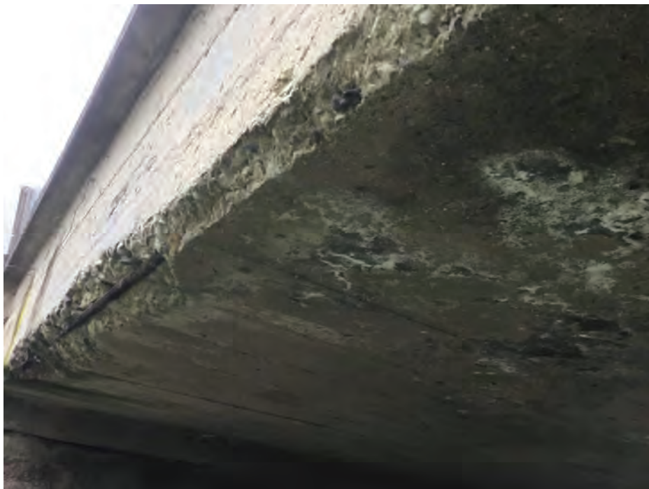
PHOTO 12 Condition Description Bottom of slab has corner spall on N end
