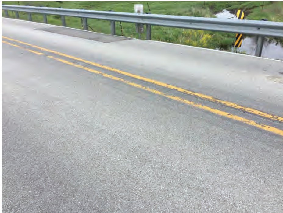
PHOTO 3 Condition Description Pavement condition above culvert
