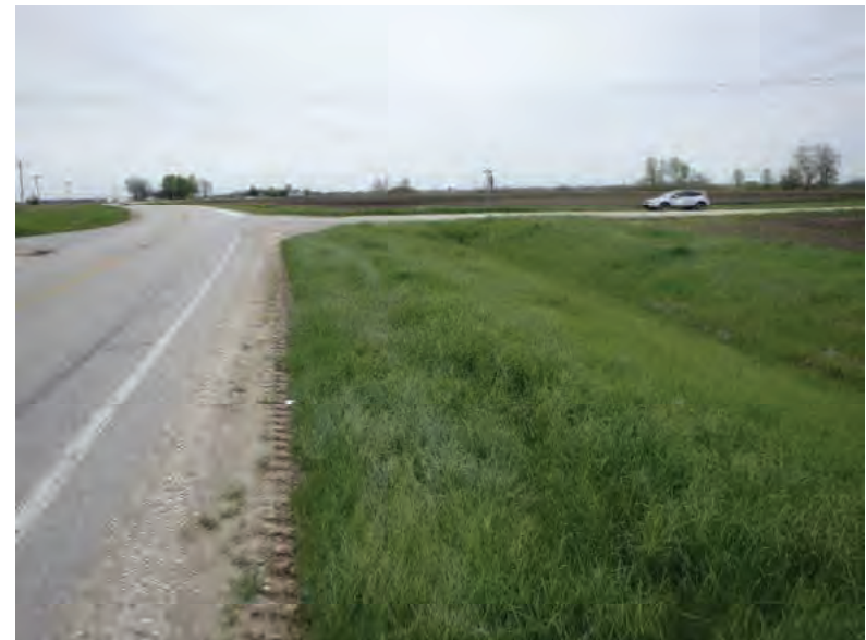
Picture 650: looking east, toward N 600 E, along a roadside ditch on the south side of SR 26, 05/04/2020 (Exhibit 6AI)
