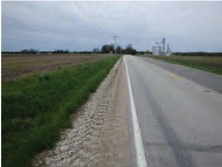
Picture 581: looking west along a roadside ditch on the south side of SR 26, 05/04/2020 (Exhibit 6AE)
