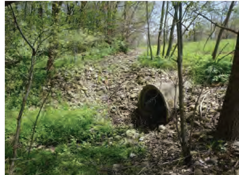
Picture 512: Looking east at the northern opening to the structure and riprapped roadside ditch leading to it, 05/04/2020 (Exhibit 6AB)
