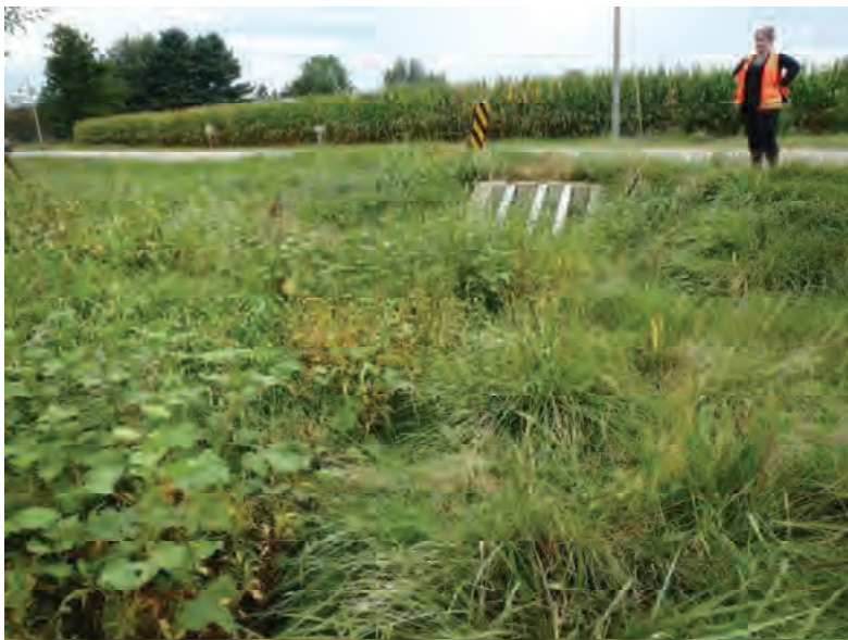
Picture 928: Looking northwest at the opening of the structure and lack of a defined channel with an OHWM, 09/01/2020 (Exhibit 6X)
