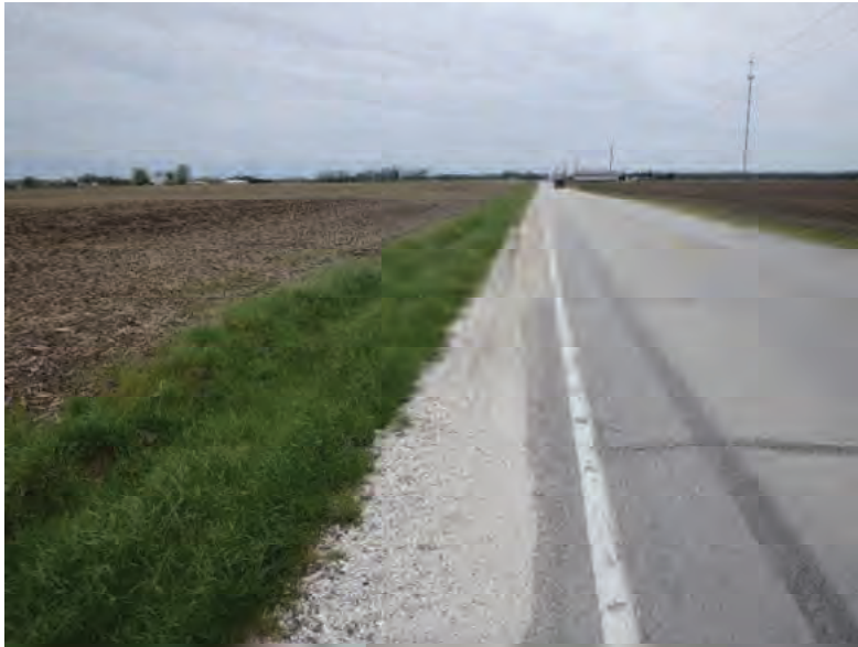
Picture 615: looking west along a roadside ditch on the south side of SR 26, 05/04/2020 (Exhibit 6AG)
