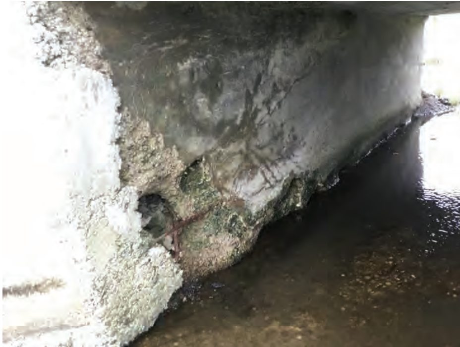
PHOTO 8 Condition Description East abutment also showing spalled area at NE corner
