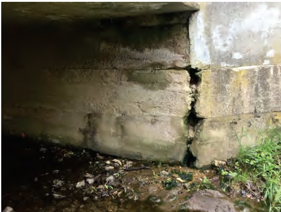
PHOTO 10 Condition Description Spalled areas on concrete at NW corner
