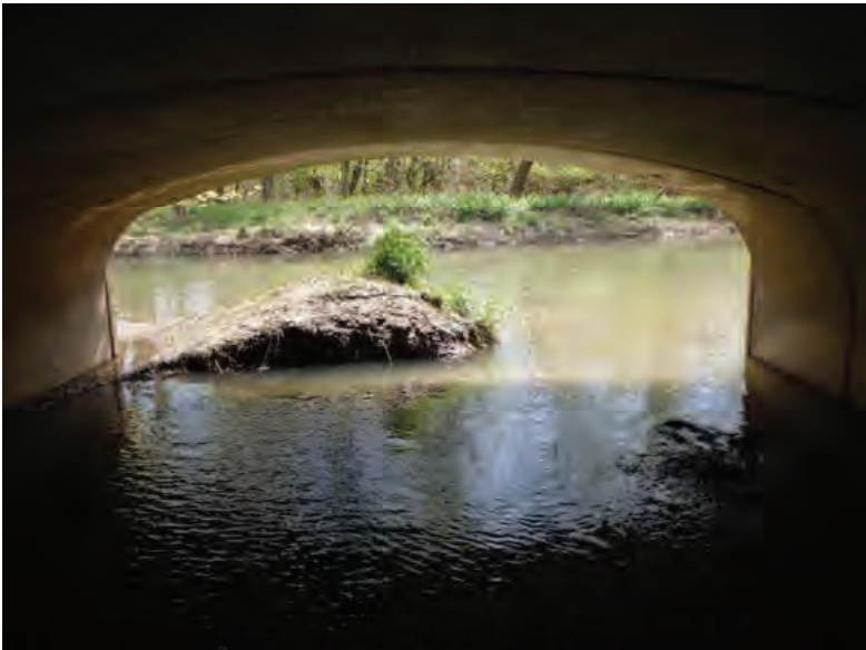
Picture 527: Looking south, downstream, at the junction of UNT7 to Big Pine Creek and Big Pine Creek, from within the structure, 05/04/2020 (Exhibit 6AB)
