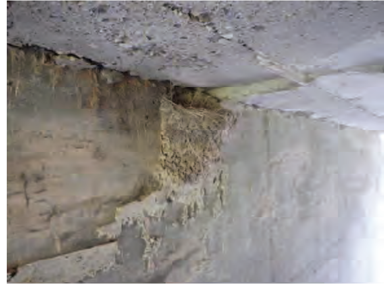
Picture 894: looking at a nest located on the west wall of the underneath side of the structure, 09/11/2019 (Exhibit 6AZ)
