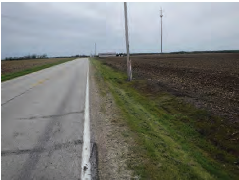
Picture 613: looking west along a roadside ditch on the north side of SR 26, 05/04/2020 (Exhibit 6AG)
