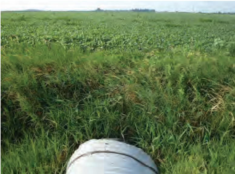
Picture 665: looking south over the south opening of structure CLV 026 86 18.49, at Wetland 25, on the south side of SR 26, east of N 600 E, 07/19/2019 (Exhibit 6AJ)
