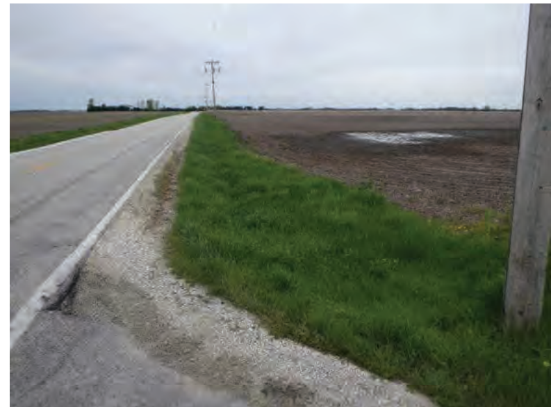
Picture 762: looking west along a roadside ditch on the north side of SR 26, adjacent to N 875 E, 05/04/2020 (Exhibit 6AQ)
