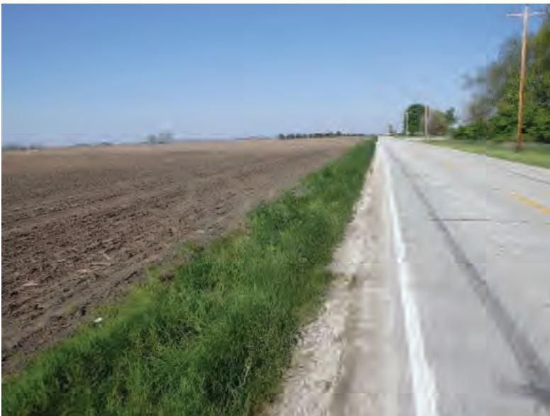
Picture 809: looking west along a roadside ditch on the south side of SR 26, east of Holder Ditch and west of N 1100 E, 05/07/2020 (Exhibit 6AU)
