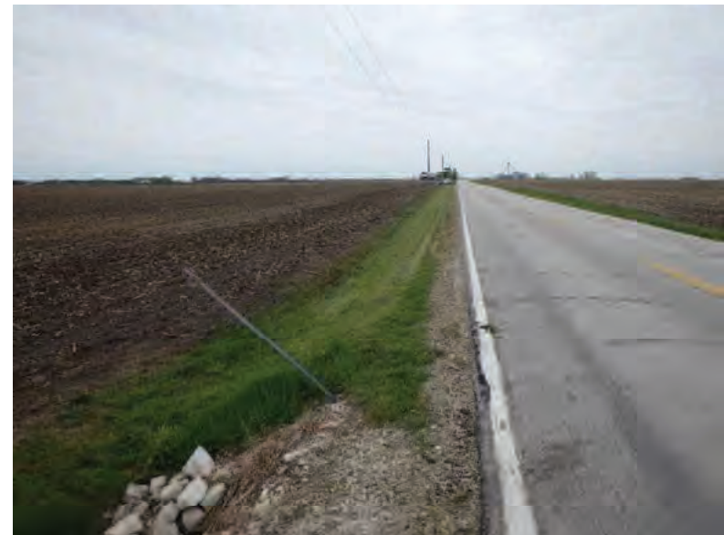
Picture 614: looking east along a roadside ditch on the north side of SR 26, 05/04/2020 (Exhibit 6AG)
