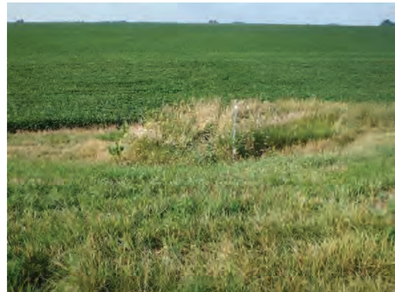
Picture 782: looking southwest at the mostly buried opening of structure CLV 026 86 20.87 within a roadside ditch, on the south side of SR 26, east of N 875 E and west of Holder Ditch, 07/19/2019 (Exhibit 6AS)
