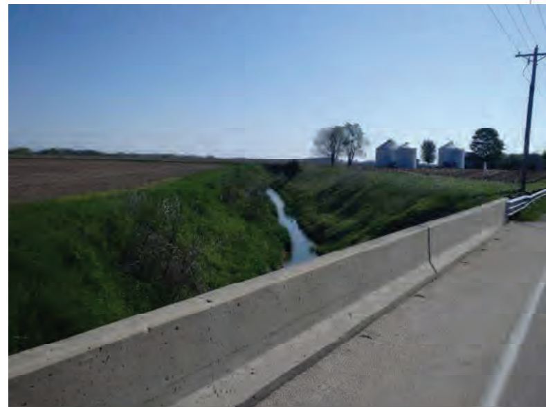
Picture 796: looking northeast, upstream along Holder Ditch from the top of the structure on the north side of SR 26, 05/07/2020 (Exhibit 6AT)
