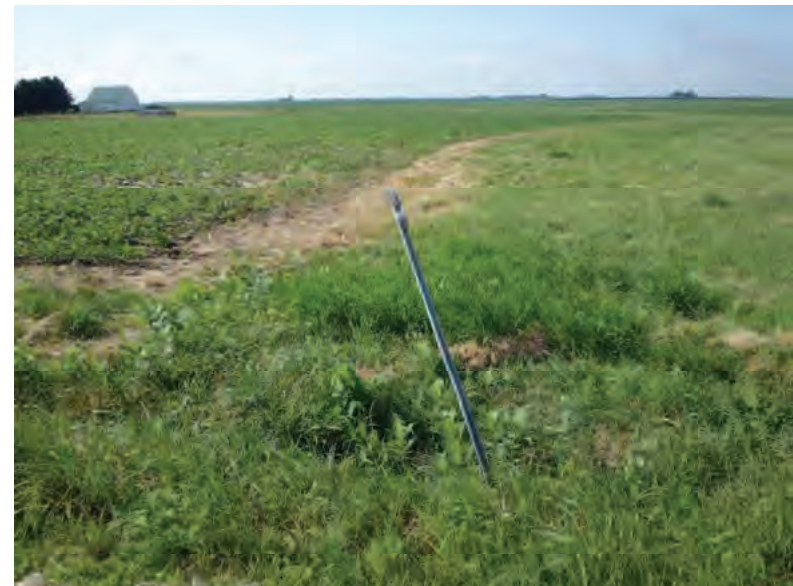
Picture 770: looking south at the mostly buried opening of structure CLV 026 86 21.52 within the roadside ditch, and a grassed waterway along the south side of SR 26; no channel present, 07/19/2019 (Exhibit 6AR)
