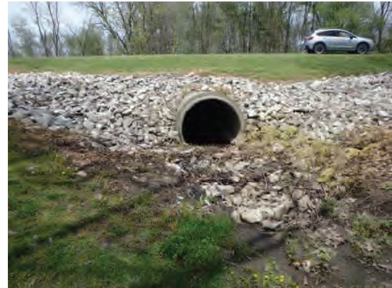
Picture 508: Looking north at the southern opening of structure CV 026 86 15.45 on the south side of SR 26, 05/04/2020 (Exhibit 6AB)
