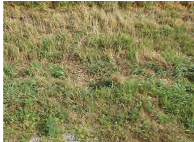
Picture 752: looking north at the mostly buried south opening of structure CLV 026 86 21.22 and a roadside ditch on the north side of SR 26, adjacent to Wetland 29 and west of N 875 E, 07/19/2019 (Exhibit 6AQ)
