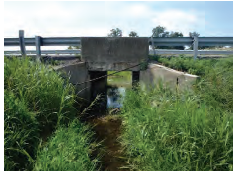
Picture 884: looking south, downstream, along UNT1 to Little Pine Creek at the north opening of the structure, on the north side of SR 26, adjacent to Wetland 35, 07/19/2019 (Exhibit 6AZ)
