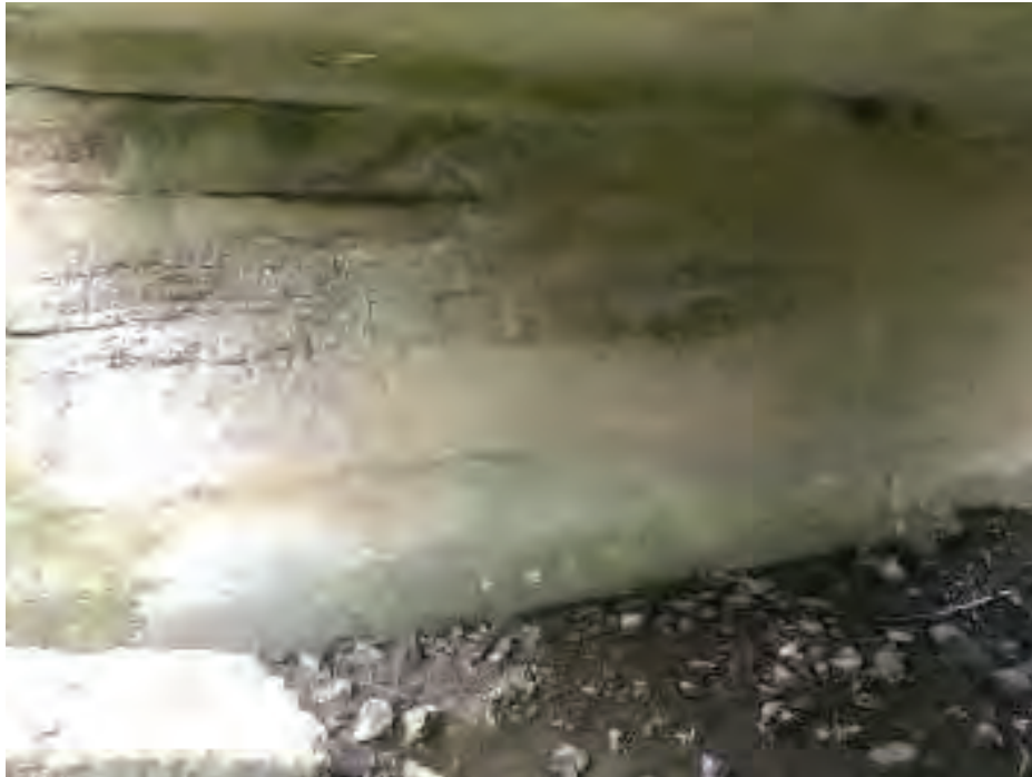
PHOTO 9 Condition Description East abutment condition
