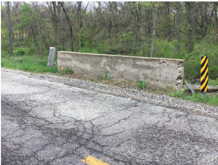
PHOTO 4 Condition Description North parapet wall condition
