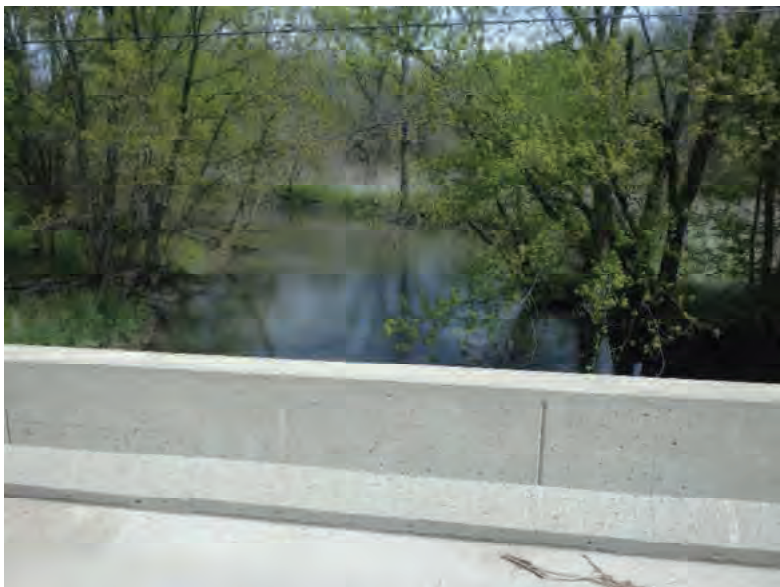
Picture 561: Looking east along Big Pine Creek from eastern side of structure (26)55-86-05834 B, 05/04/2020 (Exhibit 6AC)
