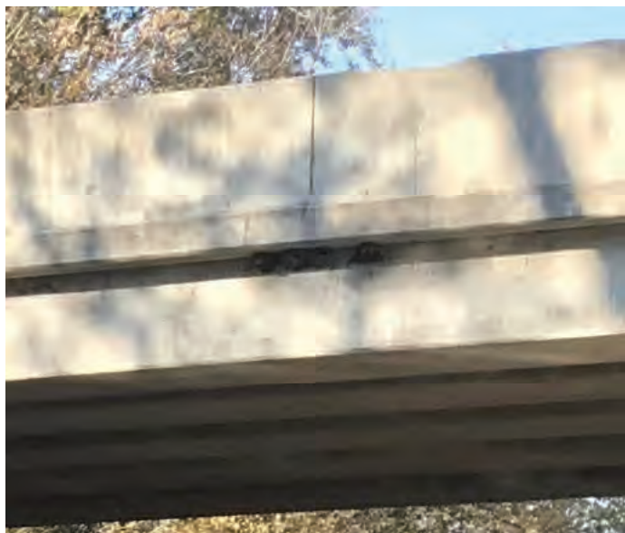
Picture 559: Looking west, at the east side of the structure and several bird nests; these nests were present in several areas on the structure 11/05/2019 (Exhibit 6AC)
