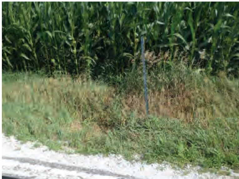
Picture 861: looking north where the mostly buried opening of the structure is, within a roadside ditch on the north side of SR 26, east of N 1150 E and west of County Line Rd, 07/19/2019 (Exhibit 6AZ)
