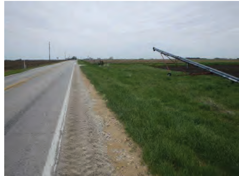
Picture 610: looking east along a roadside ditch on the north side of SR 26, 05/04/2020 (Exhibit 6AG)
