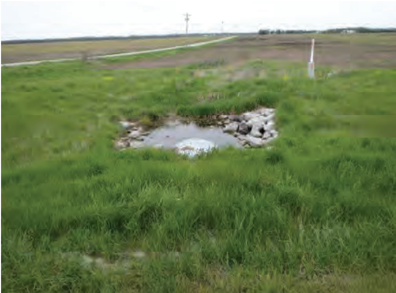
Picture 663: looking north at a scour hole backfilled with riprap adjacent to the north opening of structure CLV 026 86 18.49, east of N 600 E; no channel present, 05/04/2020 (Exhibit 6AJ)
