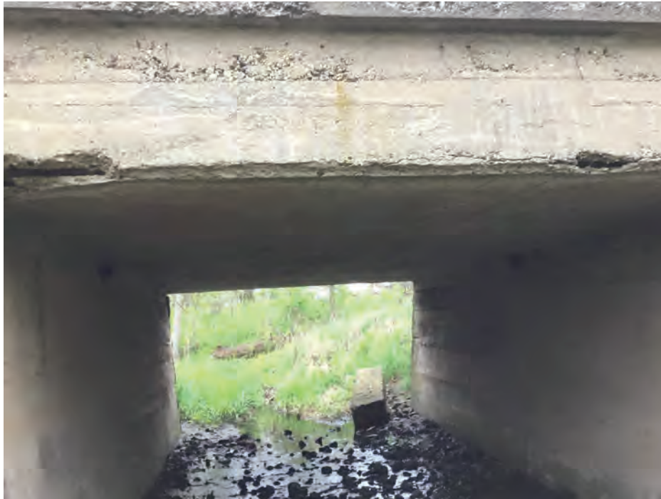
PHOTO 11 Condition Description Bottom of slab has corner spalls on S end
