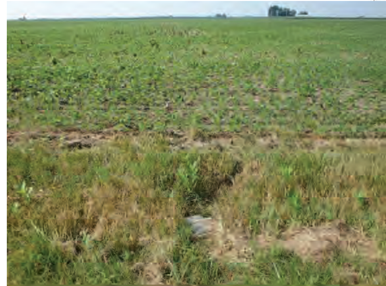
Picture 764: looking south at the mostly buried opening of structure CLV 026 86 21.22 and a roadside ditch on the south side of SR 26, east of N 875 E, 07/19/2019 (Exhibit 6AQ)
