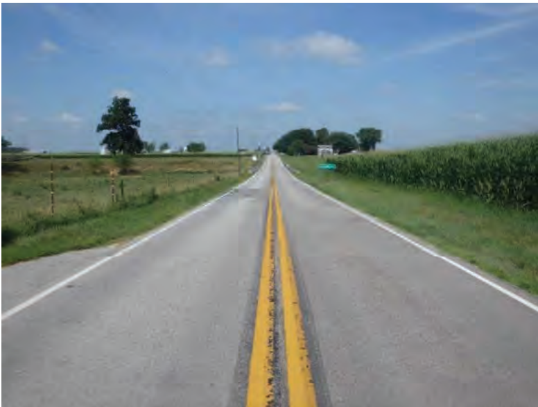
Picture 895: looking west from the eastern end of the project, 07/19/2019 (Exhibit 6AZ)
