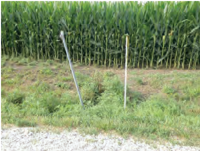
Picture 623: looking south at the mostly buried opening of structure CLV 026 86 18.00 on the south side of SR 26; no channel present, 07/19/2019 (Exhibit 6AH)
