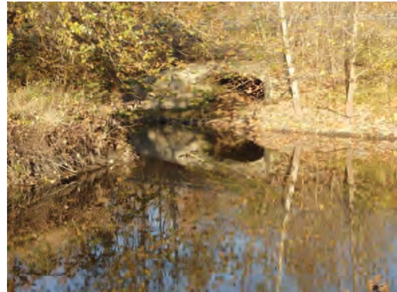
Picture 544: Looking northwest along Big Pine Creek, at the south opening of structure 026-86-08172 and junction of Big Pine Creek and UNT7 to Big Pine Creek, 11/05/2019 (Exhibit 6AB)
