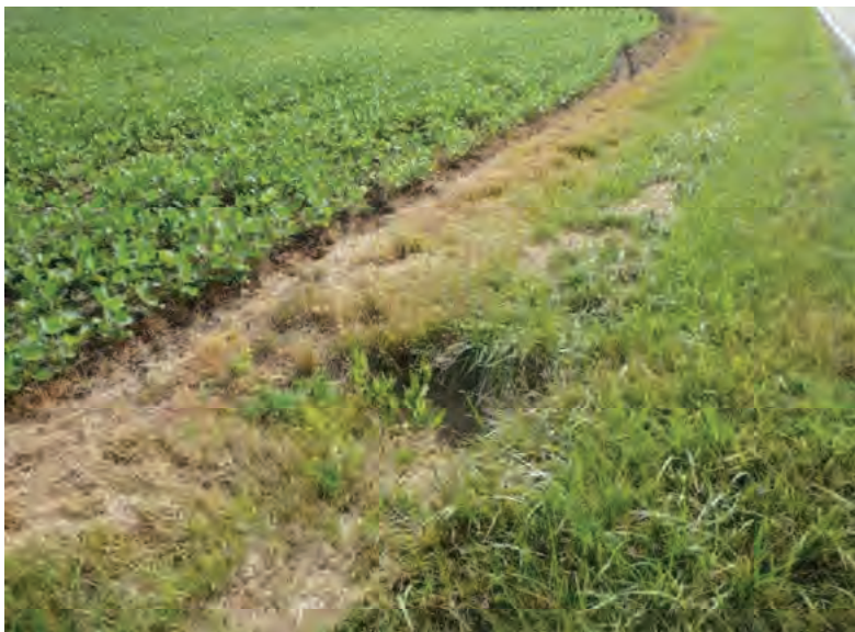
Picture 777: looking east at the completely buried opening of structure CLV 026 86 21.68 on the north side of SR 26, east of N 875 E and west of Holder Ditch, 07/19/19 (Exhibit 6AR)
