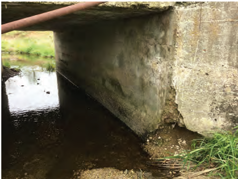
PHOTO 9 Condition Description West abutment also showing spalled area at NW corner
