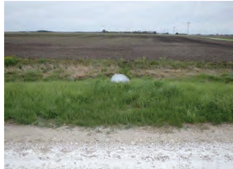
Picture 666: looking south over the south opening of structure CLV 026 86 18.49, at Wetland 25, on the south side of SR 26, east of N 600 E, 05/04/2020 (Exhibit 6AJ)
