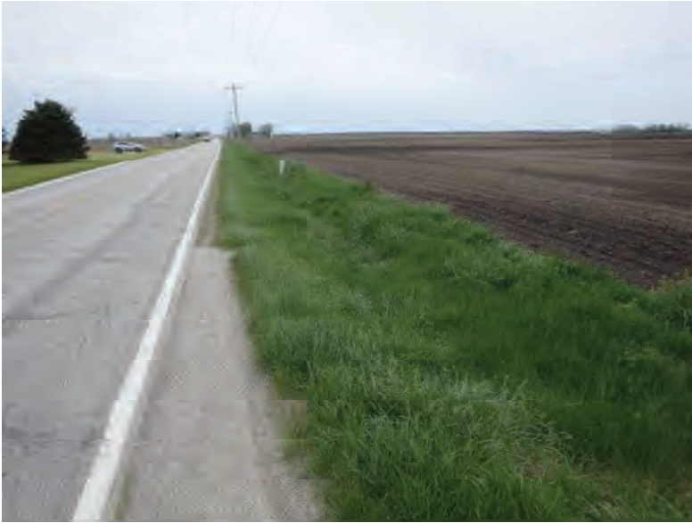
Picture 699: looking west along a roadside ditch on the north side of SR 26, east of N 725 E, 05/04/2020 (Exhibit 6AL)
