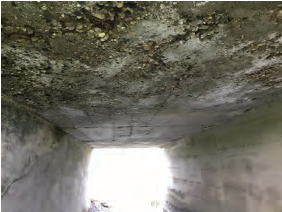
PHOTO 7 Condition Description Bottom of slab has honeycombing towards N
