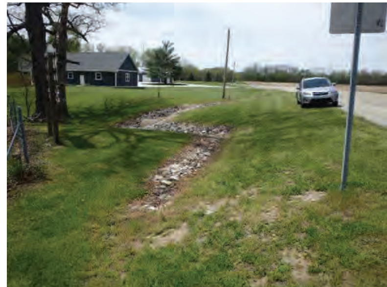
Picture 516: Looking west along the riprapped roadside ditch that leads to the south opening of structure CV 026 86 15.45 on the south side of SR 26, 05/04/2020 (Exhibit 6AB)
