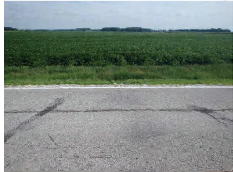
Picture 852: looking north where the buried opening of the structure is located, within a roadside ditch on the north side of SR 26, east of N 1100 E and west of N 1150 E, 07/19/2019 (Exhibit 6AY)
