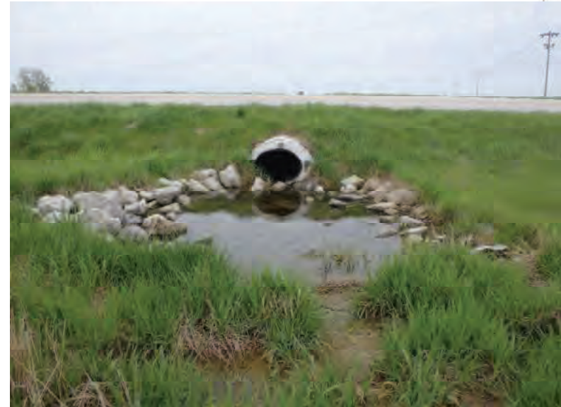
Picture 664: looking south at a scour hole backfilled with riprap adjacent to the north opening of structure CLV 026 86 18.49, east of N 600 E, 05/04/2020 (Exhibit 6AJ)
