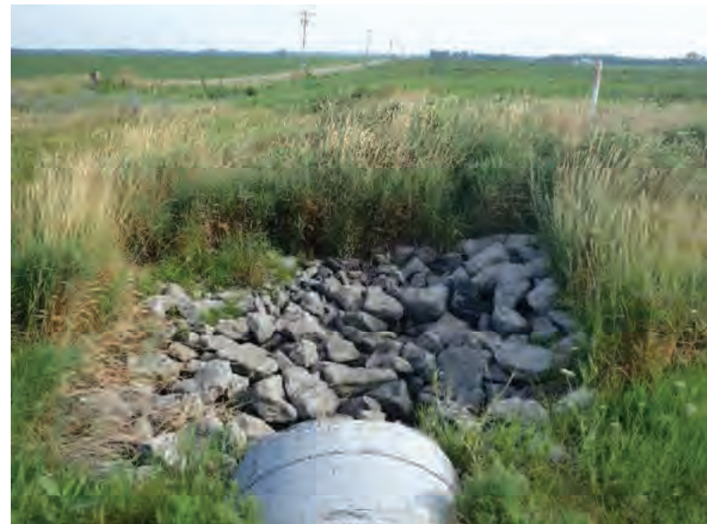
Picture 662: looking north at a scour hole backfilled with riprap adjacent to the north opening of structure CLV 026 86 18.49, east of N 600 E; no channel present 07/19/2019 (Exhibit 6AJ)
