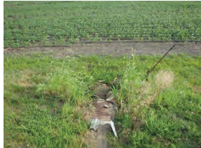
Picture 602: looking north, at the northern opening of structure CLV 026 86 17.19 on the south side of SR 26; no channel present, 07/19/2019 (Exhibit 6AF)
