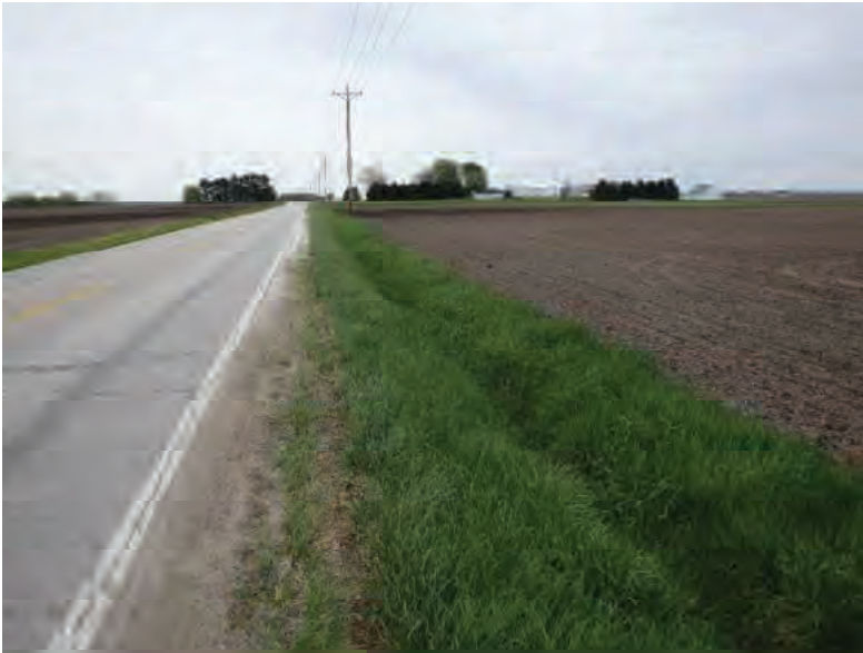
Picture 767: looking east along a roadside ditch on the south side of SR 26, east of N 875 E 05/04/2020 (Exhibit 6AR)
