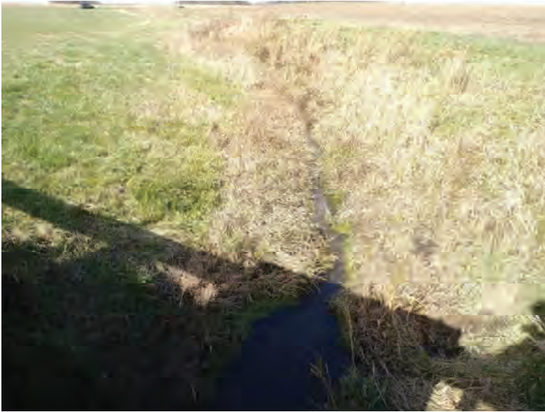
Picture 893: looking north at Wetland 35, along UNT1 to Little Pine Creek, located adjacent to the north side of the structure, east of County Line Rd., 11/06/2019 (Exhibit 6AZ)
