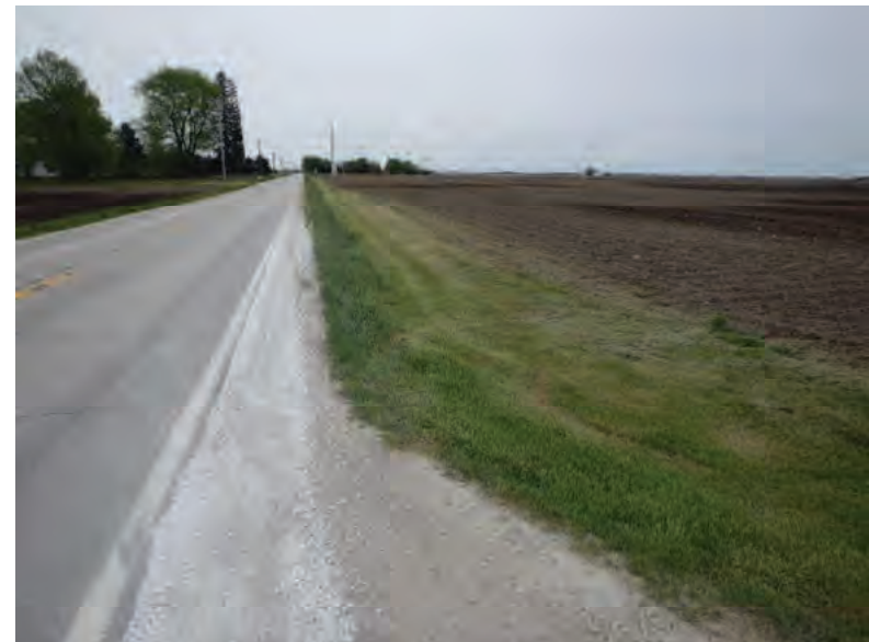
Picture 710: Looking east along a roadside ditch on the south side of SR 26, adjacent to N 725 E, 05/04/2020 (Exhibit 6AM)
