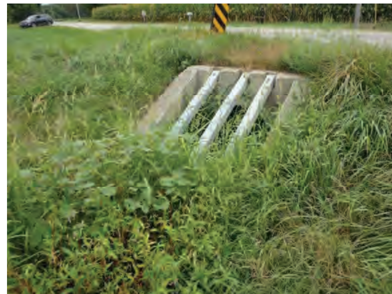
Picture 927: looking northwest at structure CLV 026 86 14.46 and the start of Channel 4, on the south side of SR 26, 09/01/2020 (Exhibit 6X)
