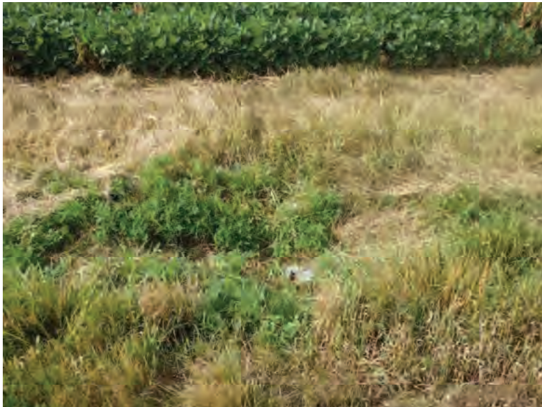
Picture 751: looking south at the mostly buried south opening of structure CLV 026 86 21.22 within a roadside ditch on the south side of SR 26, just west of N 875 E, 07/19/2019 (Exhibit 6AQ)
