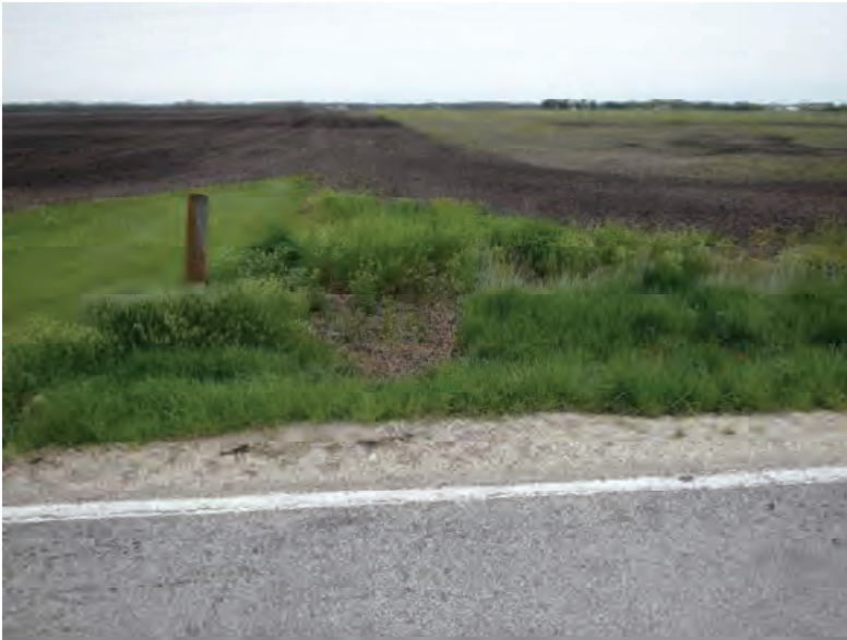
Picture 647: looking north at the roadside ditch where the north opening of structure CLV 026 86 18.25 is located, on the north side of SR 26; no channel present, 05/04/2020 (Exhibit 6AI)
