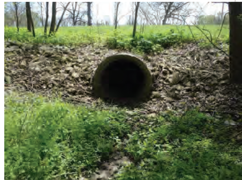
Picture 514: Looking south, downstream, along Channel 6, at the northern opening of the structure on the northern side of SR 26, 05/04/2020 (Exhibit 6AB)
