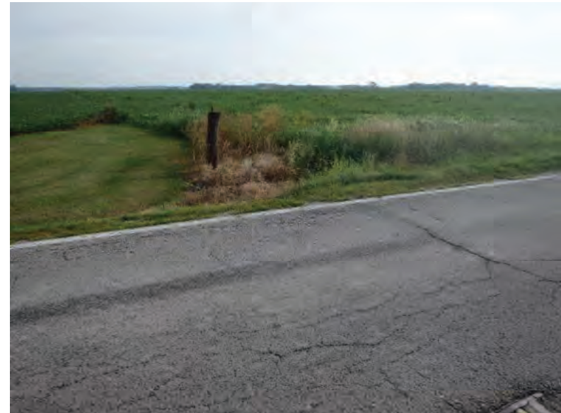
Picture 646: looking north at the roadside ditch where the north opening of structure CLV 026 86 18.25 is located, on the north side of SR 26; no channel present, 07/19/2019 (Exhibit 6AI)
