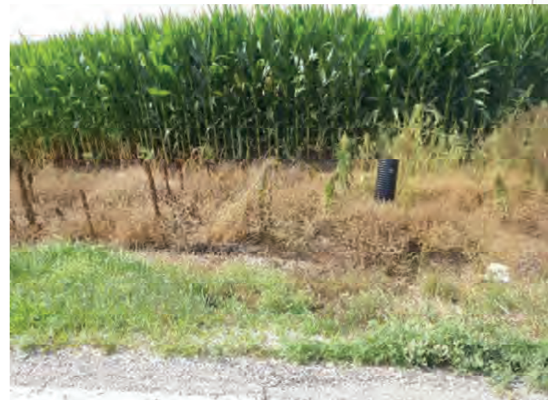
Picture 860: looking south at a stand pipe located adjacent to the south opening of structure CLV 026 86 24.14 on the south side of SR 26, east of N 1150 E and west of County Line Rd, 07/19/2019 (Exhibit 6AY)
