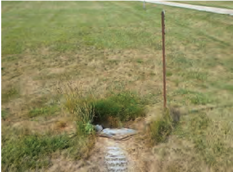
Picture 735: looking south at the south opening of structure CLV 026 86 20.87 within a mown lawn on the south side of SR 26, east of N 725 E and west of N 875 E, 07/19/2019 (Exhibit 6AP)
