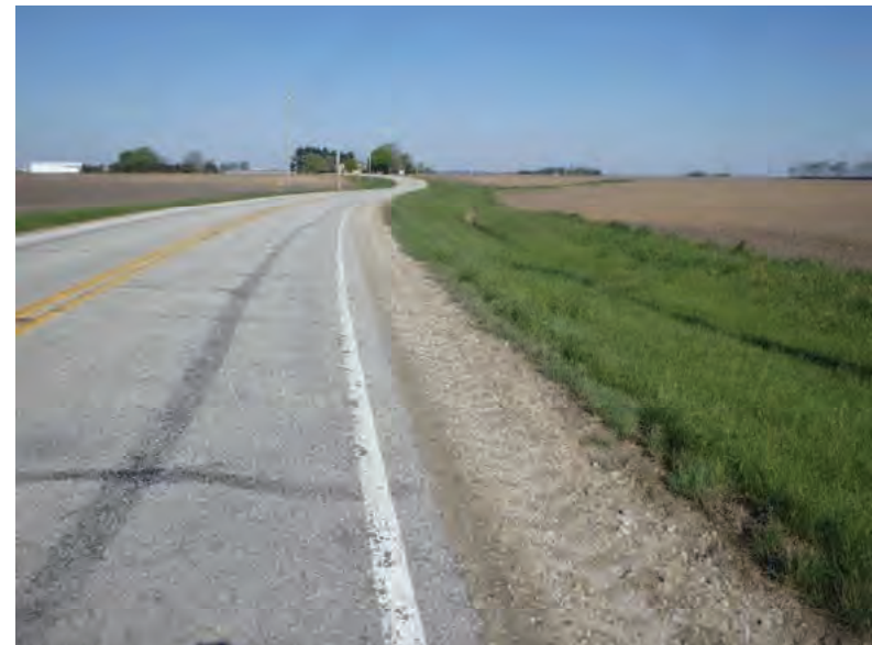
Picture 786: looking northwest along a roadside ditch on the north side of SR 26, east of N 875 E and west of Holder Ditch, 05/07/2020 (Exhibit 6AS)
