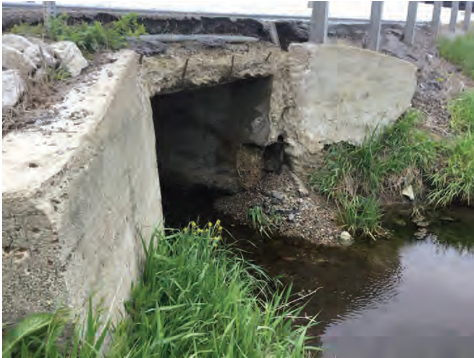
PHOTO 6 Condition Description Profile looking north also showing spalled area at SE corner
