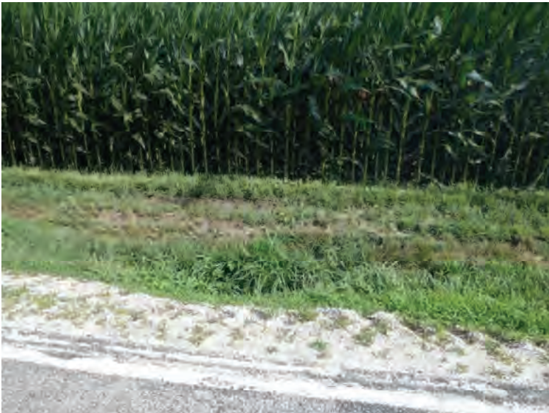
Picture 845: looking south at the mostly buried south opening of structure CLV 026 86 23.57 within a roadside ditch, east of Gephart-Magee Ditch and west of N 1100 E, 07/19/2019 (Exhibit 6AX)
