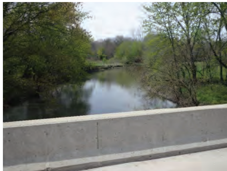
Picture 560: Looking west along Big Pine Creek from western side of structure (26)55-86-05834 B, 05/04/2020 (Exhibit 6AC)
