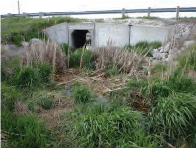
Picture 839: looking northwest, upstream, at the south opening of the structure on the south side of SR 26, 05/07/2020 (Exhibit 6AW)
