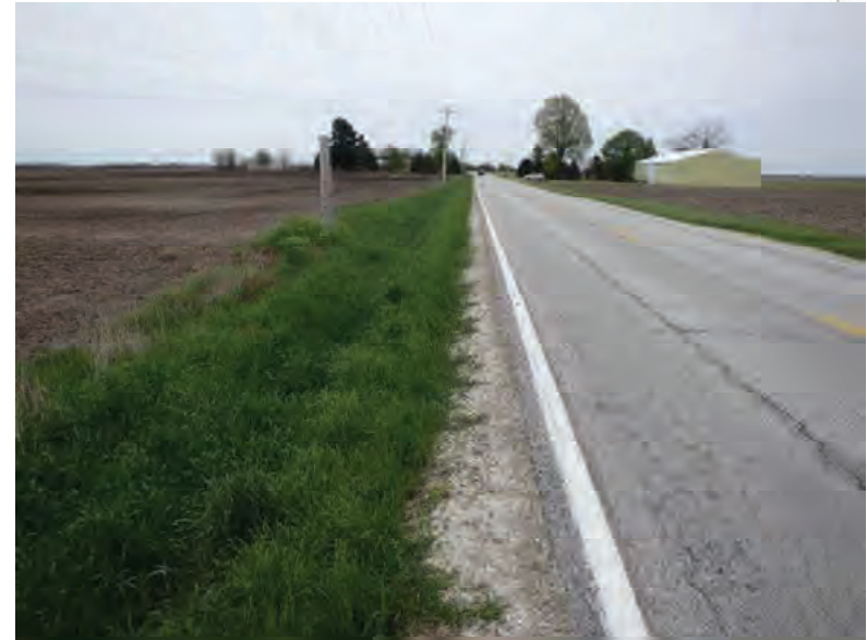
Picture 696: looking east along a roadside ditch on the north side of SR 26, 05/04/2020 (Exhibit 6AK)
