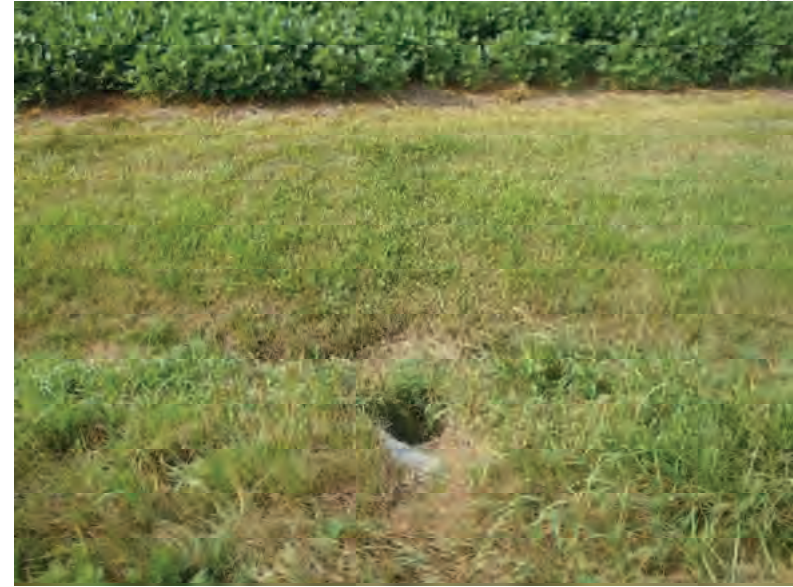
Picture 712: looking south at the mostly buried opening of CLV 026 86 19.79 and a roadside ditch on the south side of SR 26, east of N 725 E, 07/19/2019 (Exhibit 6AM)
