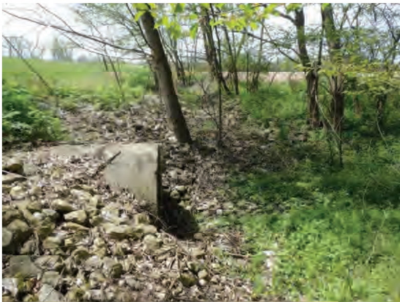
Picture 513: Looking west at the northern opening to the structure and riprapped roadside ditch leading to it, 05/04/2020 (Exhibit 6AB)
