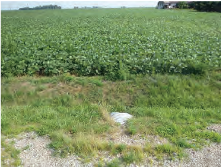
Picture 765: looking north at the opening of structure CLV 026 86 21.22 and a roadside ditch on the north side of SR 26, east of N 875 E, 07/19/2019 (Exhibit 6AQ)
