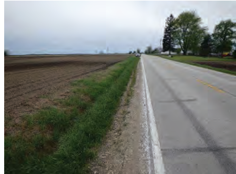
Picture 714: Looking west, towards N 725 E, along a roadside ditch on the south side of SR 26, 05/04/2020 (Exhibit 6AM)
