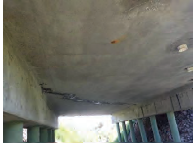
Picture 800: looking northeast, at the underneath side of the structure to document no evidence of bats or birds, 05/07/2020 (Exhibit 6AT)
