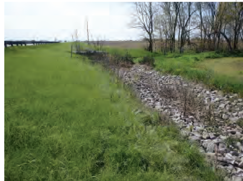
Picture 363: Looking west along roadside ditch leading to UNT4 to Big Pine Creek on the north side of SR 26, 05/01/2020 (Exhibit 6S)
