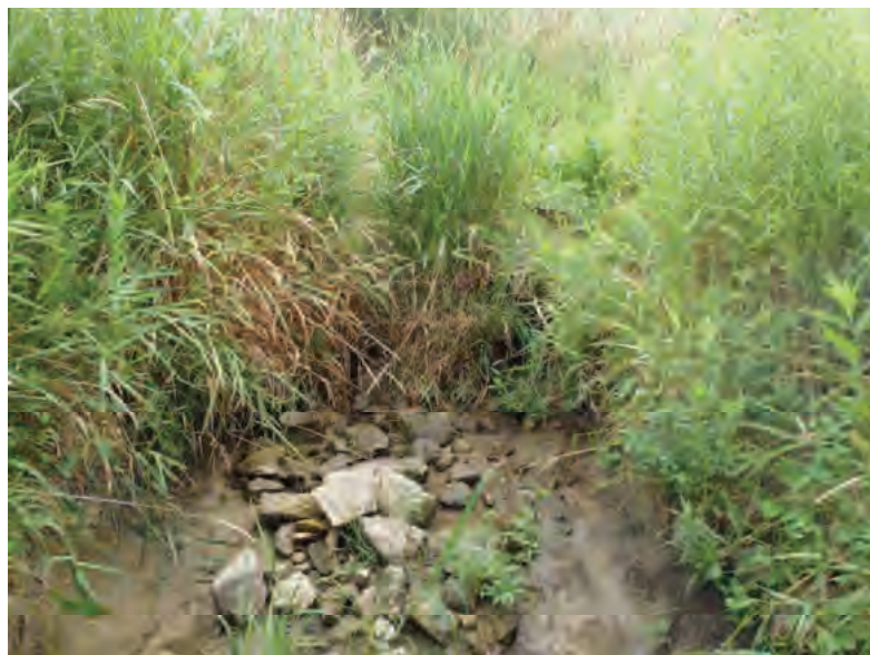
Picture 230: Looking northeast at the development of a headcut and bank instability, southwest of the structure opening, 07/16/2019 (Exhibit 6M)
