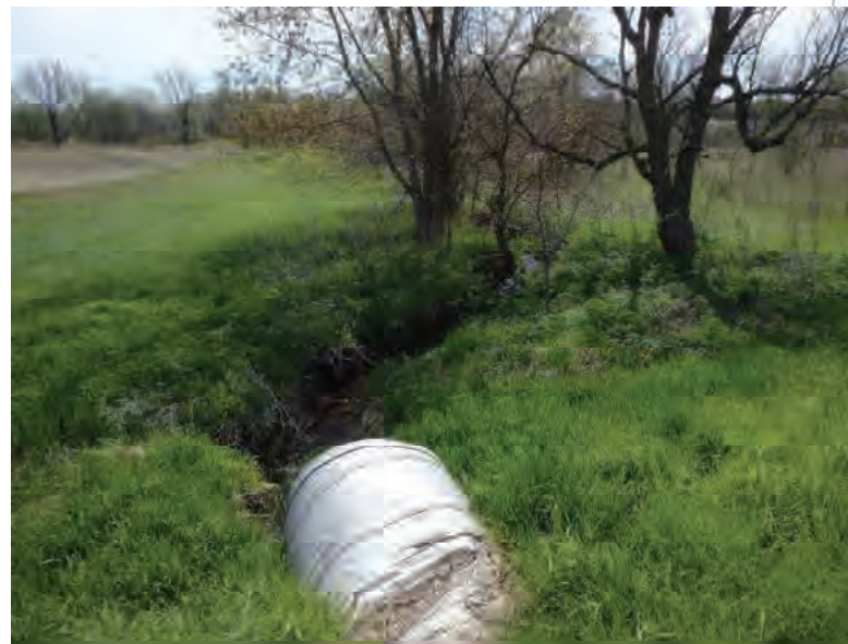
Picture 307: Looking south, downstream, along UNT2 to Big Pine Creek, from the top of structure CV 026 86 12.59, on the south side of SR 26, 05/01/2020 (Exhibit 6Q)
