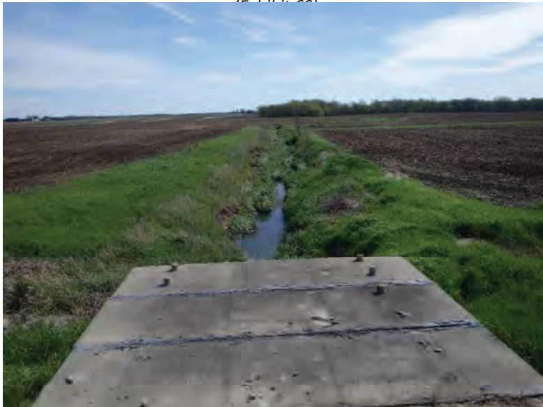
Picture 352: Looking south, downstream, at UNT4 to Big Pine Creek from the top of structure CV 026 86 13.10, on the south side of SR 26, 05/01/2020 (Exhibit 6S)
