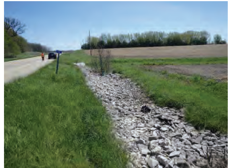
Picture 92: Looking east along a riprapped roadside ditch, on the south side of SR 26 and west of UNT3 to Mud Pine Creek, 05/01/2020 (Exhibit 6F)
