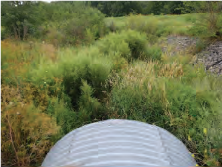
Picture 21: Looking S, downstream, at UNT1 to Mud Pine Creek from the top of the structure, on the south side of SR 26, 07/16/2019 (Exhibit 6A)
