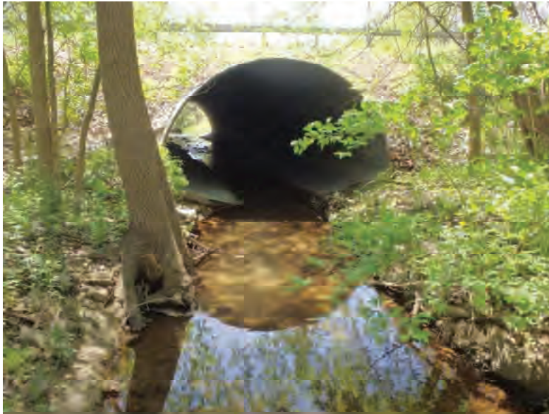
Picture 489: Looking south, downstream, along UNT6 to Big Pine Creek, at the north opening of the structure on the north side of SR 26, 05/04/2020 (Exhibit 6AA)
