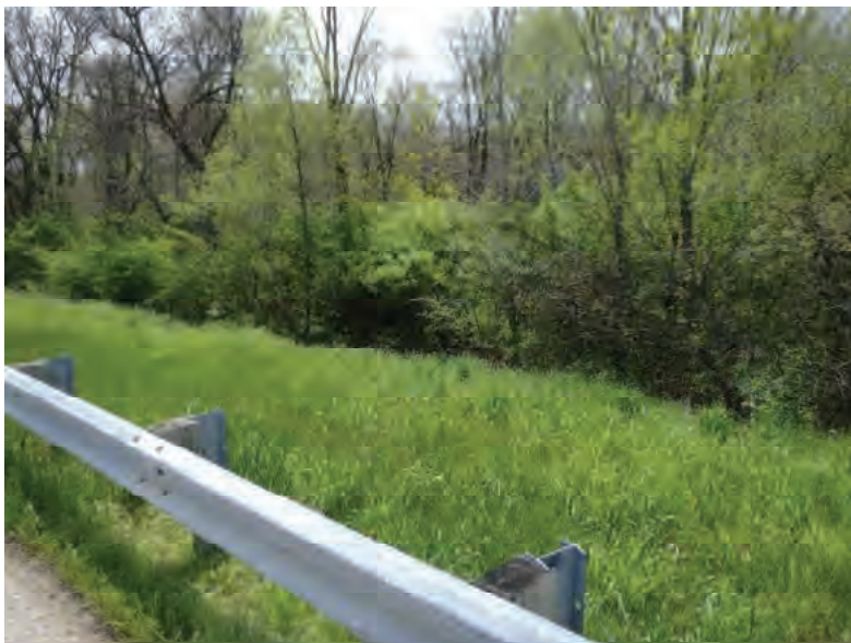
Picture 465: Looking south at a grassed slope, leading to the south opening of structure CV 026 86 15.00 on the south side of SR 26, 05/04/2020 (Exhibit 6Z)
