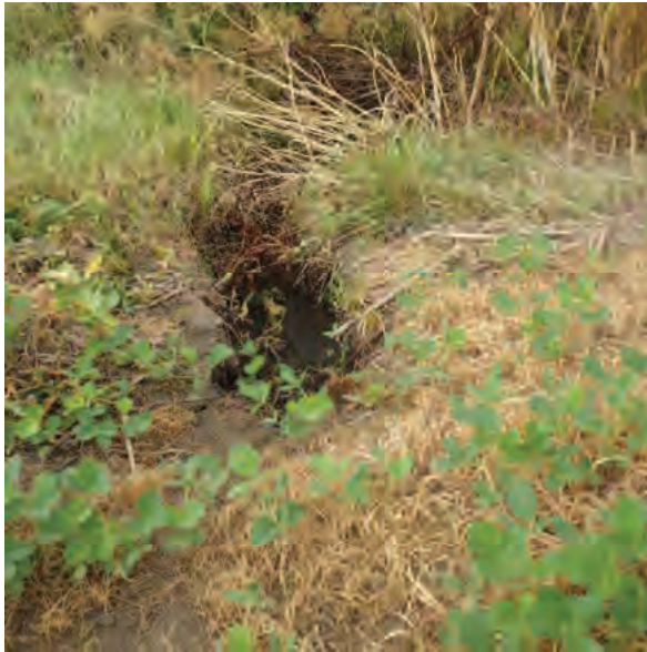
Picture 314: Looking south at headcut that formed adjacent to the northern opening of structure CV 026 86 12.59, 07/16/2019 (Exhibit 6Q)
