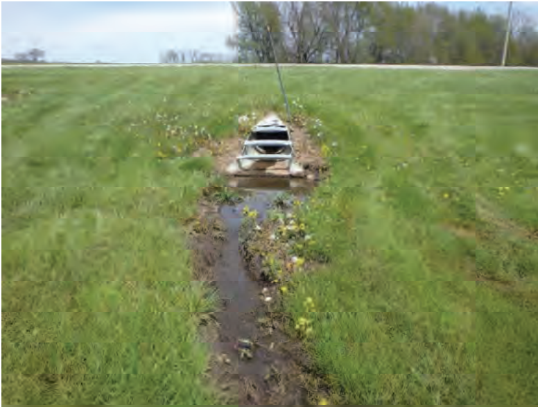
Picture 254: Looking northeast, upstream, at the start of Channel 2 and structure CLV 026 86 11.87, on the western side of SR 26, 05/01/2020 (Exhibit 6N)
