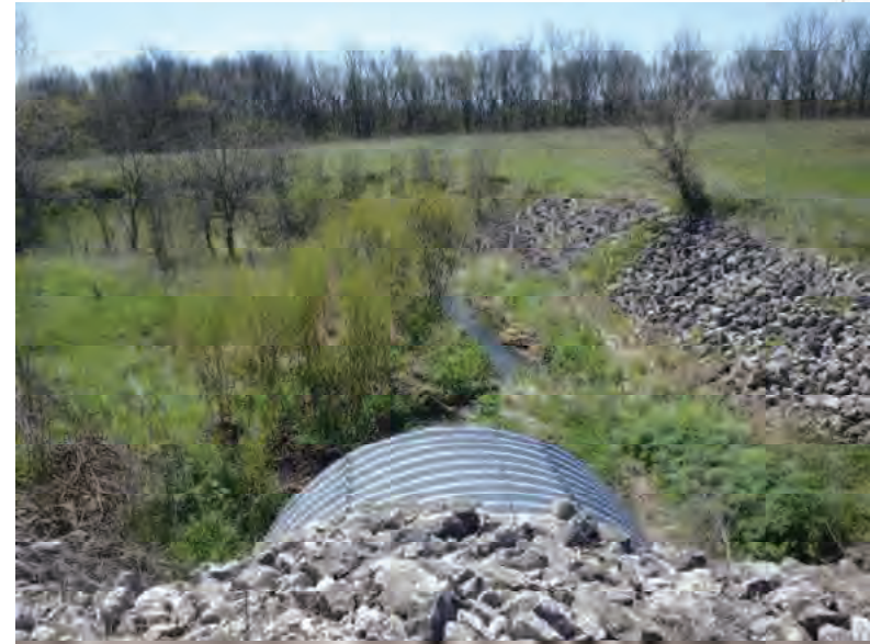
Picture 22: Looking S, downstream, at UNT1 to Mud Pine Creek from the top of the structure, on the south side of SR 26, 05/01/2020 (Exhibit 6A)
