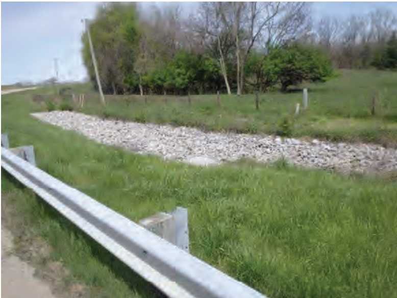
Picture 471: Looking north at a riprapped roadside ditch and structure CV 026 86 15.00 on the north side of SR 26, 05/04/2020 (Exhibit 6Z)
