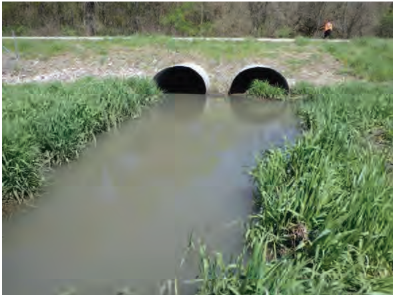
Picture 105: Looking north at Wetland 5 and the structure from the southern edge of Wetland 5, 05/01/2020 (Exhibit 6F)
