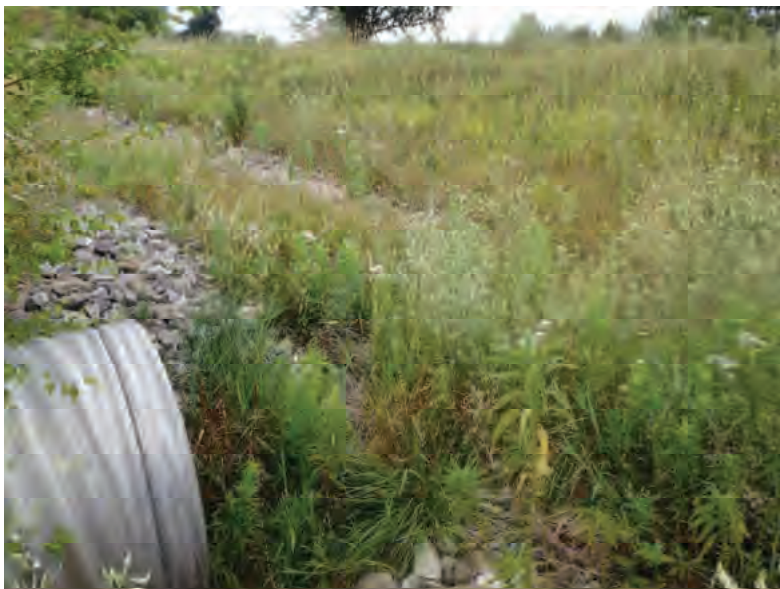
Picture 235: Looking northwest at the northeastern opening of structure CV 026 86 11.70, on the northeast side of SR 26, 07/16/2019 (Exhibit 6M)
