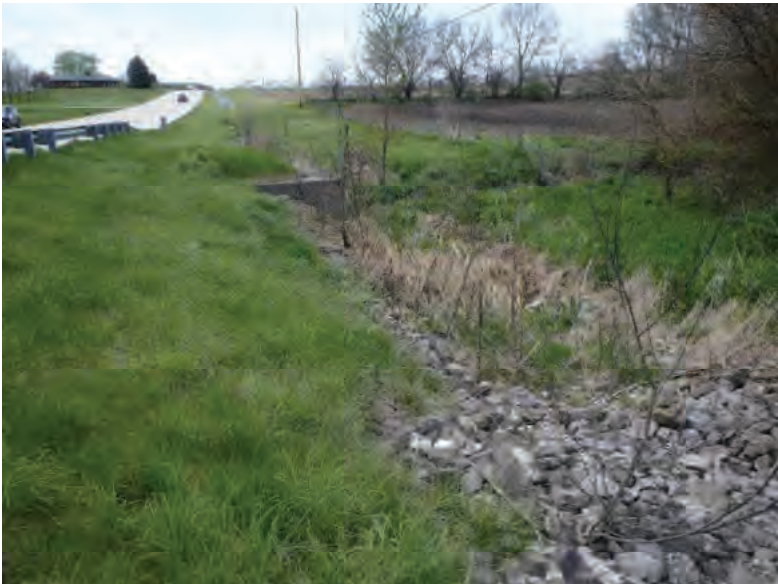
Picture 210: Looking west, towards UNT5 to Mud Pine Creek, along a riprapped roadside ditch on the north side of SR 26, 05/01/2020 (Exhibit 6K)
