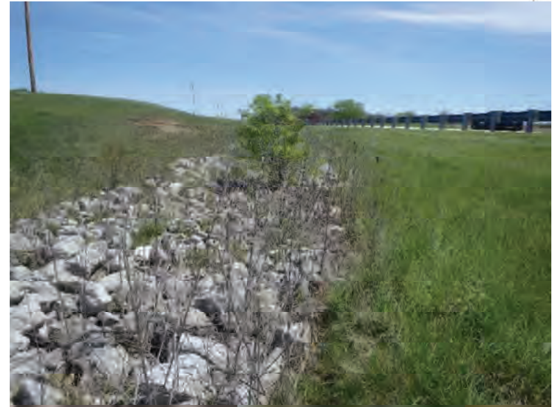
Picture 178: Looking east, east of UNT4 to Mud Pine Creek, along a roadside ditch on the north side of SR 26, 05/01/2020 (Exhibit 6J)
