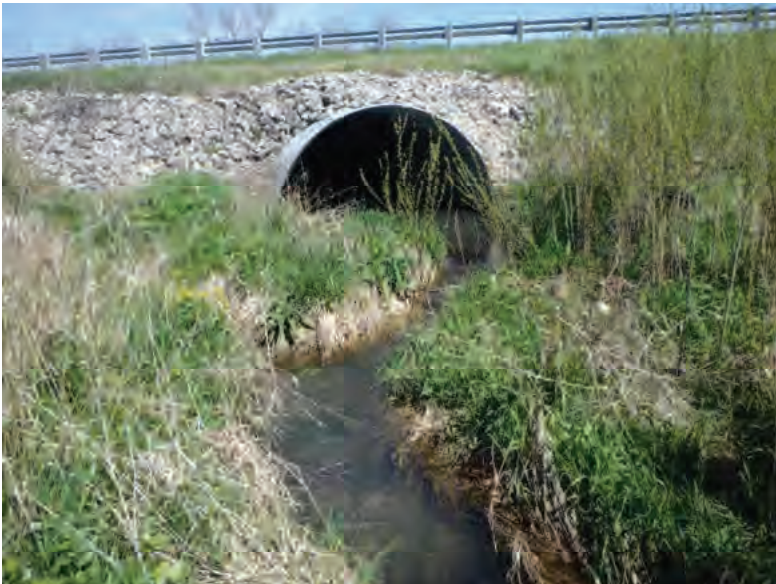
Picture 23: Looking N, upstream, at the southern opening of the structure and UNT1 to Mud Pine Creek, on the south side of SR 26, 05/01/2020 (Exhibit 6A)
