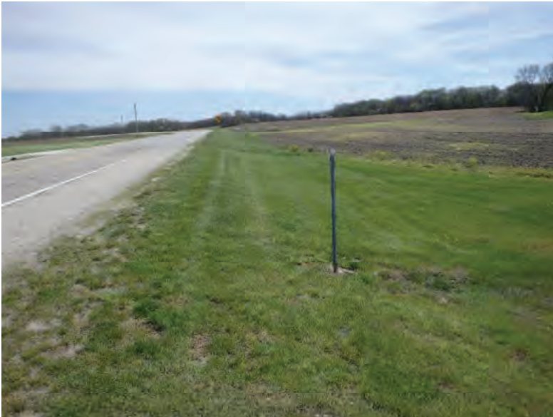
Picture 272: Looking southeast along grassy area on the west side of SR 26, adjacent to Wetland 14, 05/01/2020 (Exhibit 60)
