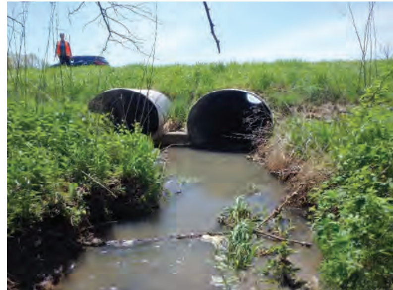
Picture 110: Looking south, downstream, from within UNT3 to Mud Pine Creek on the north side of SR 26, 05/01/2020 (Exhibit 6F)
