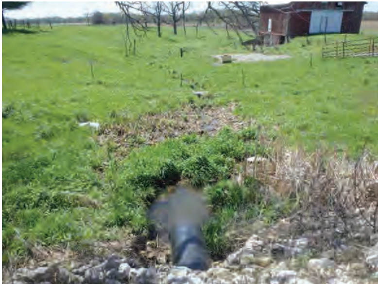
Picture 71: Looking south at Wetland 7, located on the south side of SR 26, adjacent to the south opening of structure CLV 026 86 9.60, 05/01/2020 (Exhibit 6E)
