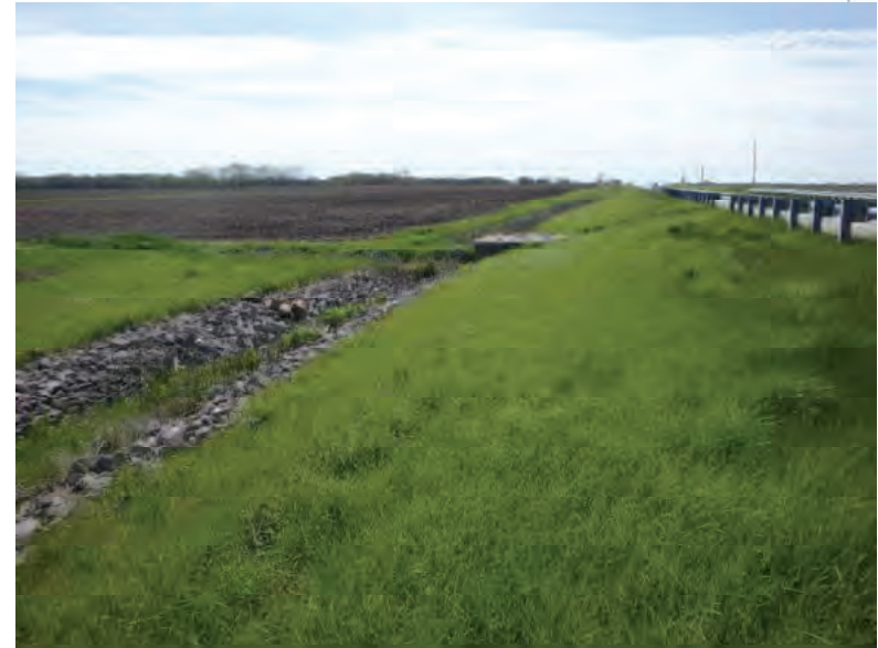
Picture 355: Looking west, along a riprapped roadside ditch leading to UNT4 to Big Pine Creek, on the south side of SR 26, 05/01/2020 (Exhibit 6S)
