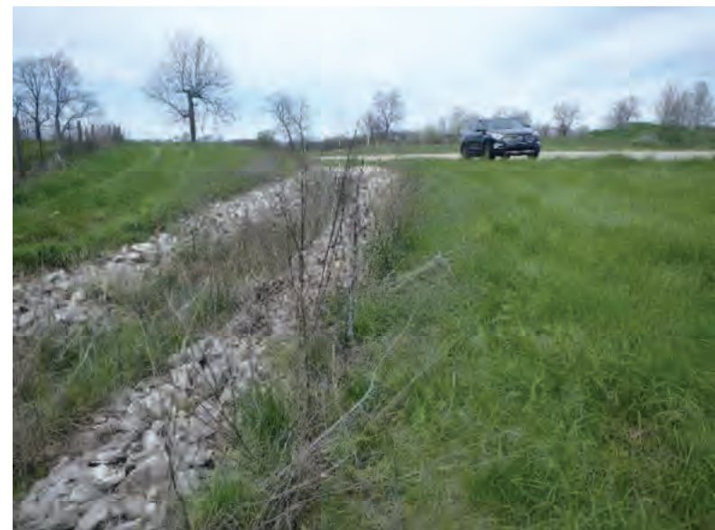
Picture 223: Looking northwest along a riprapped roadside ditch on the west side of SR 26, north of UNT6 to Mud Pine Creek, 05/01/2020 (Exhibit 6M)
