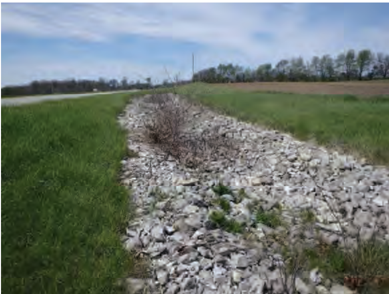
Picture 256: Looking northwest along riprapped roadside ditch on the east side of SR 26, northwest of Channel 3, 05/01/2020 (Exhibit 6O)
