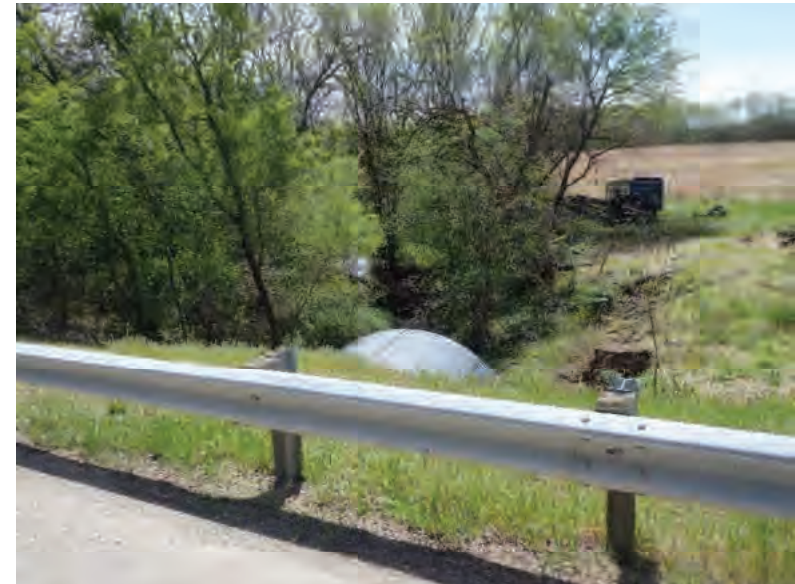
Picture 492: Looking south, downstream, at the southern opening of the structure and UNT6 to Big Pine Creek from the south edge of SR 26, 05/04/2020 (Exhibit 6AA)
