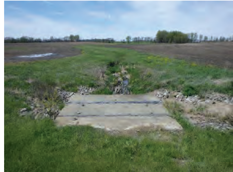
Picture 285: Looking north at the grassed waterway that precedes UNT1 to Big Pine Creek, from the top of structure CV 026 86 12.45 on the north side of SR 26, 05/01/2020 (Exhibit 6Q)
