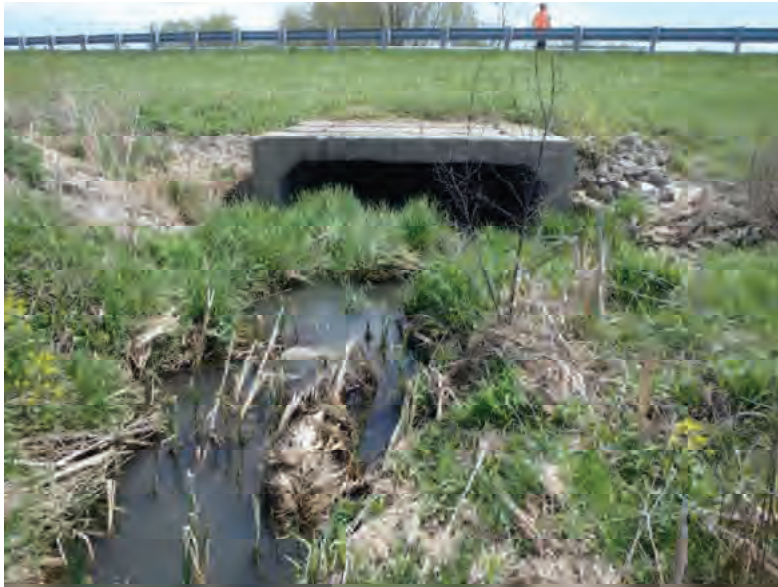
Picture 286: Looking south, from within the heavily deteriorating grassed waterway that precedes UNT1 to Big Pine Creek on the north side of SR 26; no OHWM or defined bed and bank, 05/01/2020 (Exhibit 6Q)
