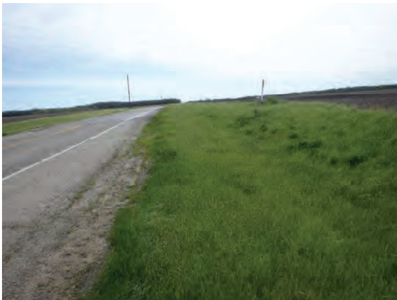
Picture 366: Looking east along roadside ditch, east of UNT4 to Big Pine Creek, on the south side of SR 26, 05/04/2020 (Exhibit 6T)
