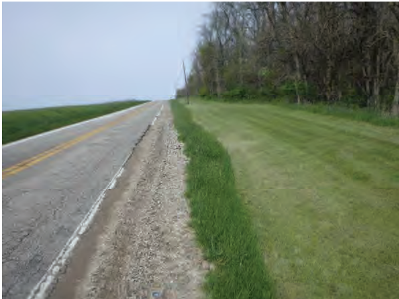
Picture 388: Looking west along a roadside ditch on the north side of SR 26, just west of N 200 E, 05/04/2020 (Exhibit 6V)
