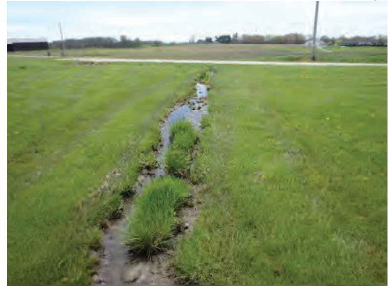
Picture 255: Looking southwest, downstream, along Channel 2, on the western side of SR 26, 05/01/2020 (Exhibit 6N)
