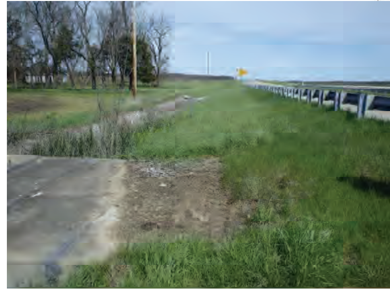
Picture 359: Looking east from the corner of the structure at roadside ditch on the north side of SR 26, 05/01/2020 (Exhibit 6S)
