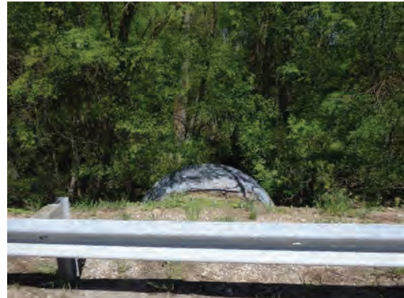
Picture 488: Looking north at the northern opening of structure CV 026 86 15.15, from the edge of the road on the north side of SR 26, 05/04/2020 (Exhibit 6AA)
