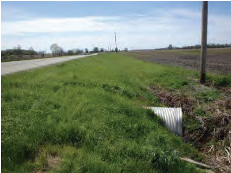
Picture 316: Looking west at the northern opening of the structure, along a grassed slope, on the northern side of SR 26, 05/01/2020 (Exhibit 6Q)
