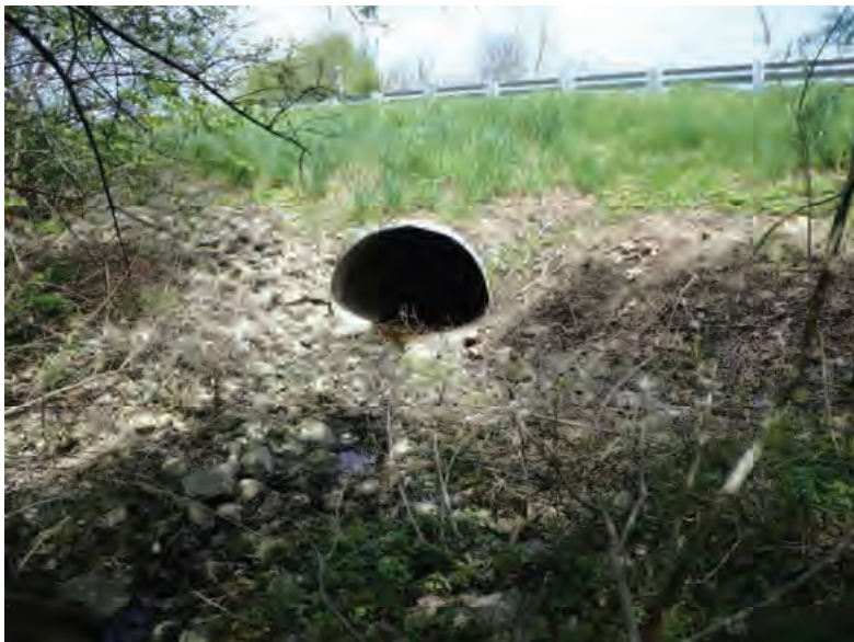
Picture 467: Looking north, at the south opening of the structure on the south side of SR 26, 05/04/2020 (Exhibit 6Z)
