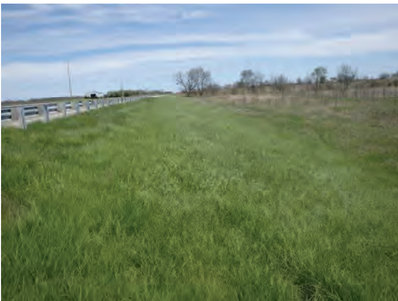
Picture 300: Looking east at grassed slope on the south side of SR 26, east of UNT1 to Big Pine Creek, 05/01/2020 (Exhibit 6Q)
