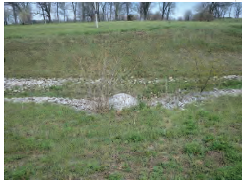
Picture 236: Looking northeast at the structure with no channel beyond the culvert and riprapped roadside ditches leading to it on the northeast side of SR 26, 05/01/2020 (Exhibit 6M)
