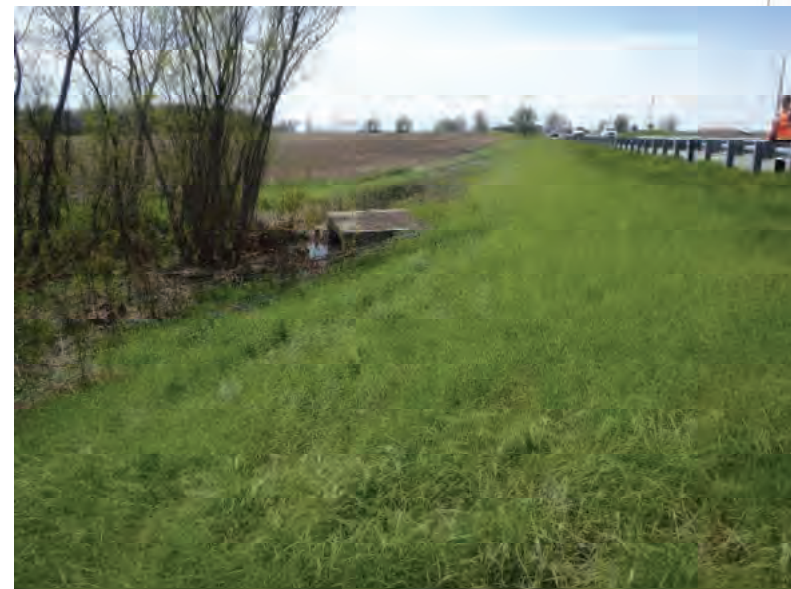
Picture 299: Looking west towards UNT1 to Big Pine Creek on the south side of SR 26, 05/01/2020 (Exhibit 6Q)
