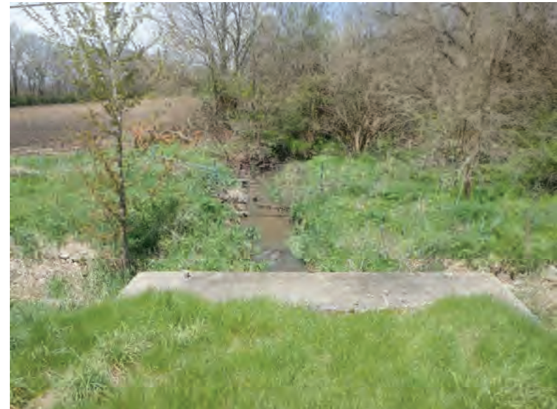
Picture 207: Looking north, upstream, along UNT5 to Mud Pine Creek from the top of the structure, on the north side of SR 26, 05/01/2020 (Exhibit 6K)
