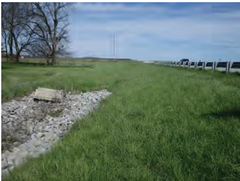
Picture 364: Looking east along roadside ditch, east of UNT4 to Big Pine Creek, on the north side of SR 126, 05/01/2020 (Exhibit 6S)
