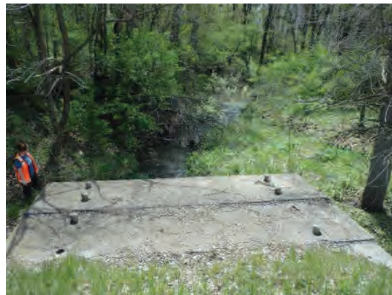
Picture 200: Looking south, downstream, along UNT5 to Mud Pine Creek, from the top of the structure, on the south side of SR 26, 05/01/2020 (Exhibit 6K)
