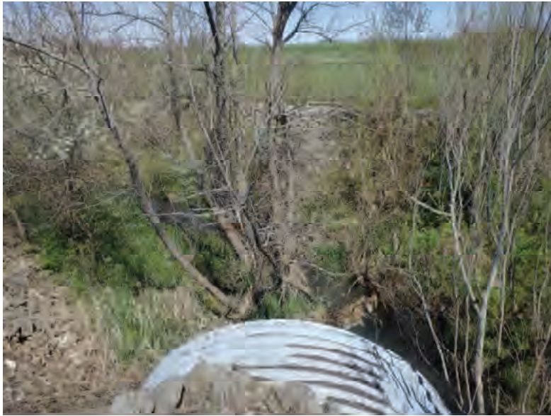
Picture 25: Looking N, upstream, at UNT1 to Mud Pine Creek from the top of the structure, on the north side of SR 26, 05/01/2020 (Exhibit 6A)
