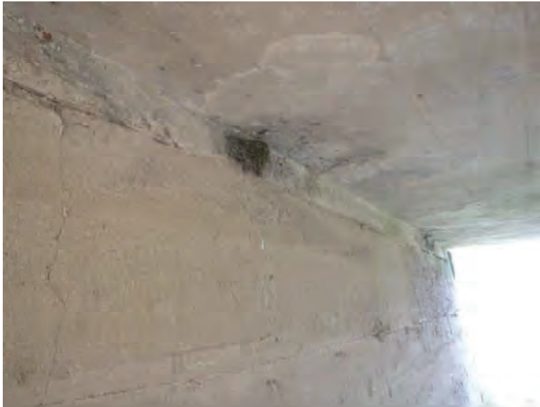
Picture 417: Looking north, through the structure, at a nest on the west wall, 05/04/2020 (Exhibit 6W)
