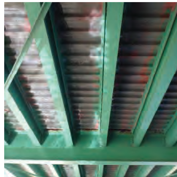
Picture 52: Looking at the underneath side of the historic pony truss bridge to show no evidence of bats, 05/01/2020 (Exhibit 6C)
