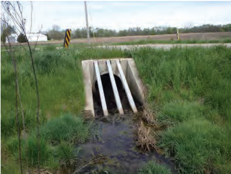
Picture 427: Looking northwest at Channel 4 and the opening of structure CLV 026 86 14.46, on the south side of SR 26, 05/04/2020 (Exhibit 6X)
