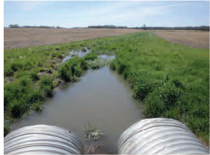
Picture 104: Looking south at Wetland 5 from the top of the structure, located on the south side of SR 26, 05/01/2020 (Exhibit 6F)
