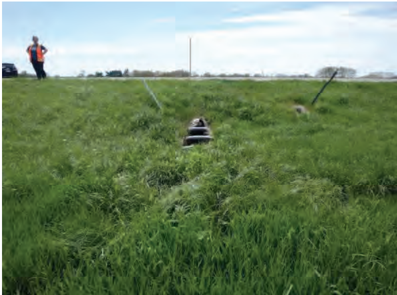
Picture 248: Looking southwest at the eastern opening of structure CLV 026 86 11.87, adjacent to Wetland 34, 05/01/2020 (Exhibit 6N)
