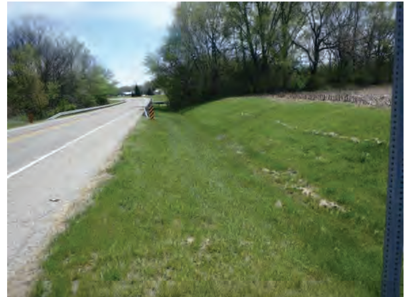
Picture 476: Looking east along a roadside ditch on the south side of SR 26, east of E Blvd and west of UNT6 to Big Pine Creek, 05/04/2020 (Exhibit 6Z)
