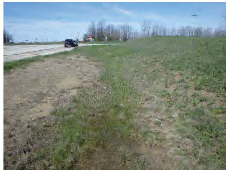
Picture 8: Looking west at roadside ditch, on the north side of SR 26, towards US-41, 05/01/2020 (Exhibit 6A)
