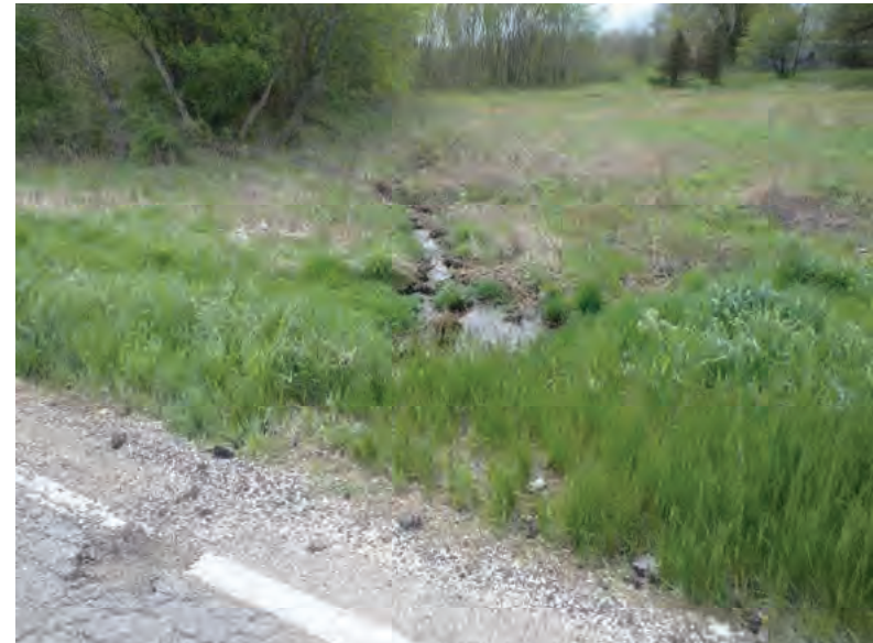
Picture 424: Looking southeast, downstream, at Channel 4 and the south opening of structure CLV 026 86 14.46, on the south side of SR 26, 05/04/2020 (Exhibit 6X)
