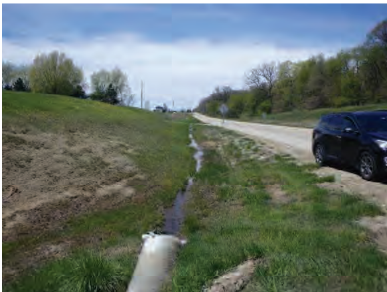
Picture 121: Looking west at a roadside ditch on the south side of SR 26, adjacent to the intersection of SR 26 and N 125 W, 05/01/2020 (Exhibit 6G)
