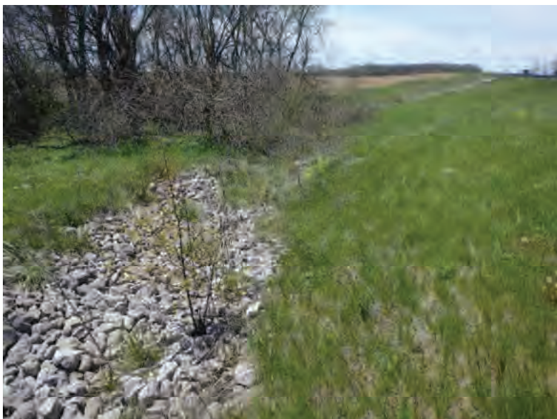
Picture 175: Looking west, towards UNT4 to Mud Pine Creek, along a roadside ditch on the south side of SR 26, 05/01/2020 (Exhibit 6J)
