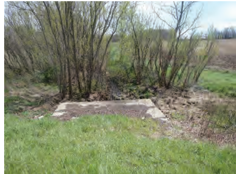
Picture 289: Looking south, downstream, at UNT1 to Big Pine Creek and the top of structure CV 026 86 12.45, on the south side of SR 26, 05/01/2020 (Exhibit 6Q)
