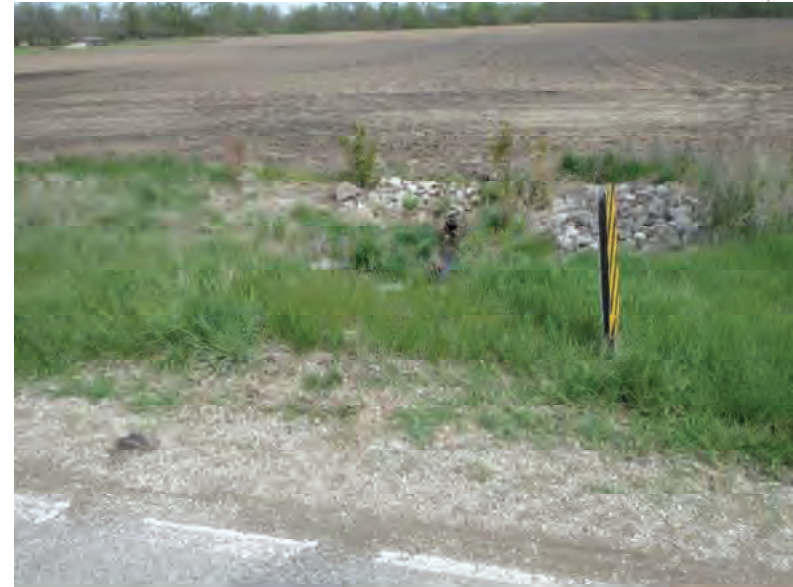
Picture 430: Looking north, upstream at the start of Channel 4 and the north opening of structure CLV 026 86 14.46, on the north side of SR 26; no channel present, 05/04/2020 (Exhibit 6X)
