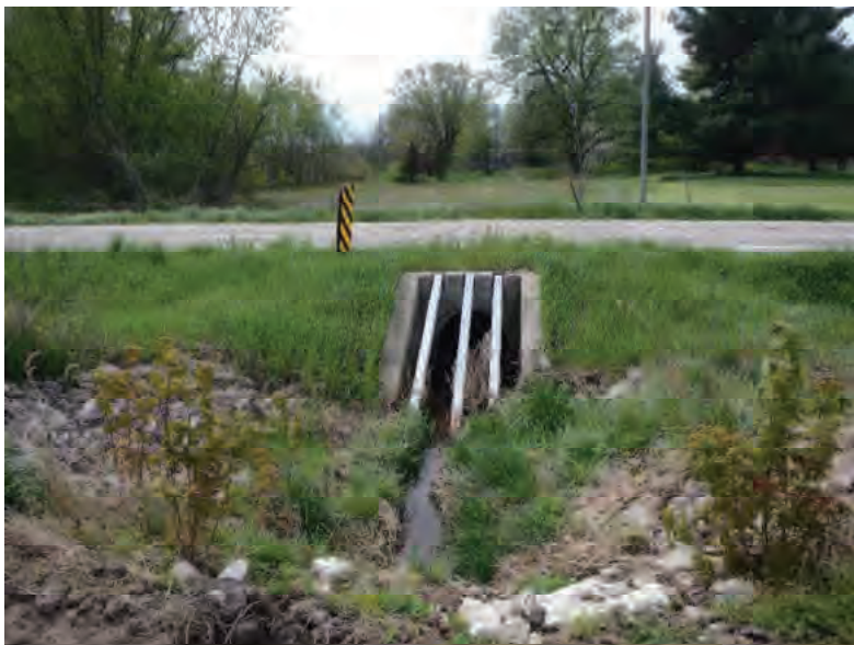
Picture 433: Looking south, downstream, at the start of Channel 4 and the north opening of the structure on the north side of SR 26, 05/04/2020 (Exhibit 6X)
