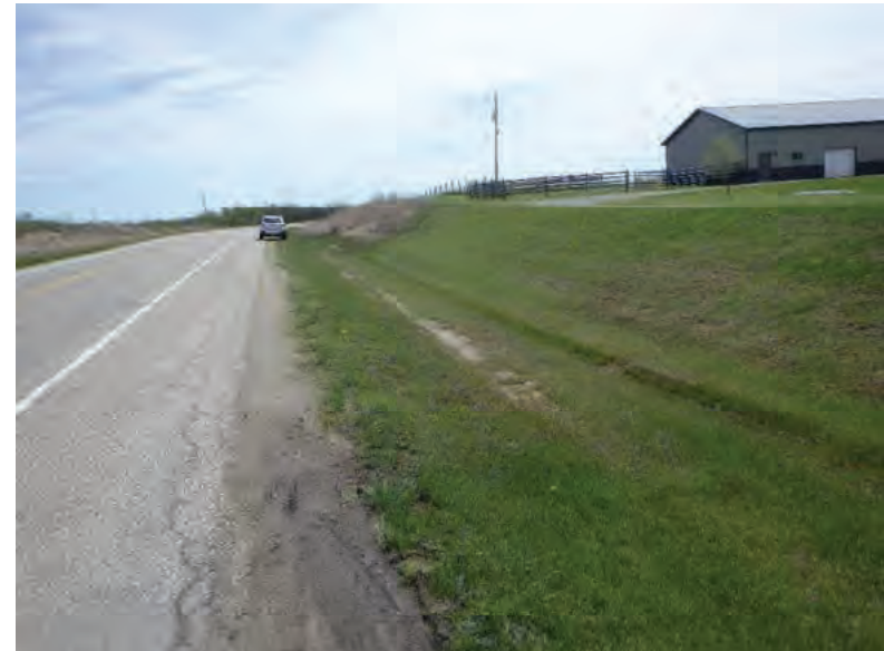
Picture 440: Looking east along a roadside ditch on the south side of SR 26, east of Channel 4 and west of Wetland 20, 05/04/2020 (Exhibit 6X)
