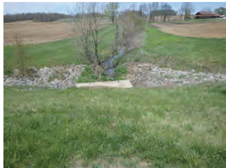
Picture 172: Looking north, upstream, at the structure and UNT4 to Mud Pine Creek from the north edge of SR 26, 05/01/2020 (Exhibit 6J)
