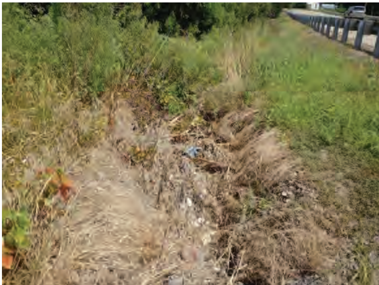
Picture 479: Looking east at a roadside ditch on the north side of SR 26 that leads to Wetland 22, 08/19/2019 (Exhibit 6AA)
