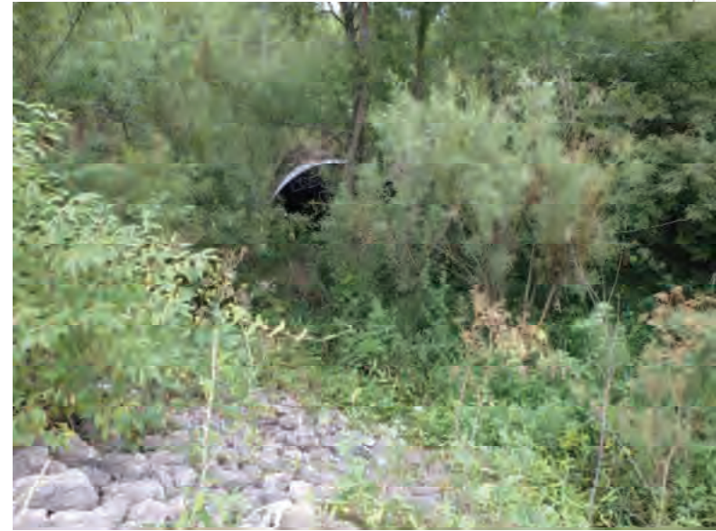
Picture 26: Looking S at the northern opening of the structure, located at the edge of a farm field on the north side of SR 26, 07/16/2019 (Exhibit 6A)
