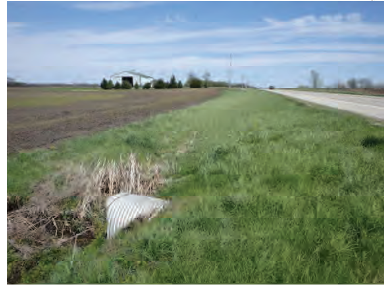
Picture 315: Looking east at the northern opening of the structure, along a grassed slope, on the northern side of SR 26, 05/01/2020 (Exhibit 6Q)
