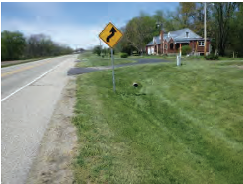
Picture 477: Looking west along a roadside ditch on the north side of SR 26, east of E Blvd and west of UNT6 to Big Pine Creek, 05/04/2020 (Exhibit 6Z)
