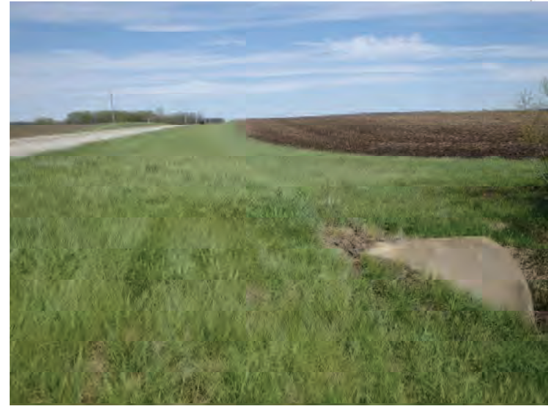
Picture 319: Looking east at the southern opening of the structure, along a grassed slope, on the south side of SR 26, 05/01/2020 (Exhibit 6R)
