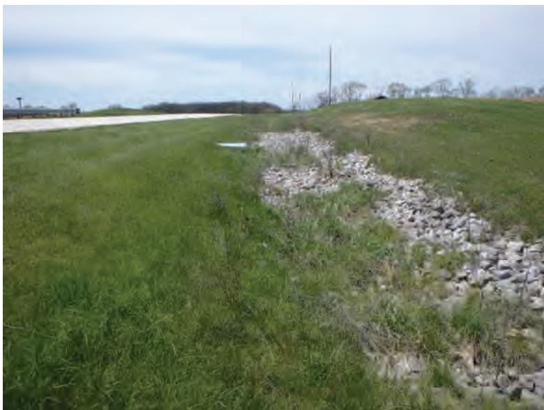
Picture 163: Looking west along a roadside ditch on the north side of SR 26, west of UNT4 to Mud Pine Creek 05/01/2020 (Exhibit 6J)
