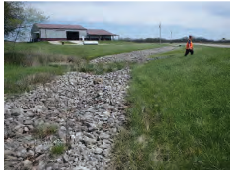
Picture 257: Looking southeast along riprapped roadside ditch on the east side of SR 26, towards Channel 3, 05/01/2020 (Exhibit 6O)
