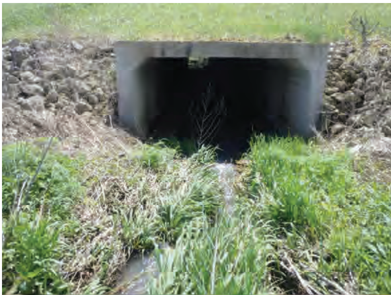
Picture 173: Looking south, downstream, at UNT4 to Mud Pine Creek and the north opening of the structure on the north side of SR 26, 05/01/2020 (Exhibit 6J)
