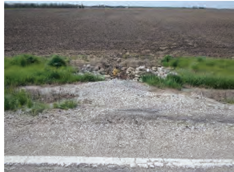
Picture 381: Looking south at south opening of structure CLV 026 86 13.69 from southern edge of the road, 05/04/2020 (Exhibit 6U)
