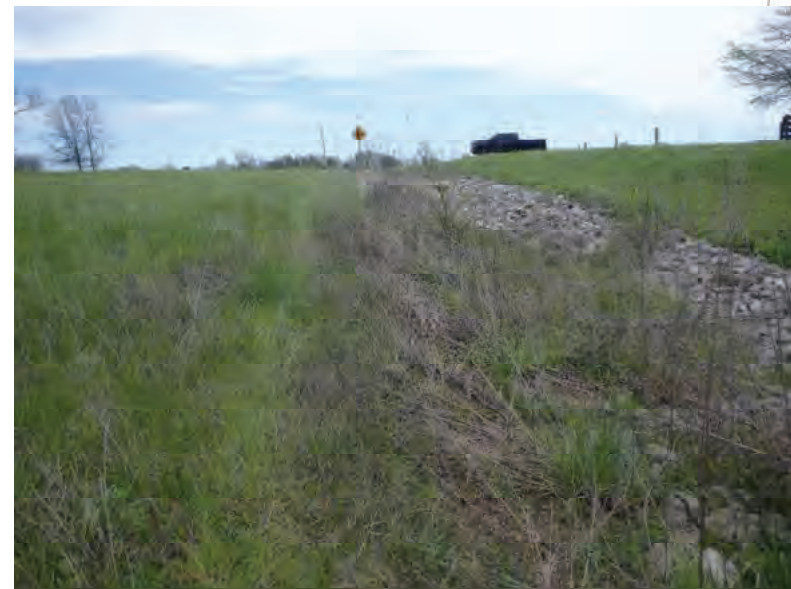
Picture 232: Looking southeast, away from UNT6 to Mud Pine Creek, along a riprapped roadside ditch on the west side of SR 26, 05/01/2020 (Exhibit 6M)
