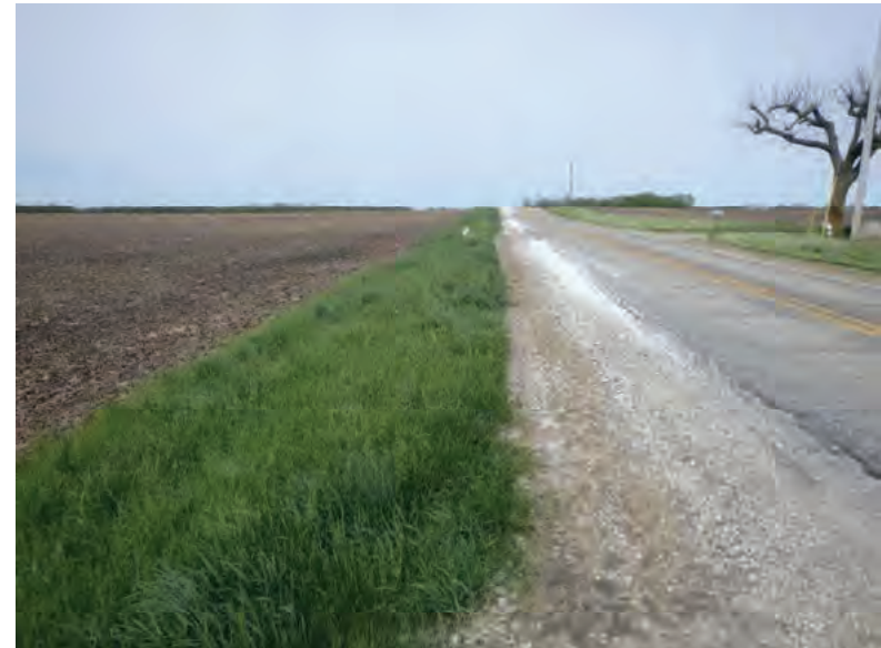
Picture 377: Looking west along roadside ditch on the south side of SR 26, west of N 175 E, 05/04/2020 (Exhibit 6T)
