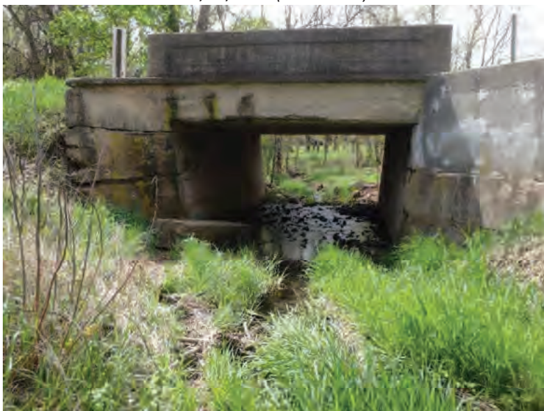
Picture 411: Looking south, downstream, along UNT5 to Big Pine Creek, at the north side of the structure, on the north side of SR 26, 05/04/2020 (Exhibit 6W)
