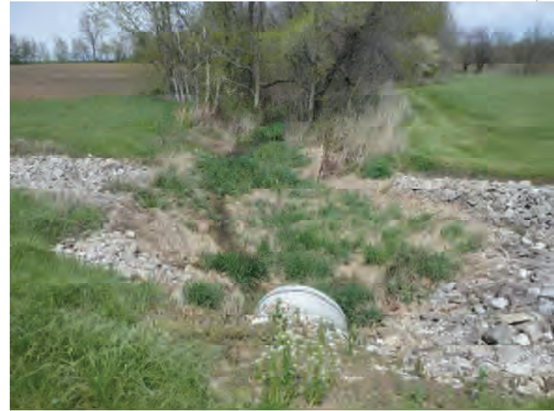
Picture 259: Looking northeast, upstream, at Channel 3, Wetland 36, and structure CV 026 86 12.10, on the east side of SR 26, 05/01/2020 (Exhibit 60)
