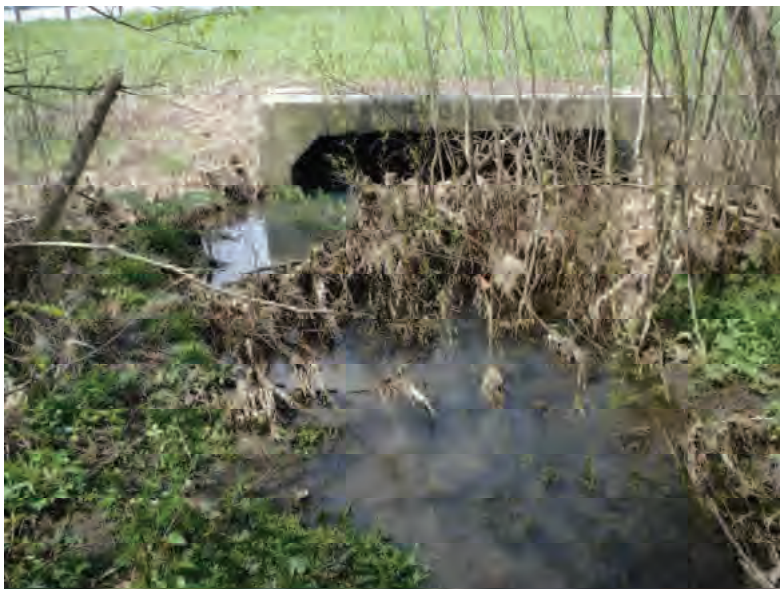
Picture 290: Looking north, upstream, along UNT1 to Big Pine Creek, on the south side of SR 26, 05/01/2020 (Exhibit 6Q)
