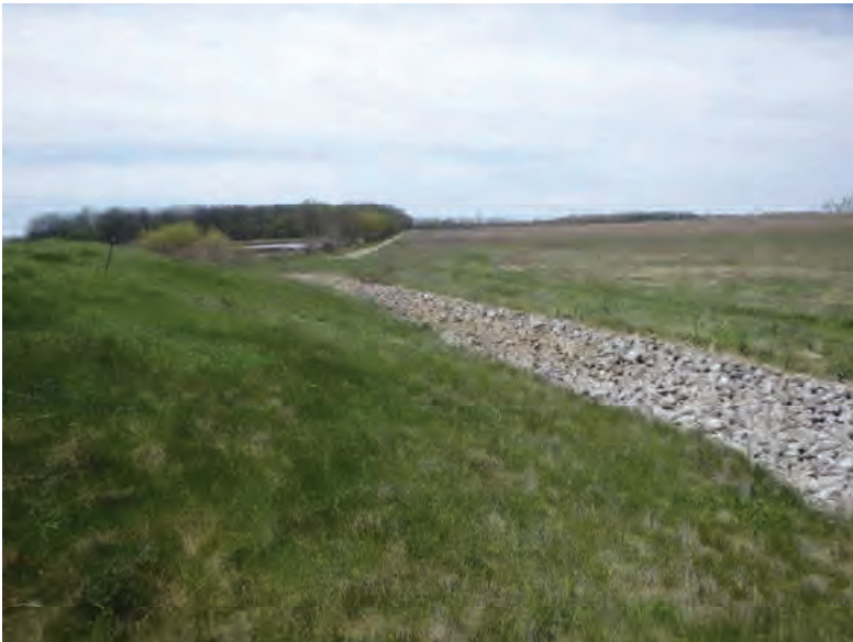
Picture 159: Looking west along a roadside ditch towards Wetland 10, on the north side of SR 26, 05/01/2020 (Exhibit 6I)
