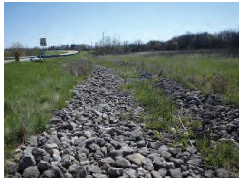
Picture 20: Looking east at riprapped roadside ditch on the south side of SR 26, leading to UNT1 to Mud Pine Creek, 05/01/2020 (Exhibit 6A)
