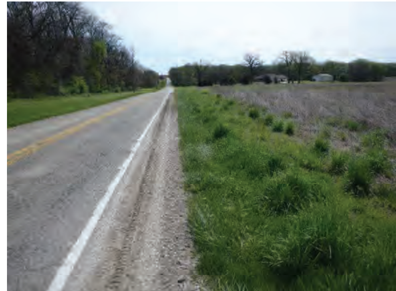
Picture 385: Looking east along the south side of SR 26, east of N 175 E 05/04/2020 (Exhibit 6V)
