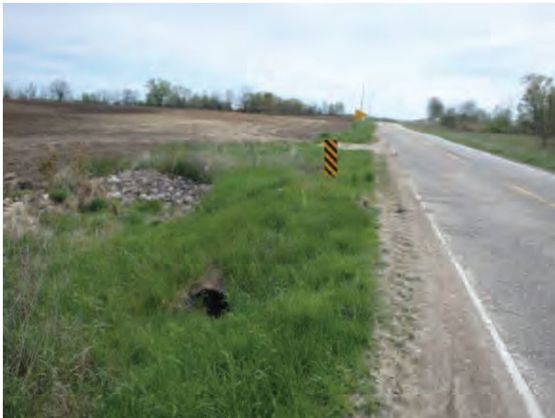
Picture 431: Looking east towards Channel 4 and the north opening of the structure along a roadside ditch on the north side of SR 26, 05/04/2020 (Exhibit 6X)
