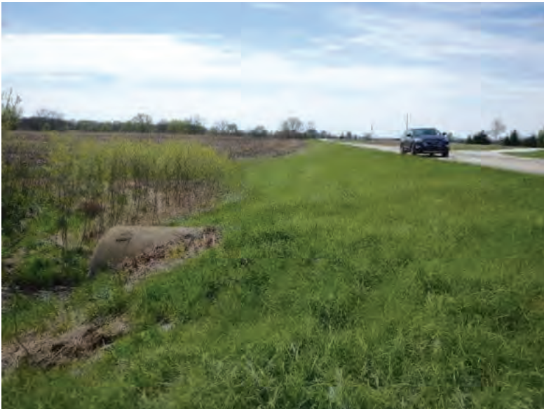
Picture 320: Looking west at the southern opening of the structure, along a grassed slope, on the south side of SR 26, 05/01/2020 (Exhibit 6R)
