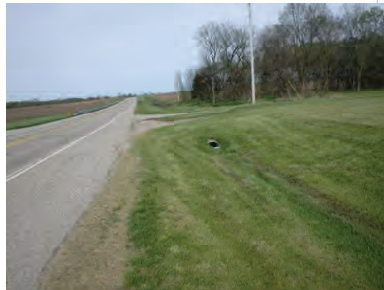
Picture 367: Looking west along roadside ditch, east of UNT4 to Big Pine Creek, on the north side of SR 26, 05/04/2020 (Exhibit 6S and Exhibit 6T)
