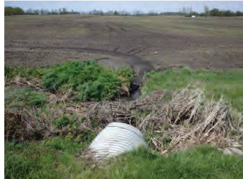
Picture 313: Looking north at the northern opening of structure CV 026 86 12.59, and flow patterns in the field (no OHWM or defined bed and bank), on the north side of SR 26, 05/01/2020 (Exhibit 6Q)
