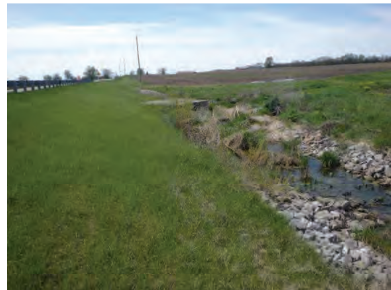
Picture 301: Looking west towards UNT1 to Big Pine Creek along a riprapped roadside ditch on the north side of SR 26, 05/01/2020 (Exhibit 6Q)
