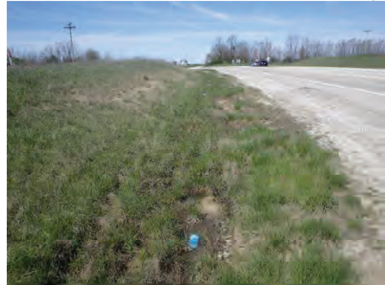
Picture 10: Looking west at roadside ditch on the south side of SR 26, towards US-41, 05/01/2020 (Exhibit 6A)
