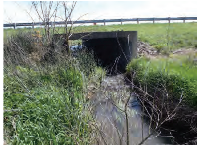
Picture 361: Looking south, downstream, along UNT4 to Big Pine Creek on the north side of SR 26, 05/01/2020 (Exhibit 6S)
