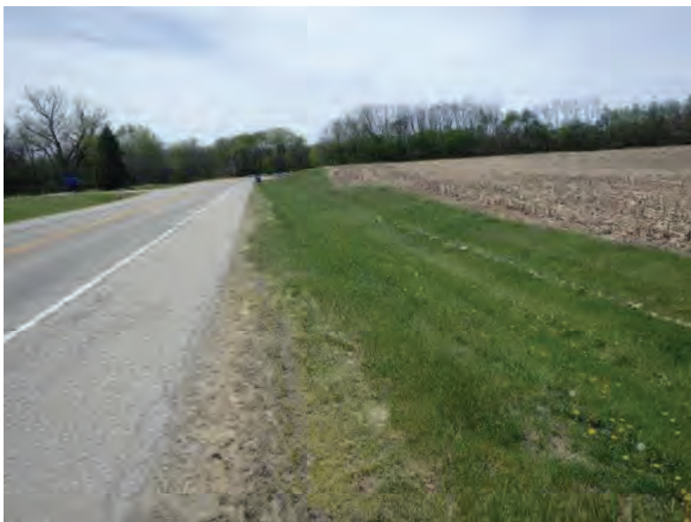
Picture 499: Looking southwest along a roadside ditch on the north side of SR 26, 05/04/2020 (Exhibit 6AA)
