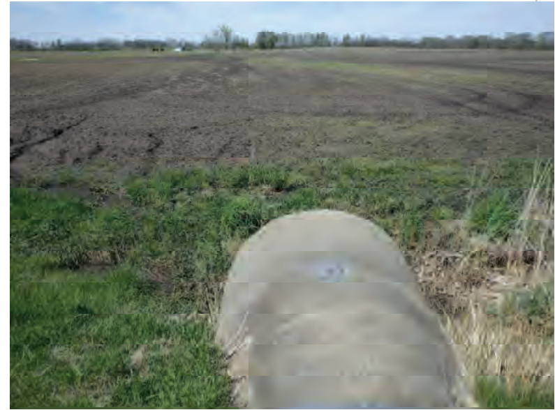
Picture 331: Looking north from the top of the northern opening of structure CV 026 86 12.70, on the north side of SR 26; no defined channel observed, 05/01/2020 (Exhibit 6R)
