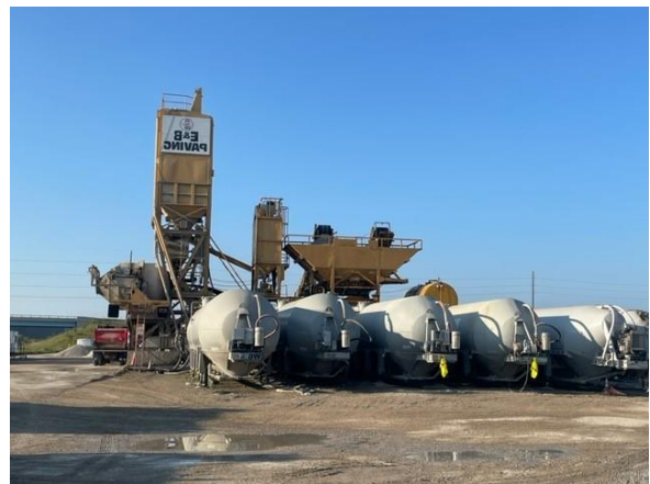
Figure 4-1 Central Mix Plant
