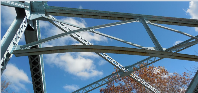
Replace Bent Upper Bracing
