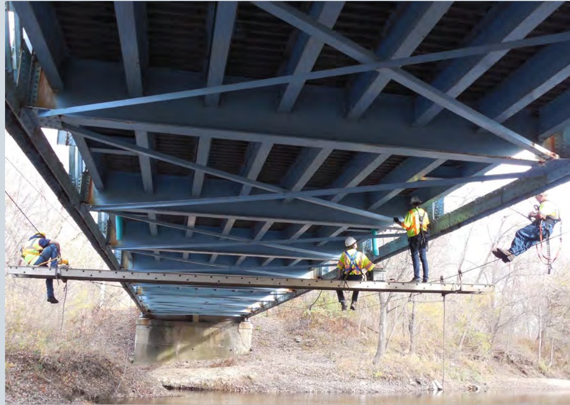
Replace 5 of 8 Substandard Stringers
