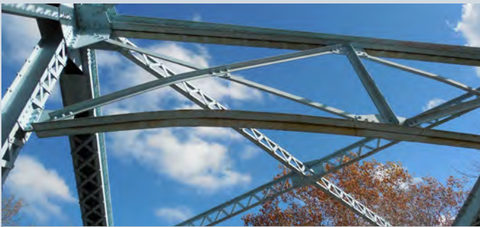
Replace Bent Upper Bracing
