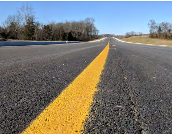
INDOT employees filling roadway cracks (at top as part of INDOT’s highway maintenance program. U.S. 50 near North Vernon, Indiana (above).
