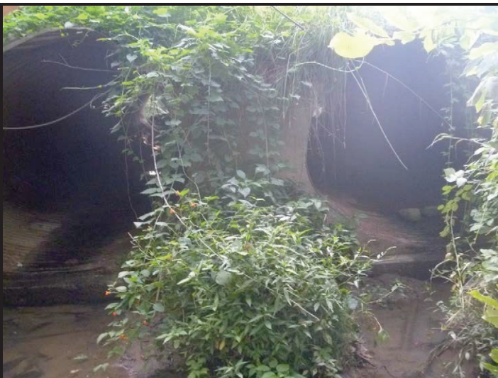
Photo 5 – Outlet at SR 159 over UNT to Splunge Creek: Facing upstream to the west toward the outlet of Str. No. CV 159-084-23.30, from east of SR 159.
