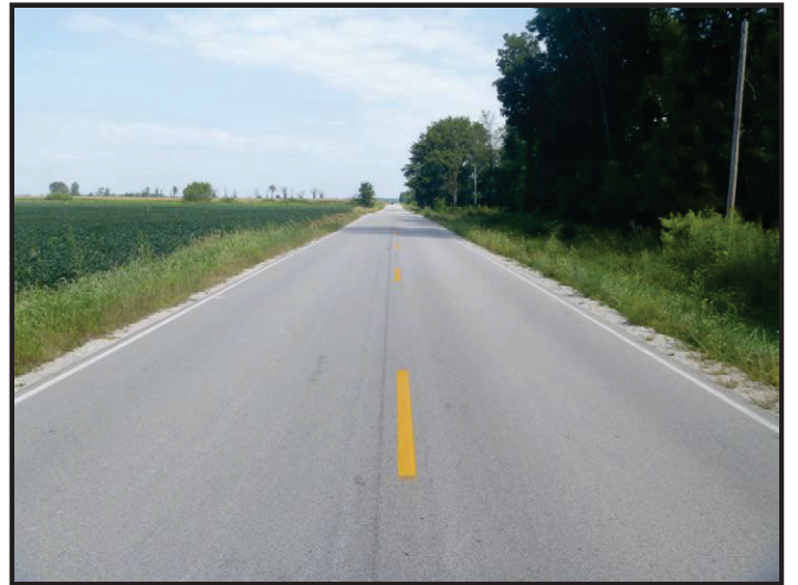
Photo 16 – SR 159 Project Setting, North of Culvert: Facing north toward the northern limits of the project.
