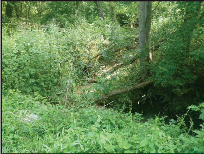
Photo 9 – SR 159 Crossing of UNT to Splunge Creek: Facing downstream to the east along UNT to Splunge Creek from the top of the SR 159 small structure. The left pipe flows freely, but the right pipe outfalls into a scour hole.
