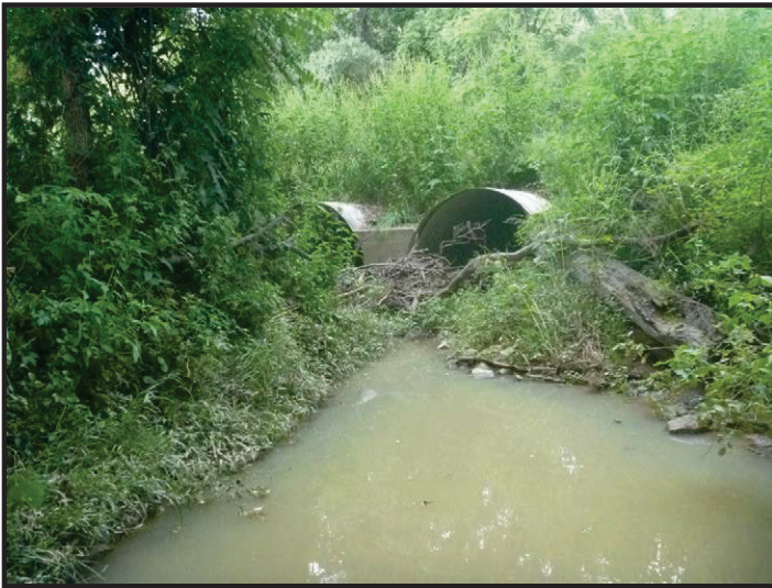
Photo 1 – Inlet at SR 159 over UNT to Splunge Creek: Facing northeast toward inlet of SR 159 small structure, Str. No. CV 159-084-23.30, a set of twin elliptical 47-foot-long steel pipes, each 8.5 feet wide and 6 feet high.
