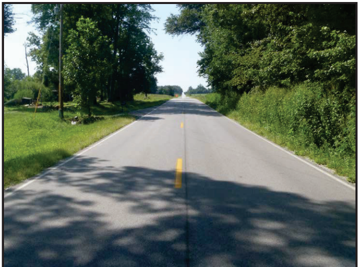
Photo 12 – SR 159 Project Area, South of Culvert: Facing south along SR 159 toward the southern limits of the project area.
