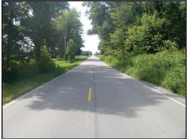
Photo 10 – SR 159 Crossing of UNT to Splunge Creek: Facing south along SR 159 from the top of the small structure at Splunge Creek. Topography is flat and land use is forested, and rural residential.
