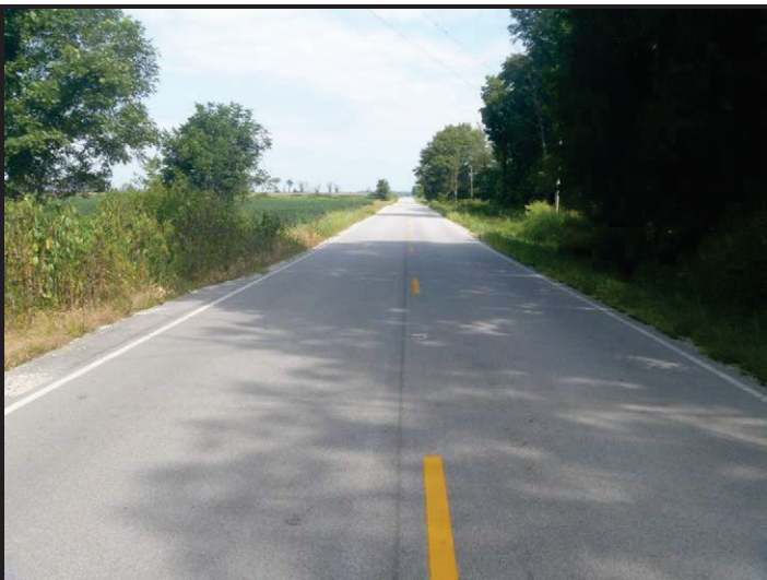
Photo 11 – SR 159 Crossing of UNT to Splunge Creek: Facing north along SR 159 from the top of the small structure at Splunge Creek. Topography is flat and land use is forested, agricultural, and rural residential.
