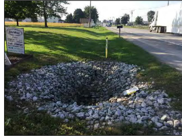
2. View of culvert located within the project area, on the west side of SR 5, looking south.
