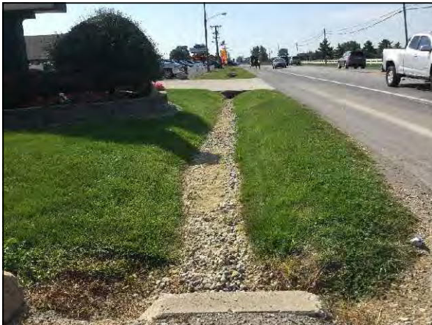
19. View of culvert on the east side of SR 5, looking south within project area.
