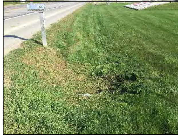
6. View of culvert on the east side of SR 5, looking north within the project area.
