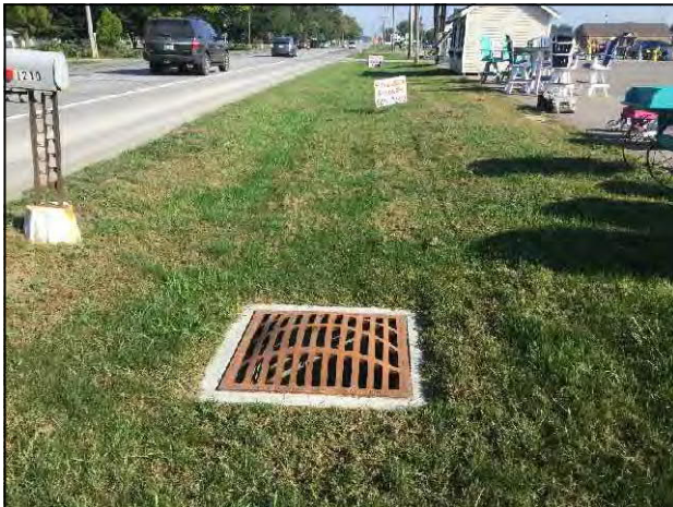
3. View of culvert and SR 5 Right-of-Way (ROW) on the east side of SR 5, looking north within project area.
