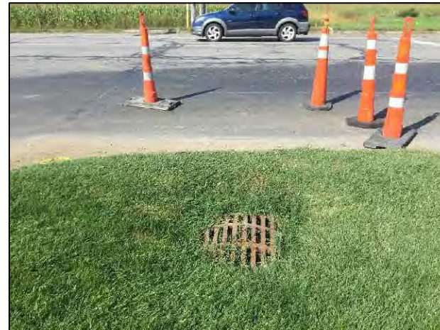
16. View of culvert and SR 5 ROW on the east side of SR 5, looking west within project area.
