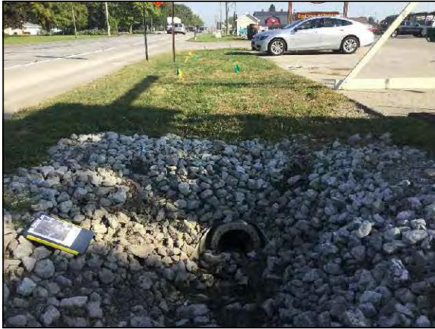
1. View of culvert located within the project area, on the east side of SR 5, looking north.
