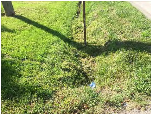
11. View of culvert on the east side of SR 5, looking south within project area.
