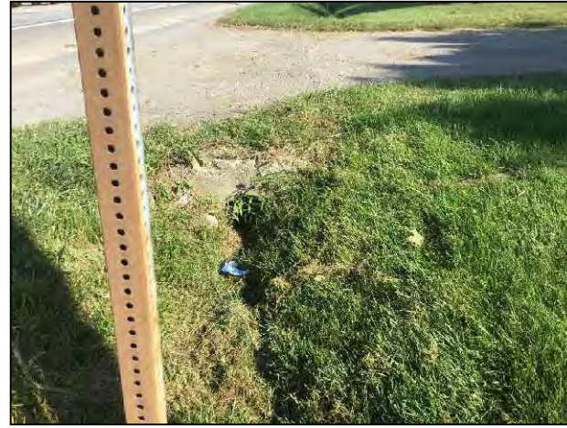
10. View of culvert on the west side of SR 5, looking south within project area.
