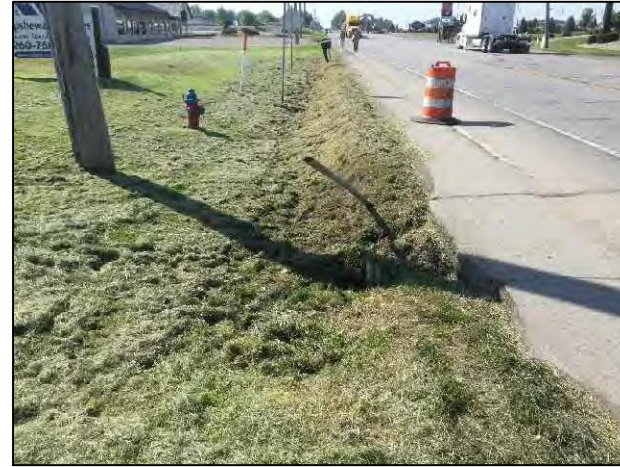
14. View of culvert on the east side of SR 5, looking south within project area.
