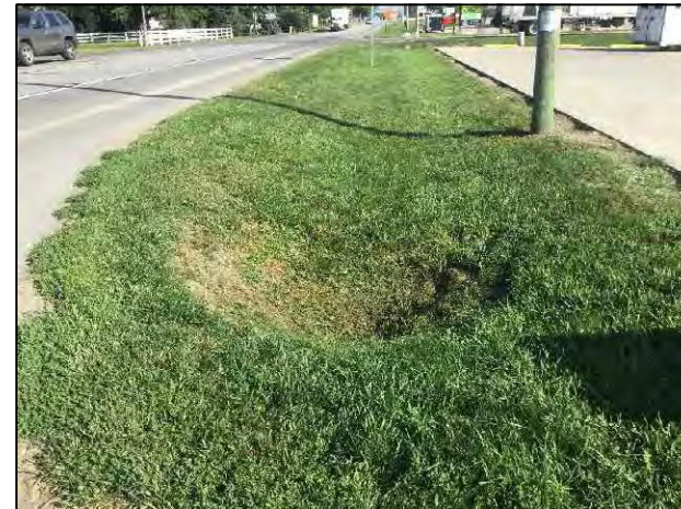
4. View of culvert on the west side of SR, looking north within project area.
