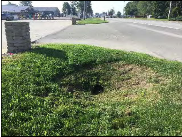
5. View of culvert on the east side of SR, looking south within the project area.
