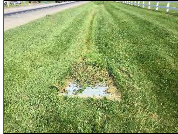
18. View of culvert on the west side of SR 5, looking north. within project area.
