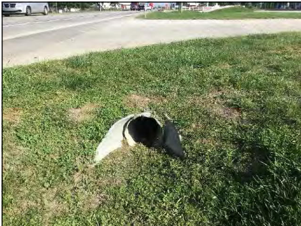
7. View of culvert on the east side of SR 5, looking north within project area.
