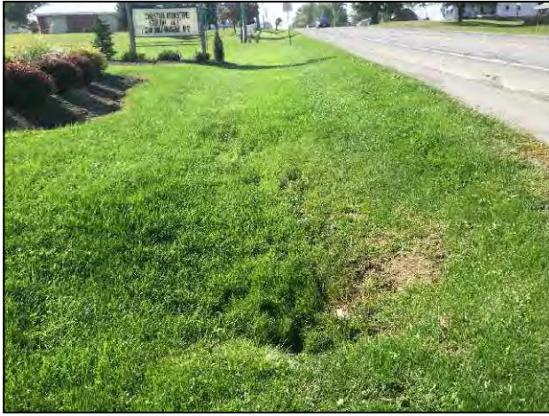
9. View of culvert on the east side of SR 5, looking north within project area.
