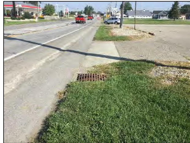
12. View of culvert and SR 5 ROW on the west side of SR 5, looking north within project area.
