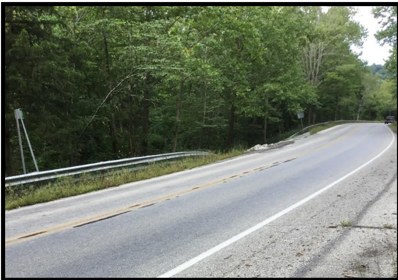
Guardrail bending and disappearing downslope on SR 1 Franklin County, Indiana
