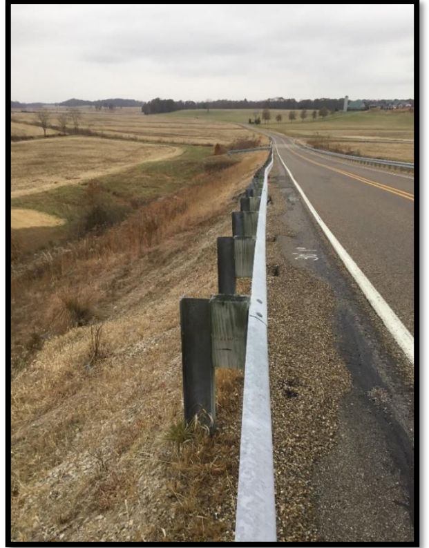
Guardrail bending on SR 245 Spencer County, Indiana
