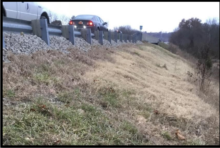
Drop in guardrail on SR 66 Vanderburgh County, Indiana
