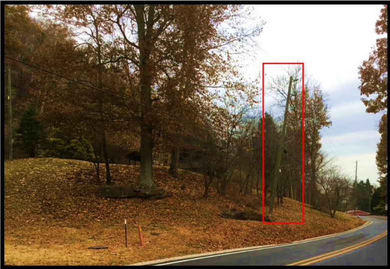
Pole leaning near SR 66 Perry County, Indiana
