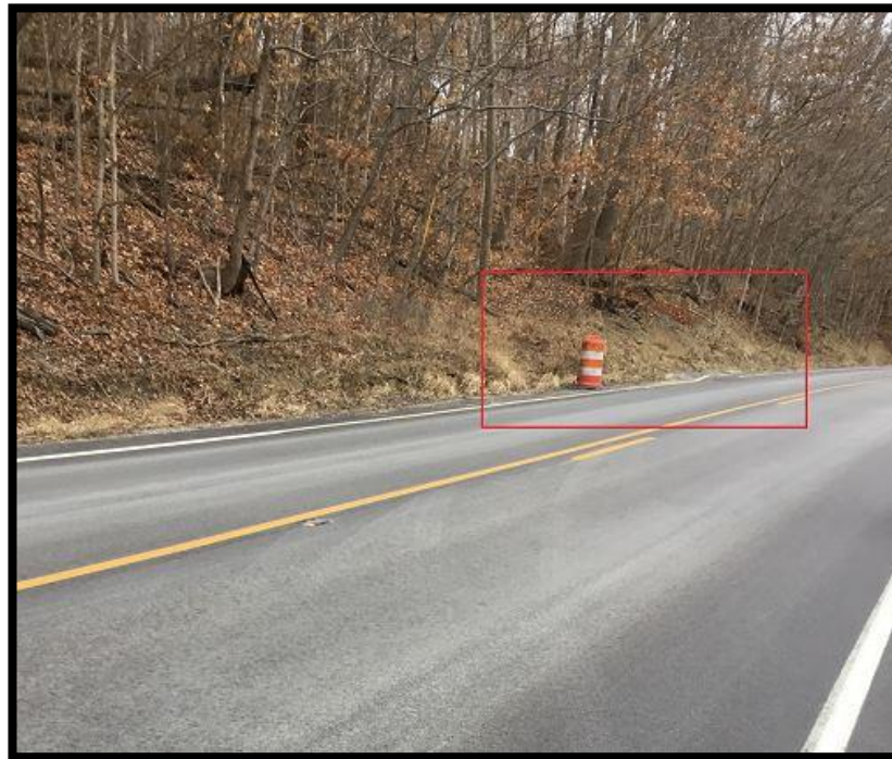
Photo: Uplift in pavement on SR 66 Spencer County, Indiana
