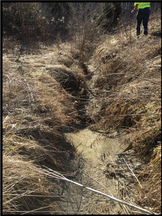
Broken paved ditch near SR 350, Ripley County Indiana
