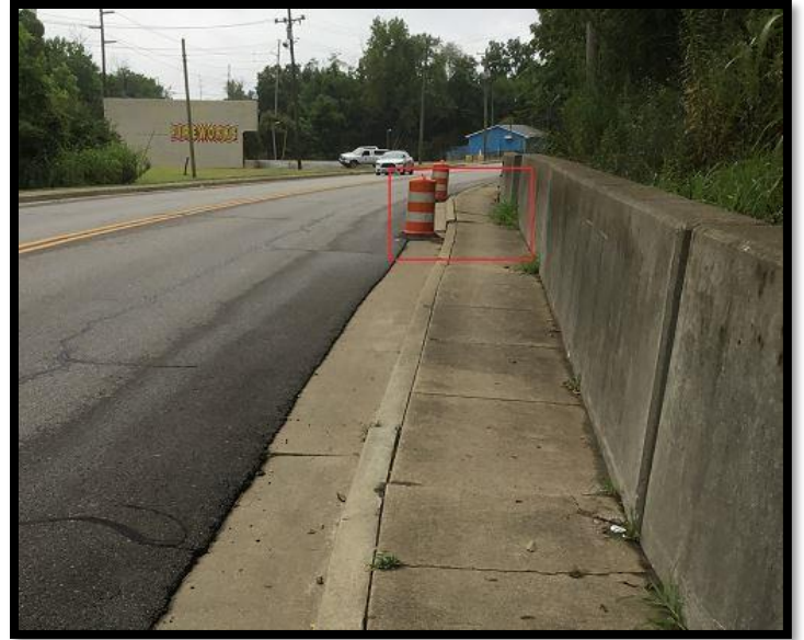
Photo: Uplift in sidewalk on SR 111, Floyd County, Indiana
