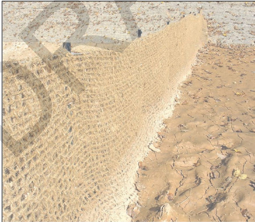
Exhibit 708.06-E. Close-up of a porous baffles made of 700 g/m 2 coir erosion control blanket. Notice the coir blanket has been anchored to the basin floor with blanket staples.
